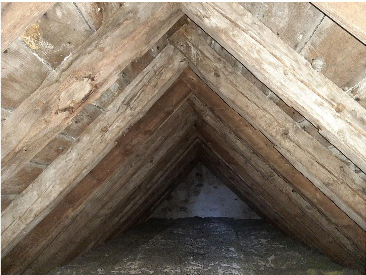
Interior of roof structure, looking north; note to right in situ pegs within relict collar joints
