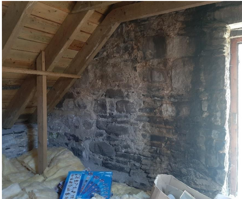
Interior of the north gable of the kitchen extension – detail of masonry construction
