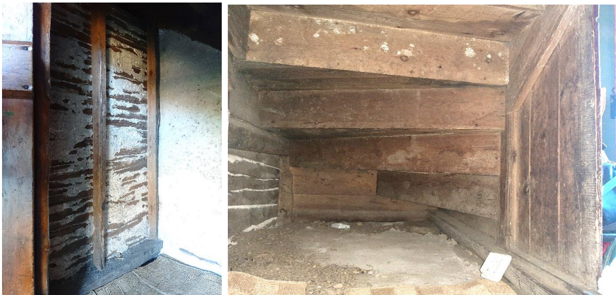
Under-stair area : left – rear wall of box-bed to south; right – stair construction
