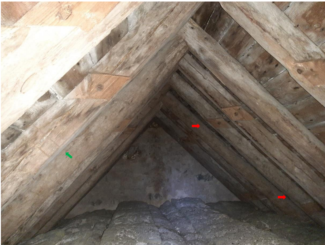
Roof interior looking south; upper faces of many rafters display relict upper and lower collar lap-joints (red arrows); some timbers display assembly marks (green arrow)
