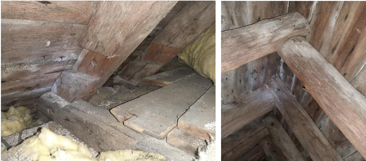
Left : roof - detail showing relict collar-beam lap-joints with peg-holes, and the existing collar below, similarly jointed but affixed with an iron spike.
