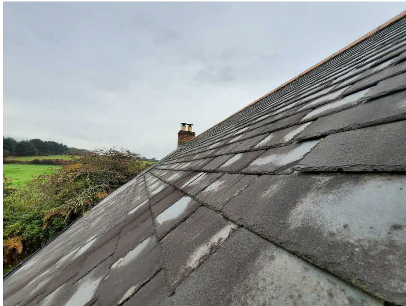
Figure 5: View south from within the first-floor room (vaulted with no roof space) of part of the east pitched roof at 'The Mowhay'.
