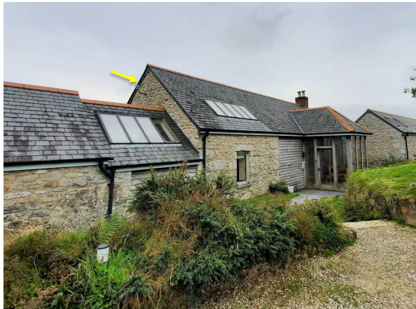
Figure 2: View of the northern and western elevations of the wider building at 'The Mowhay'; the yellow arrow indicates the approximate location of the proposals on the eastern pitch.
