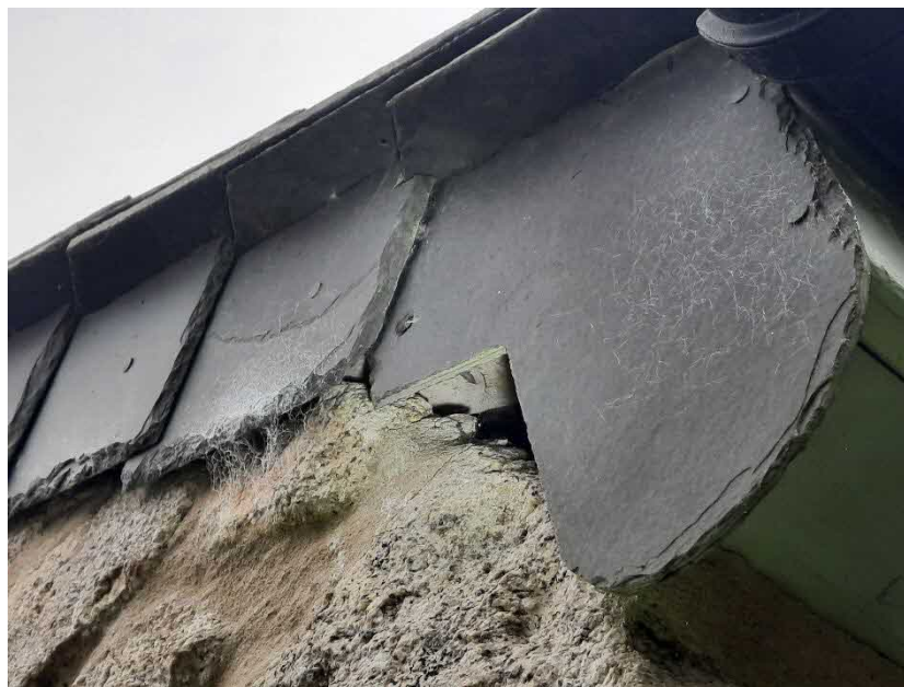
Figure 6: View of a small gap beneath the hanging slate tile and the wall top on the north-western corner of the building at 'The Mowhay, located on the opposite side of the property from where new dormer windows are proposed'.
