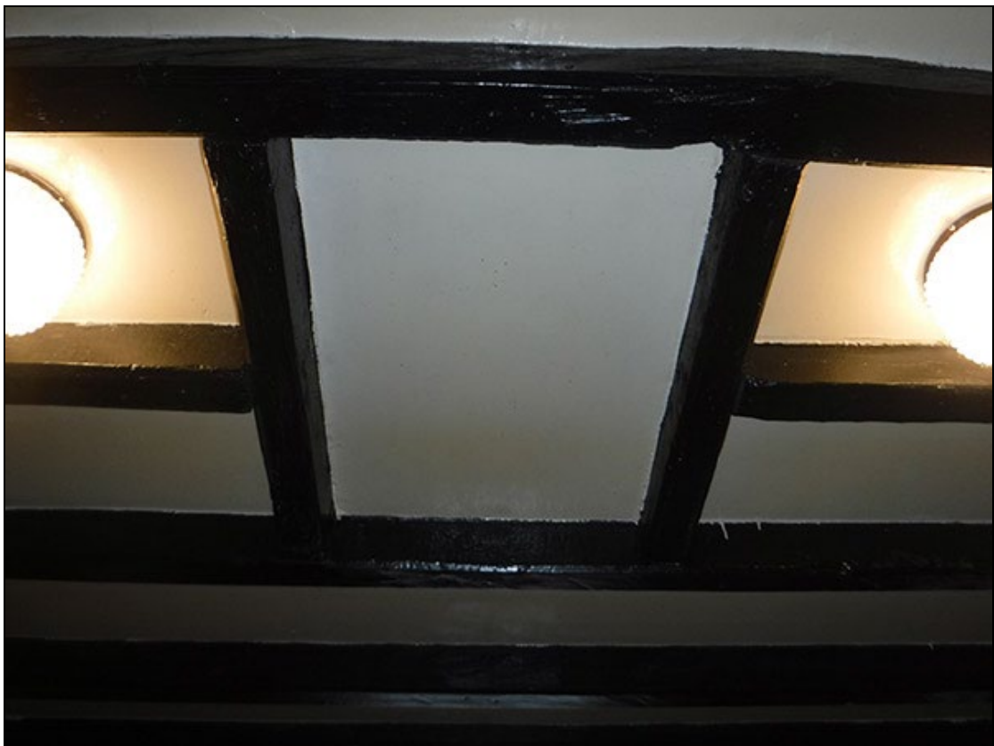
Figure 22 The location for a possible hatch in the ceiling of the first floor
