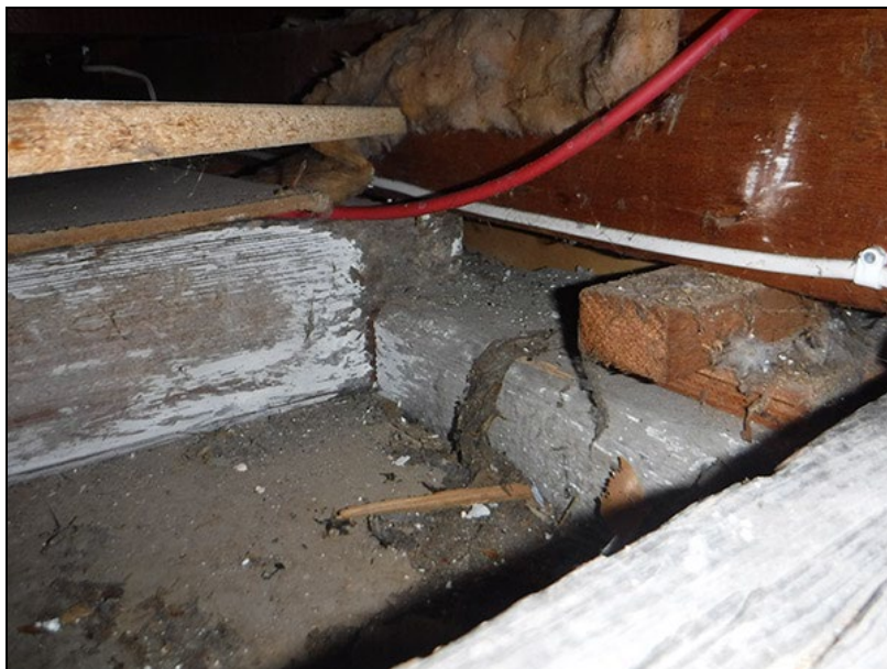
Figure 13 The top of a floor joist in the top floor showing its upper projection resting on a transverse beam
