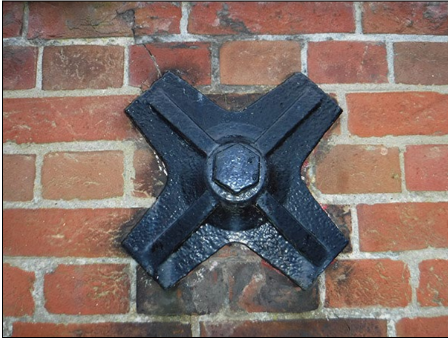
Figure 30 Details of one of the large cruciform washers on the exterior brickwork
