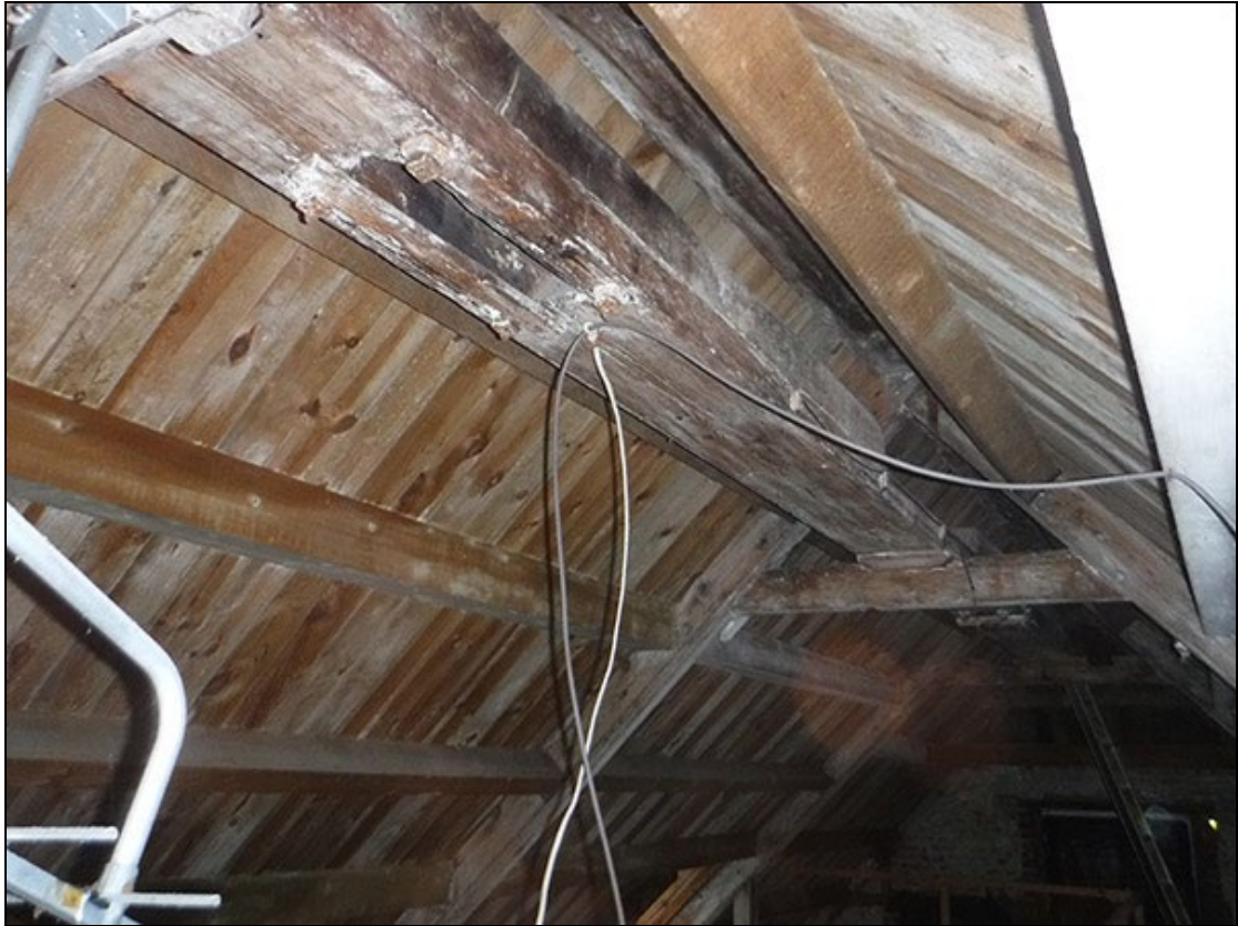
Figure 21 The remains of the hoist timber in the roof-space of the upper floor, looking north
