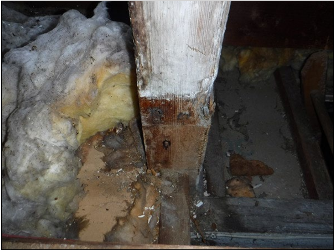
Figure 23 The evidence for a low-level retaining board in the fourth floor on one of the posts, with a coat of whitewash respecting their position
