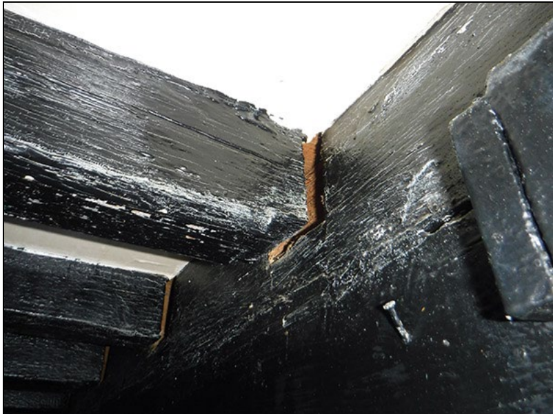
Figure 12 A floor joist on the first floor projecting out of its housing in a transvers beam
