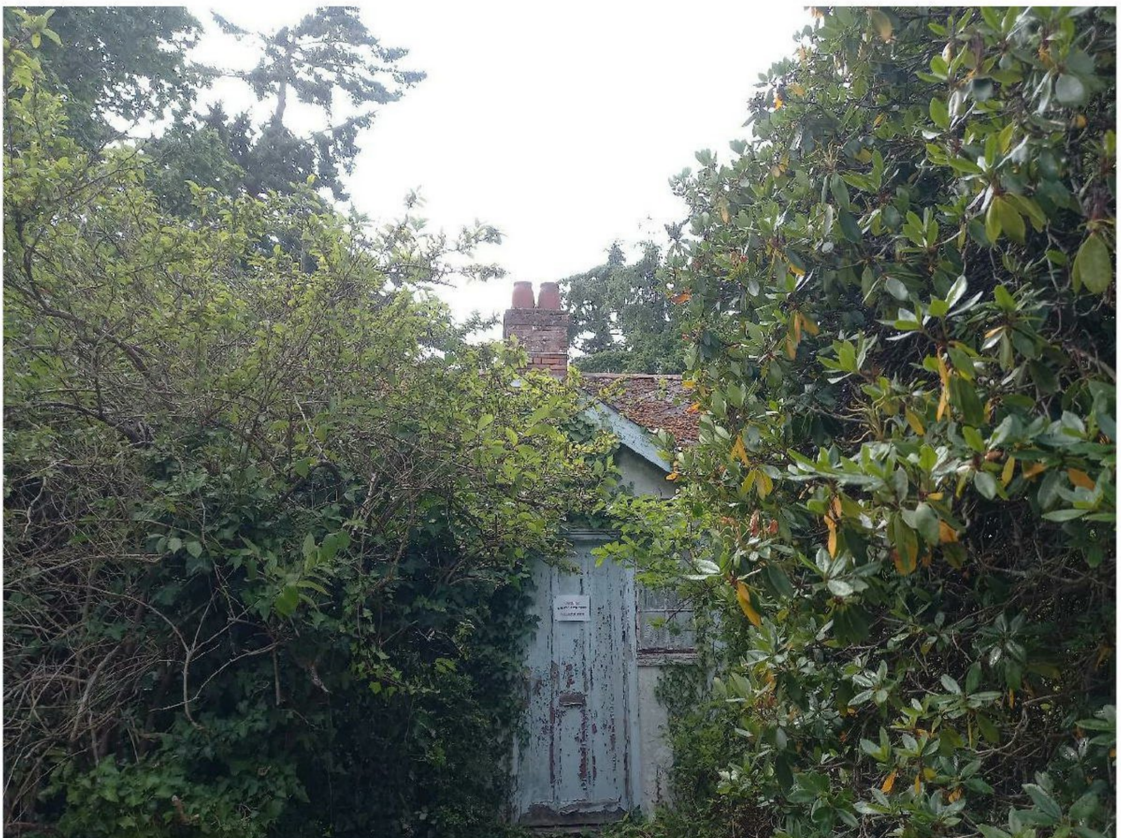
Plate 14 – Southern aspect of building 4, showing heavy overgrowth by vegetation.
