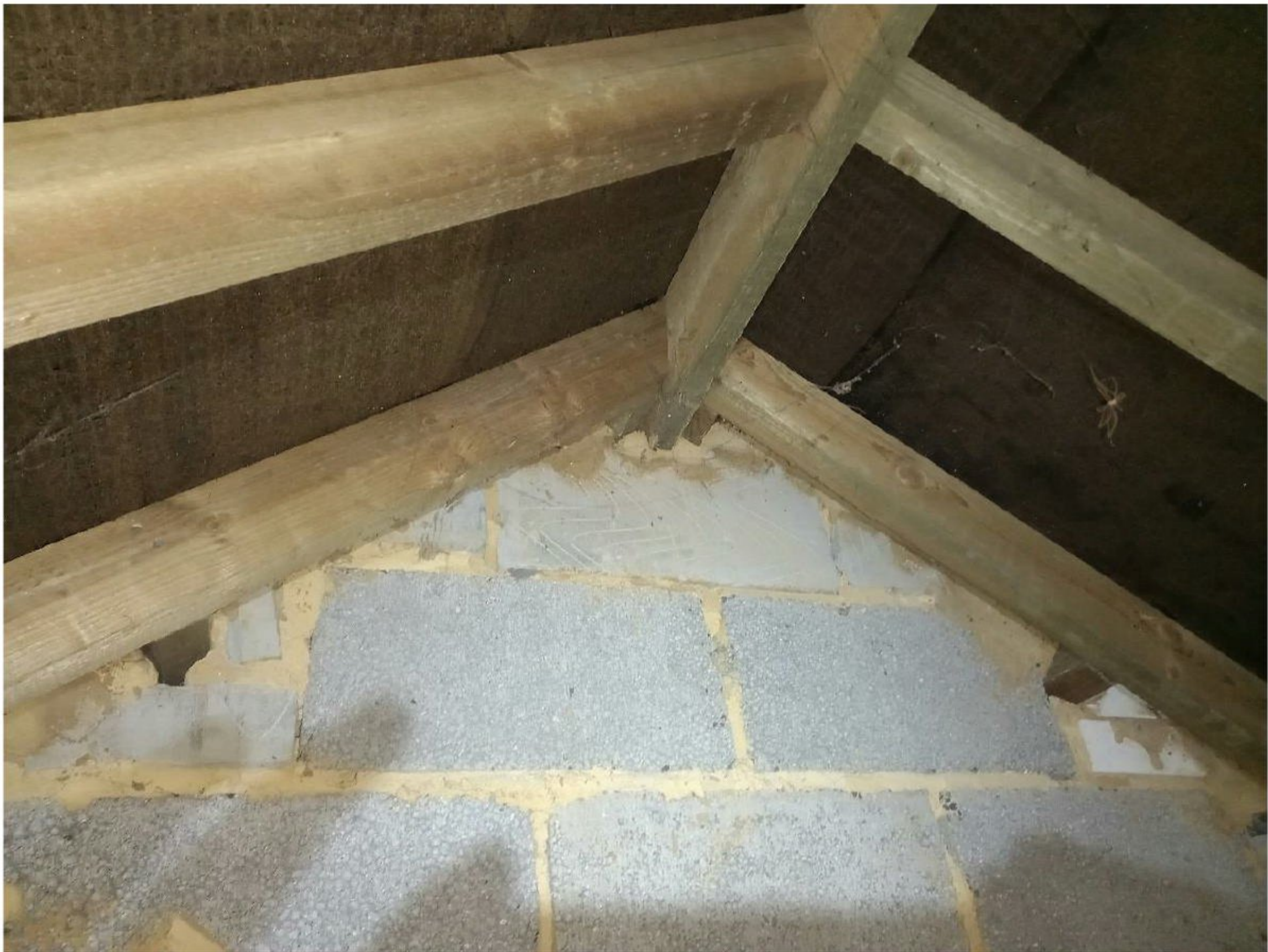
Plate 3 – Photograph showing gaps in the gable end of the loft void.
