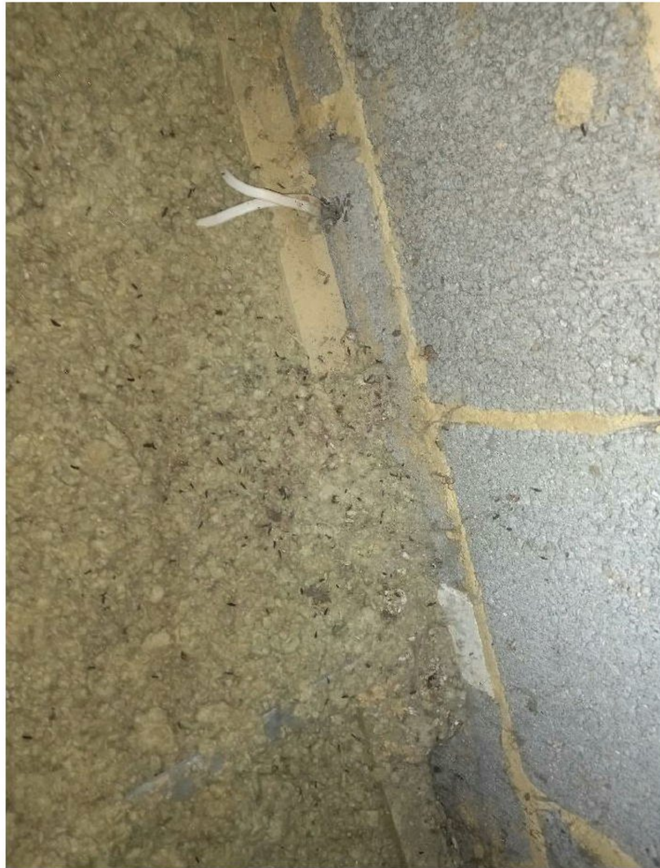
Plate 1 – Bat droppings discovered in the loft void of building 1.
