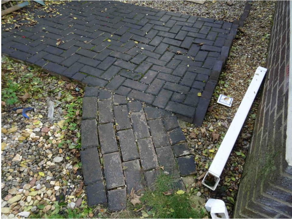
3. Displaced block paving
