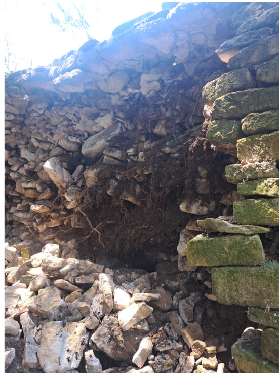
Pic 2 – shows tree roots in the wall
