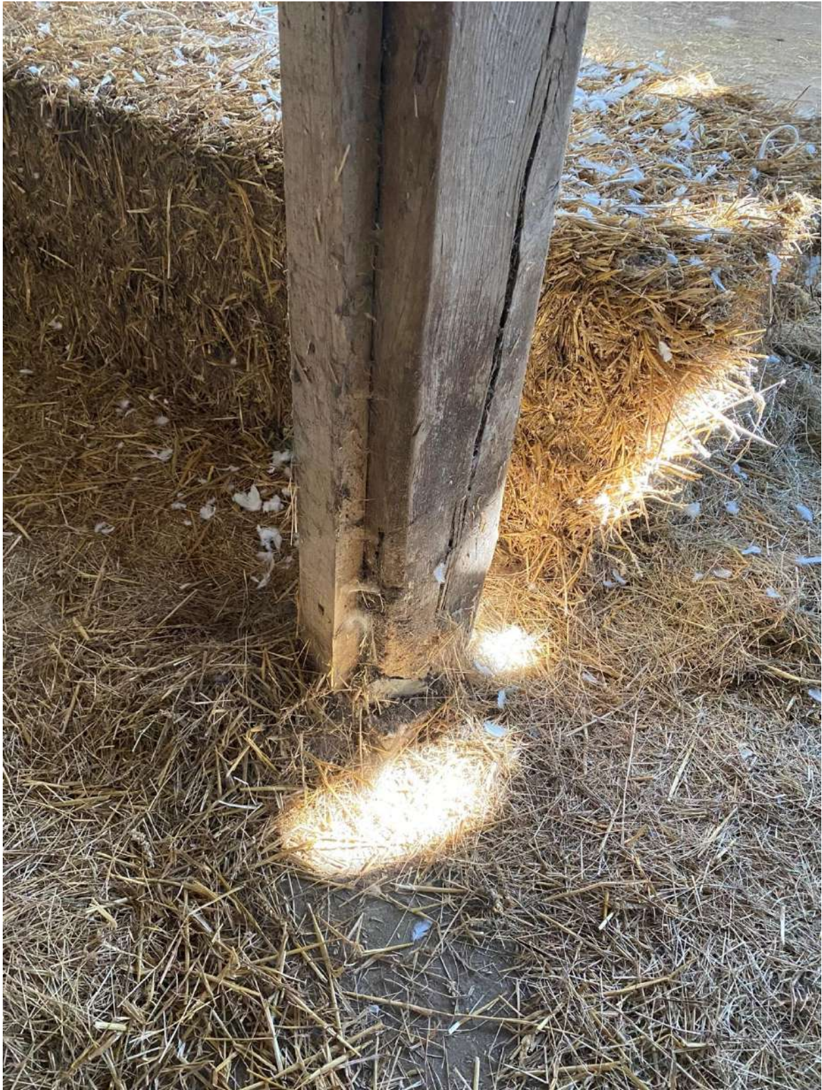
Figure 9 - Previous Repair of Column
