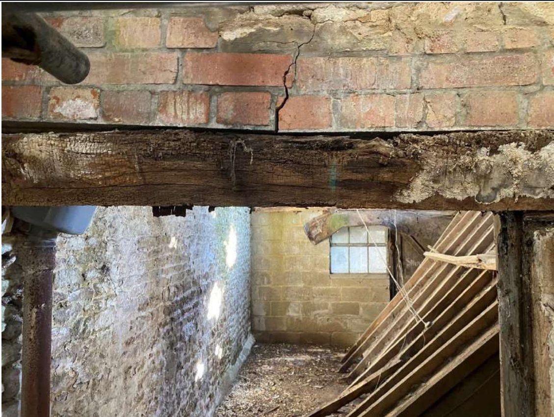
Figure 12 - Lintel Failure in Left Hand Wall
