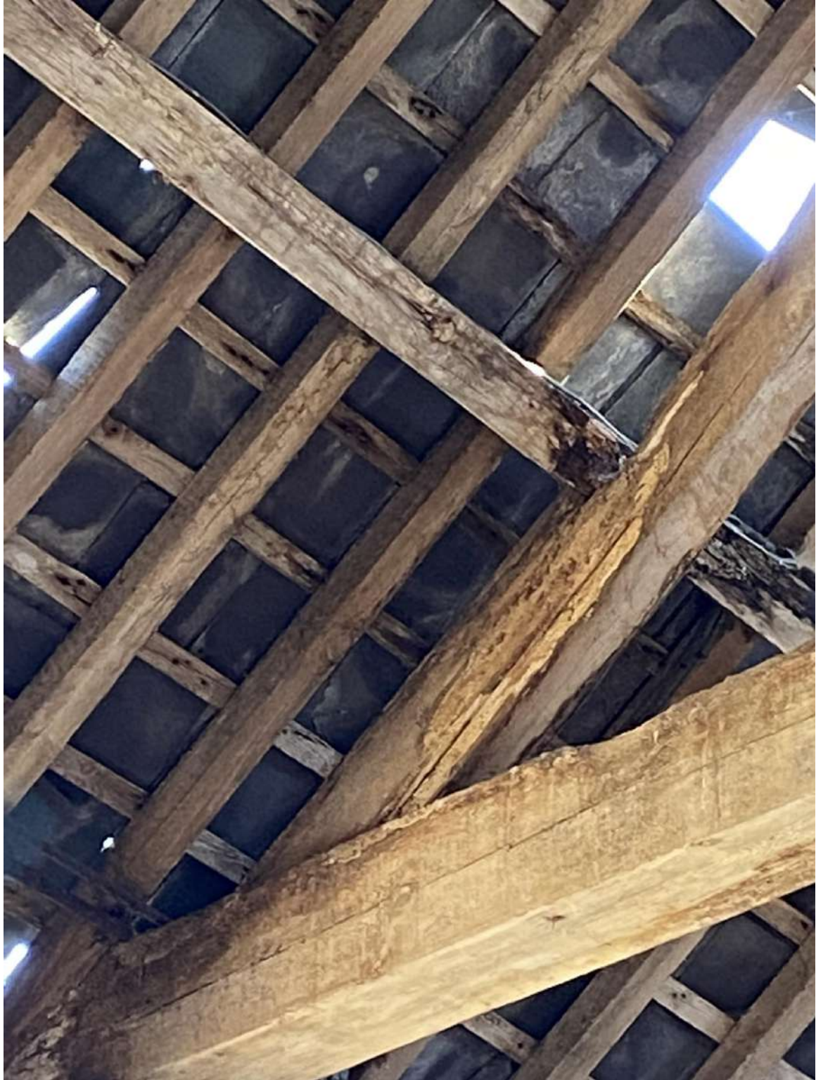
Figure 6 - Fungal Attack and Decay of the Supporting Timber
