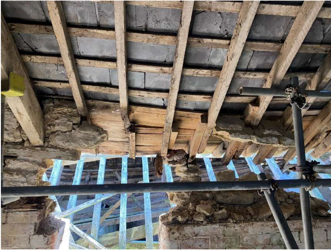
Figure 10 - Loss of Masonry At Valley Between Stonemasons Courtyard and the Covered Yard
