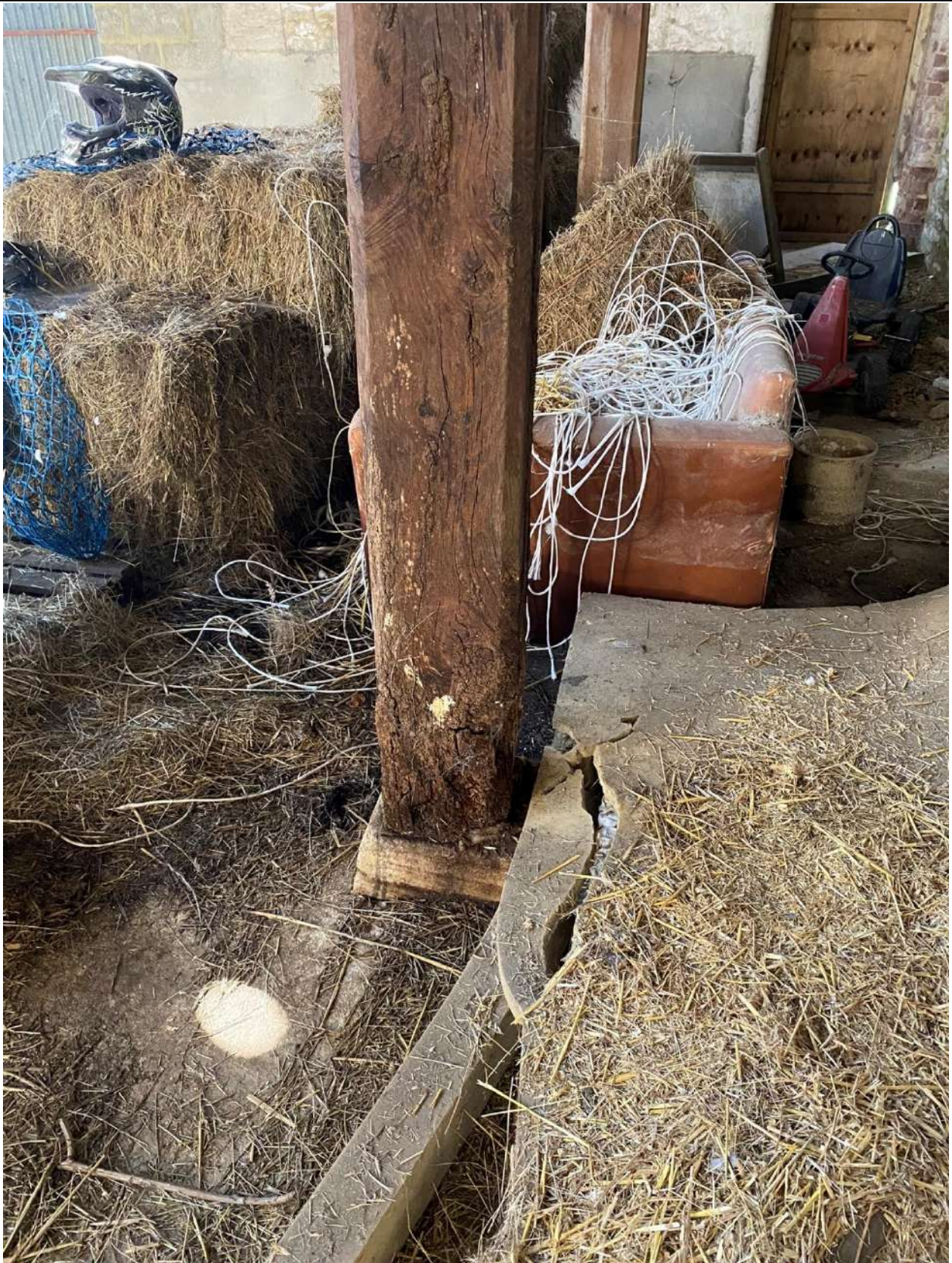
Figure 8 - Decay of Column at Base
