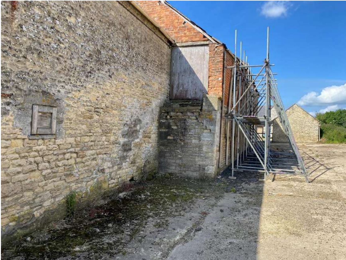
Figure 15 - Outward Movement of First Floor Wall and Installation of Scaffold Shoring
