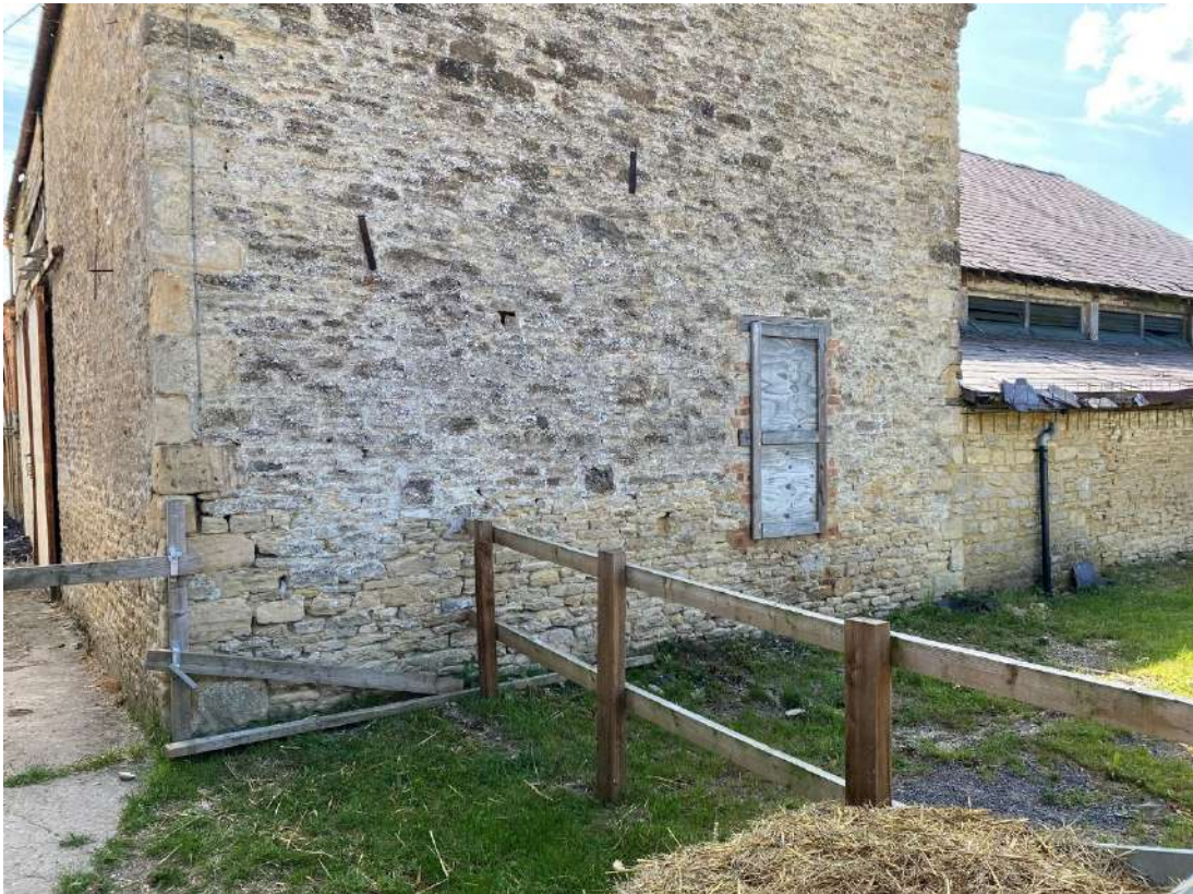
Figure 16 - Loss of Pointing Along Western Gable
