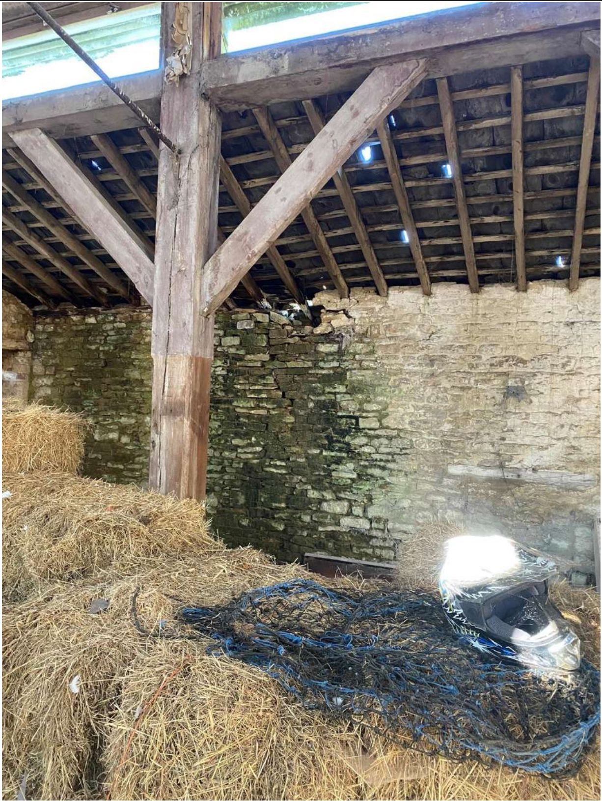
Figure 13 - Damage to Southwestern Corner of the Covered Yard
