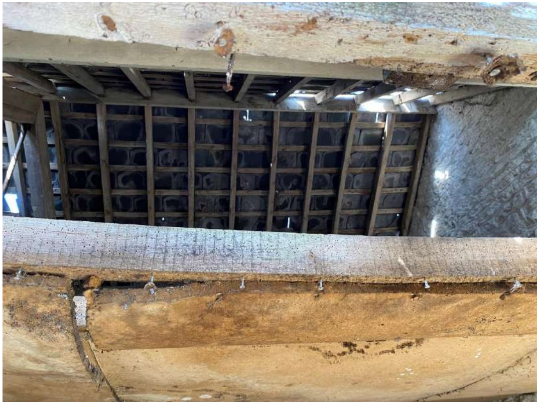
Figure 10 - Insect Attack of Floor Joists
