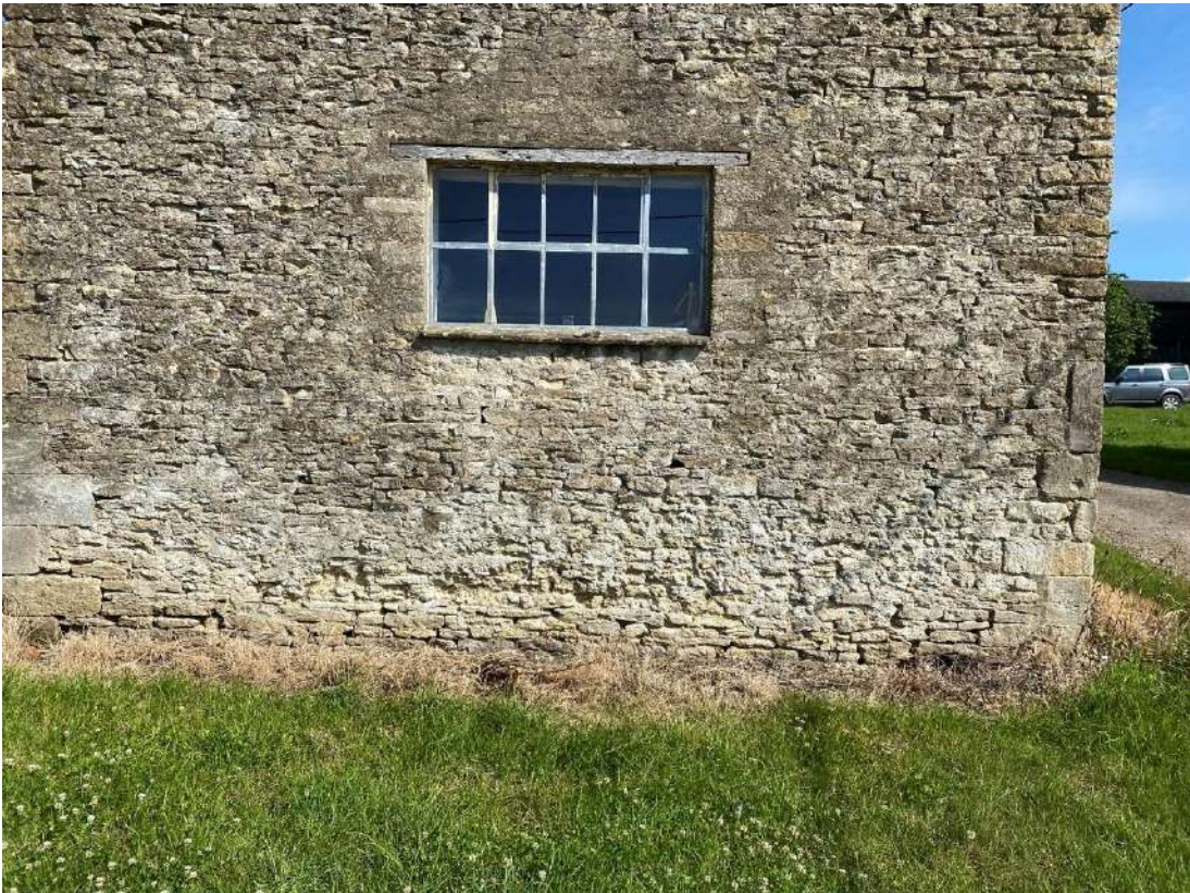
Figure 13 - Loss of Pointing at Ground Level
