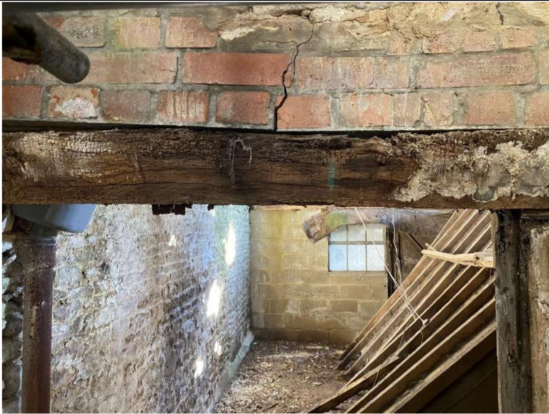
Figure 9 - Failure of Joist Bearings Onto Wall
