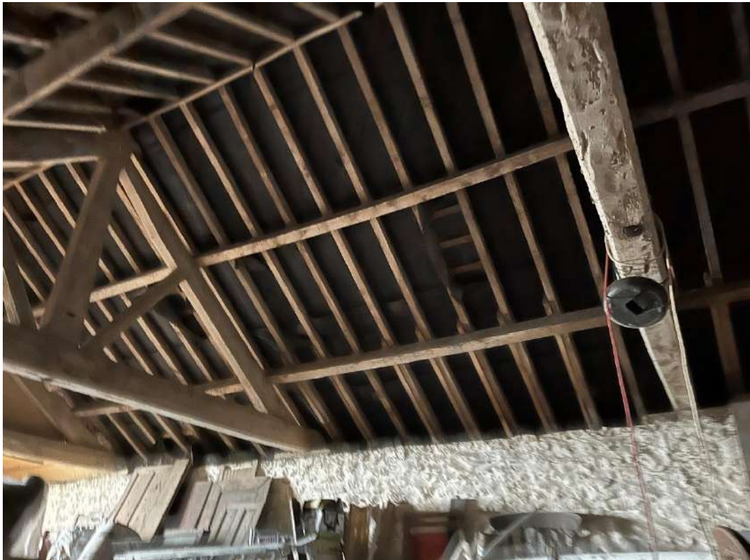
Figure 6 - Minor Damage to Roofing Felt of the Workshop Roof
