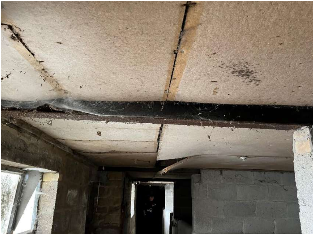
Figure 8 - Moisture Damage To Ceiling of Northern Block
