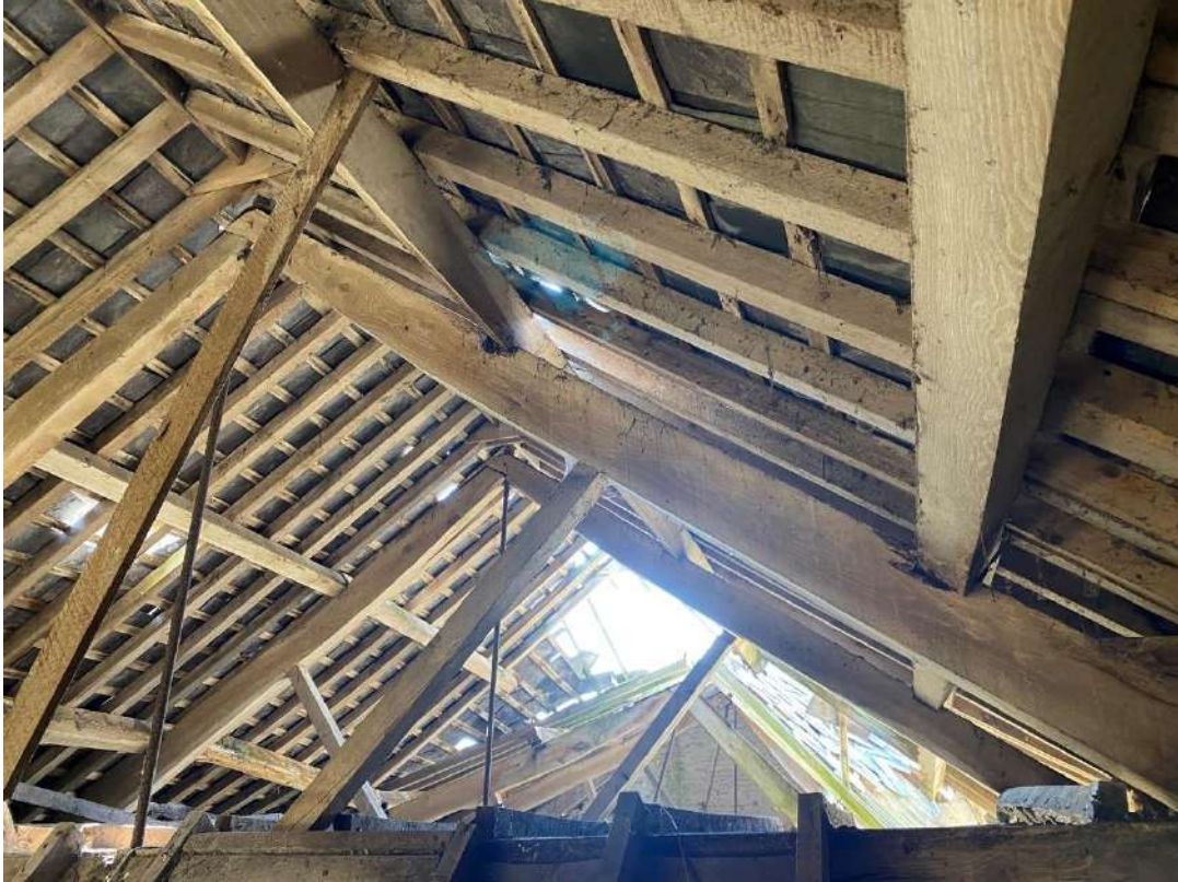
Figure 1 - Hole in Roof With Collapsed Roof Beneath
