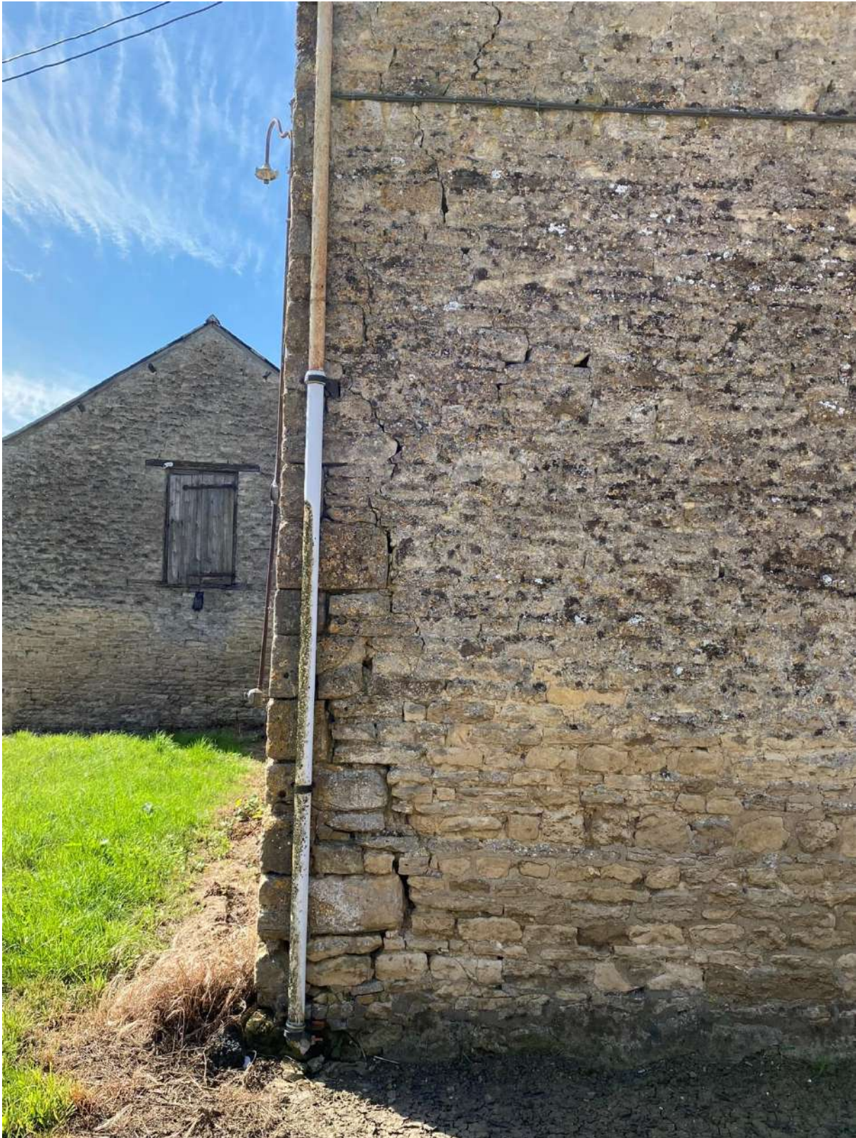
Figure 11 - Cracking at Interface of Stone and Quoins
