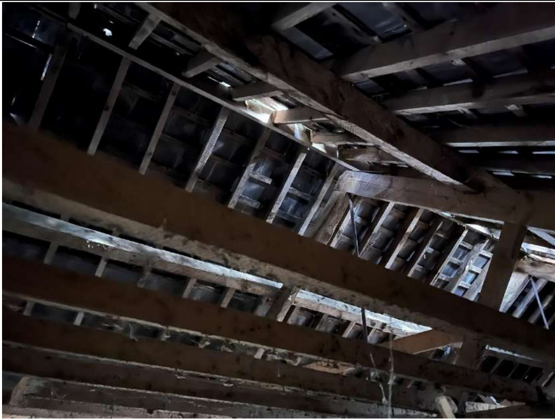
Figure 7 - Daylight Visible Through Roof of Southern Stable Block
