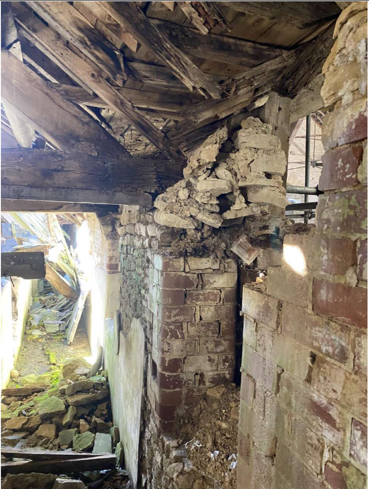
Figure 3 - Failure of Timber Lintel Supporting Masonry, Decay of Truss at Bearing and Broken, Unsupported Rafters
