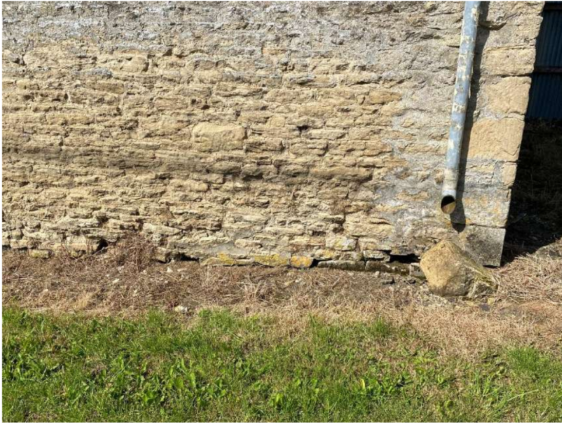
Figure 12 - Damage to Masonry Owing to Discharge of Surface Water to Ground
