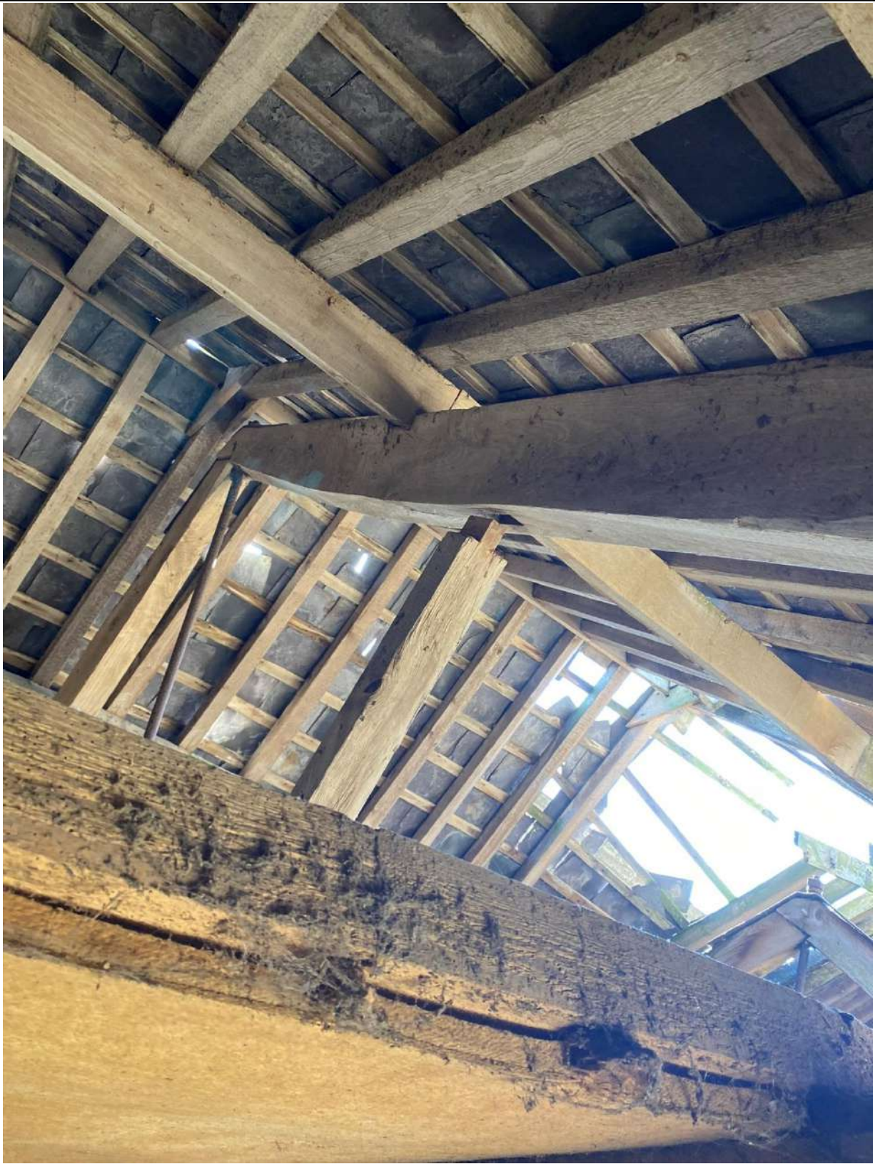
Figure 4 - Local Failure of Joint Between Rafter and Strut
