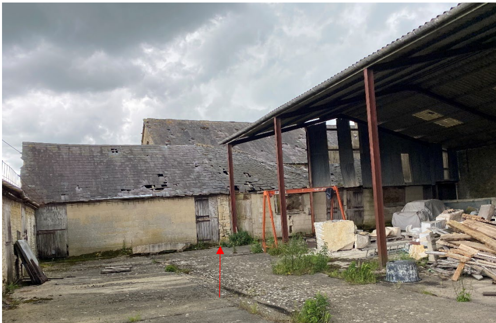
Figure 28: Looking across eastern yard towards Barn 3 with later blockwork walling, stone pier (arrowed) marks end of older structure, possibly open sided, the roof is partially collapsed but a consistent structure spanning older and later portions.
