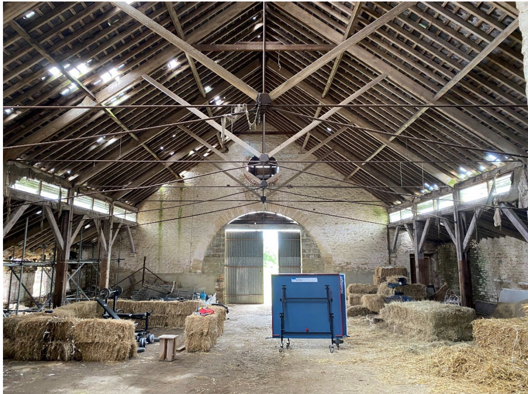
Figure 31: interior of covered yard looking south with steel tension trusses, the clerestory and posts supporting the peripheral 'aisles'.
