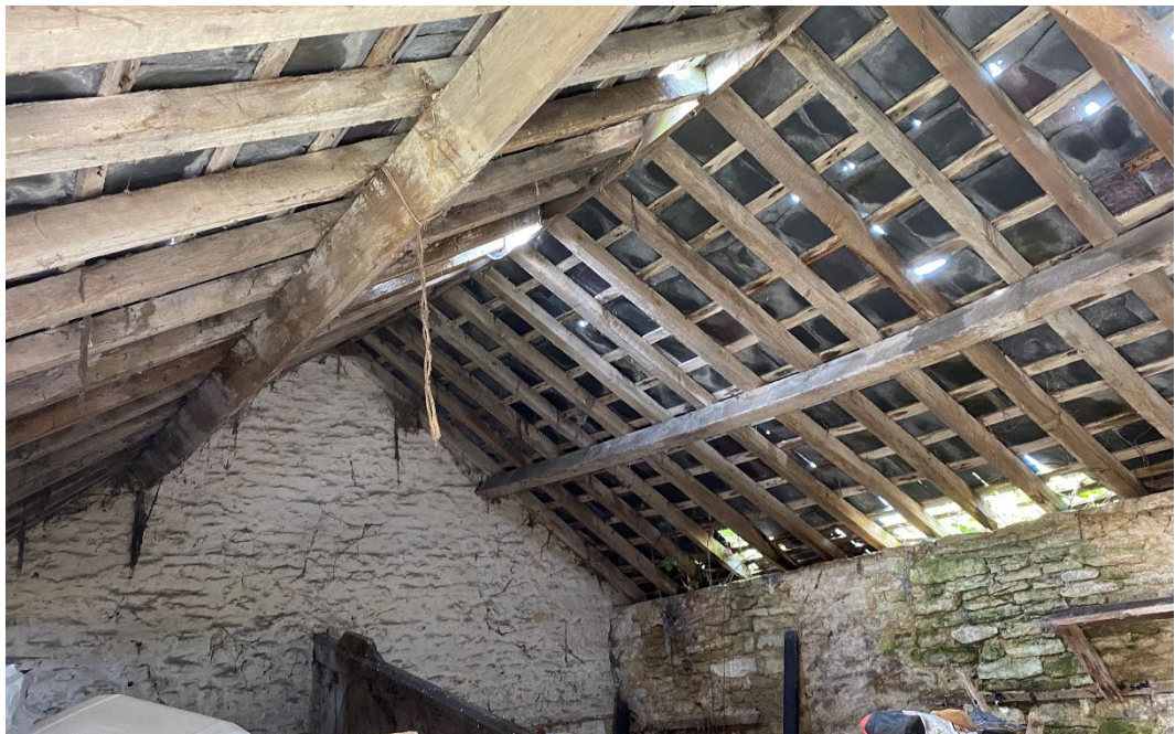
Figure 14: internal view of one of the stables at the western end the roof has been renewed here.
