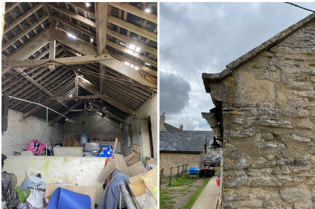
Figure 16-17: (left) interior of the western range of Barn 1; (right) view of the stone kneeler at the end of the northern stable, a matched detail to one of the two threshing barns making up building 2.
