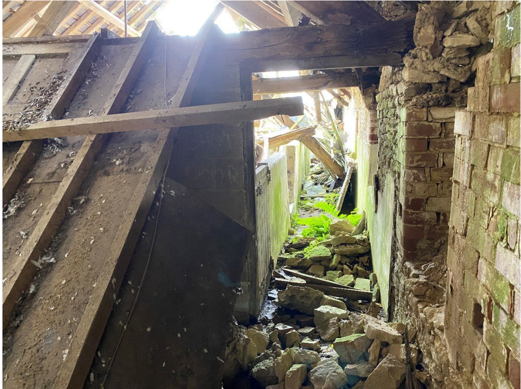
Figure 29: Partial inspection of the feeding passage within Building 3, the wall with openings on the right is to Building 4, the cement rendered stall partitions are visible in the centre of the picture, a blockwork partition visible to the left of the doorway.
