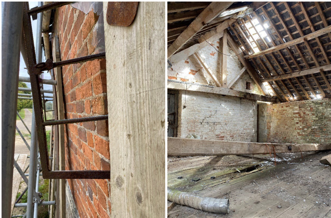
Figure 26-27: Metal framed window in linking structure, note lean on red brick wall (image view point constrained by scaffold access) and, (right) interior of the linking structure with central truss collapsed on the floor and no longer supporting the roof.
