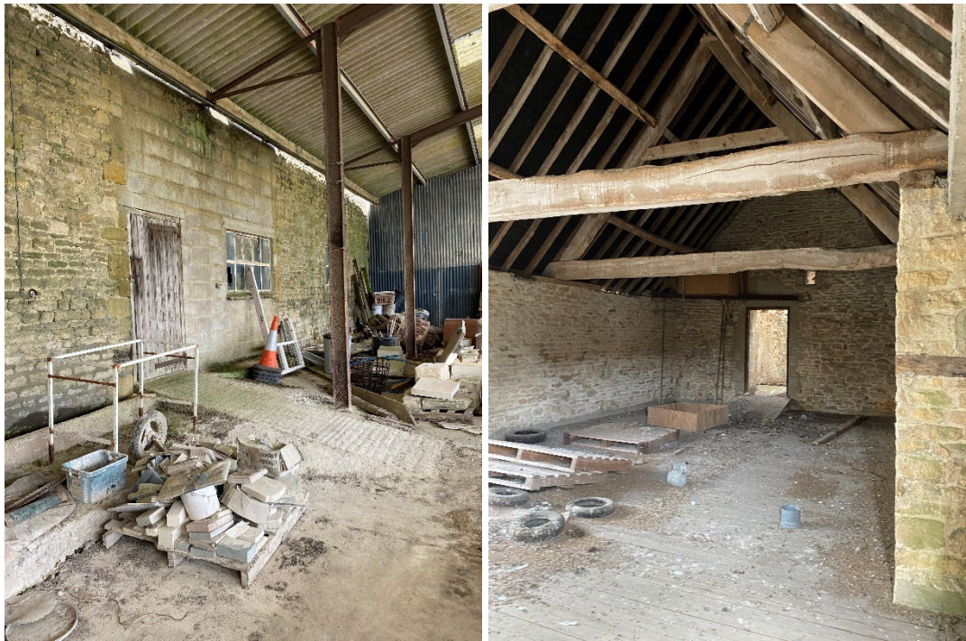
Figures 19-20: the blocked threshing door and one of the windows inserted in the southern elevation of Barn 2B with internal view of the open first floor area and link through to the intermediate structure.
