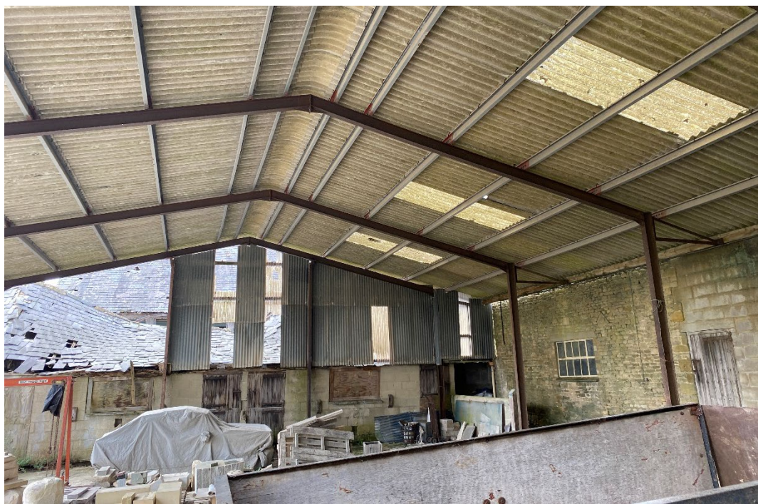
Figure 32: Interior of Building 5 covering the former yard between Barn 2B on the right and the collapse Building 3 in the centre and left.
