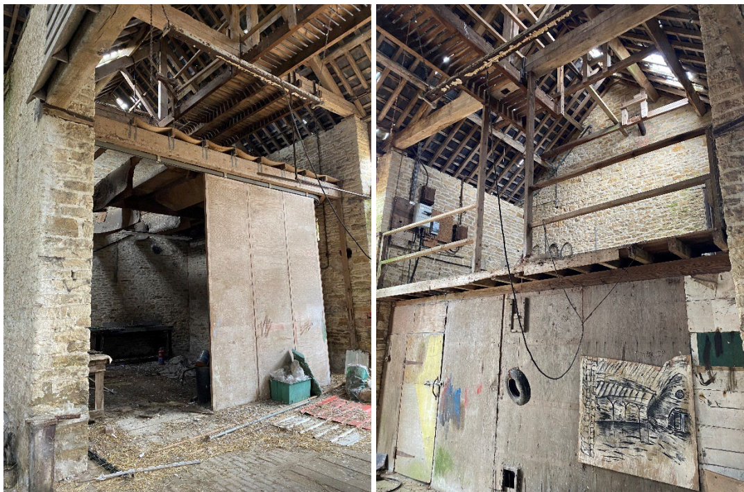
Figures 22-23: (left) internal view within western part of Barn 2 and (right) the eastern side of the barn showing substantial king post trusses and floor structures in the end bays flanking the threshing doors.
