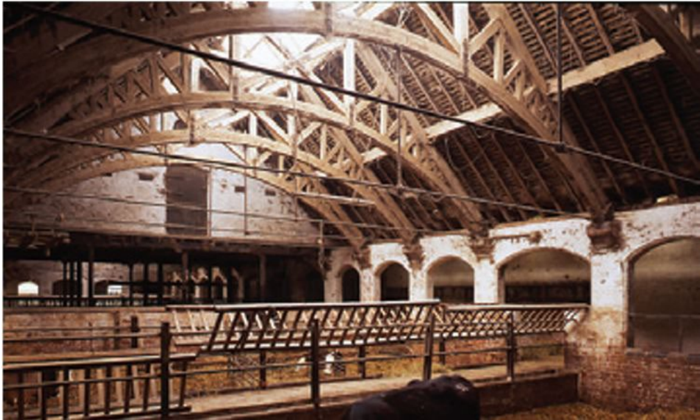
Figure 44: An example of a listed covered yard, Grade II* listed covered yard, mid-19 th century Apley Park, Shropshire (Historic England © Mike Williams) included in Historic England's summary of National Farm Building Types, 2013
