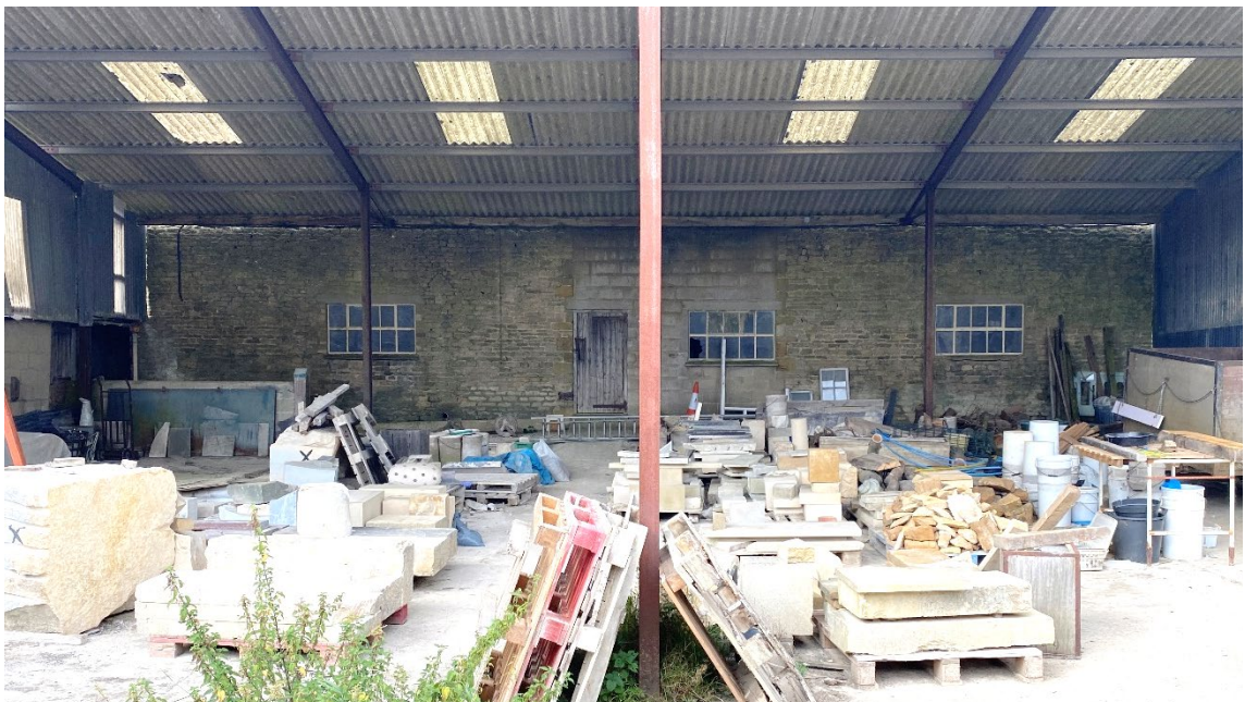
Figure 50: view to the southern façade of the eastern threshing barn which will be re-exposed with the removal of Building 5 and re-opening of the former threshing door opening.
