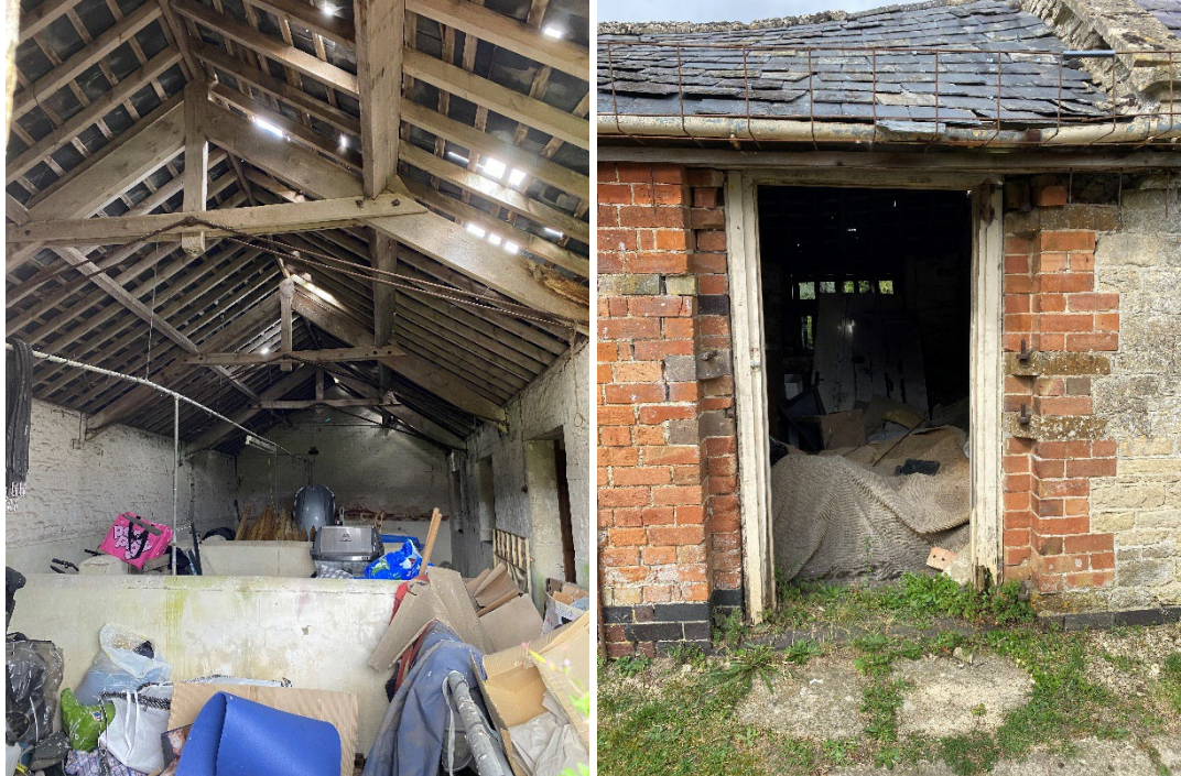
Figure 45-46: Open roof space and trusses to remain within building 1B and (right) typical red brick doorway features, including stone detailing for pintle hinges to remain with building 1A, elevated stone coping to gables also to be retained and restored.
