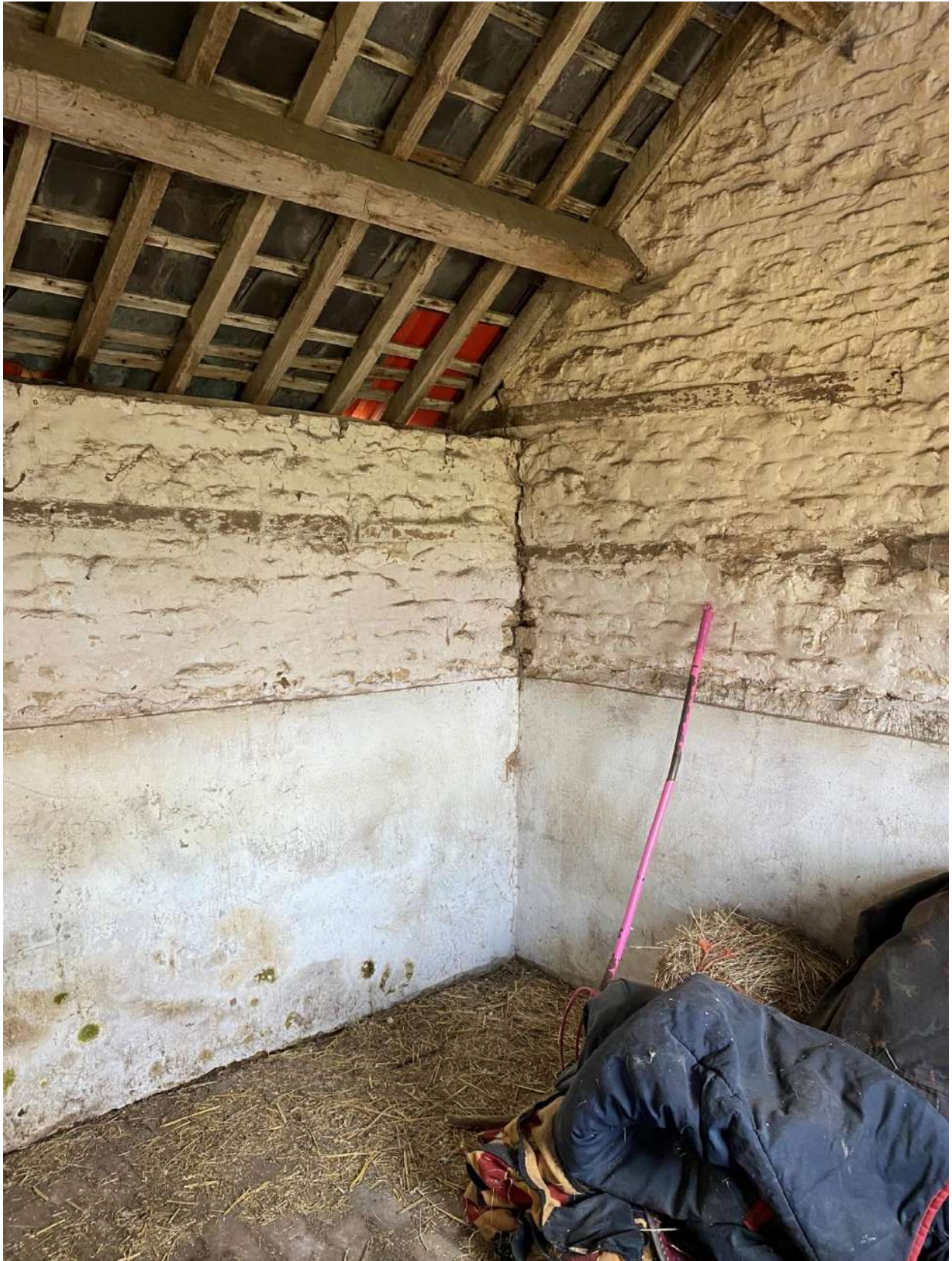
Figure 8 - Separation of Gable Wall From Rear Wall
