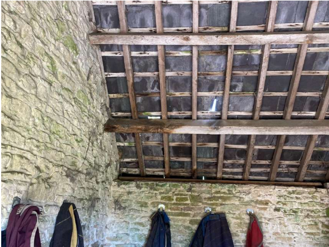
Figure 7 - Moisture Penetration Through Roof and Possible Decay of Purlin
