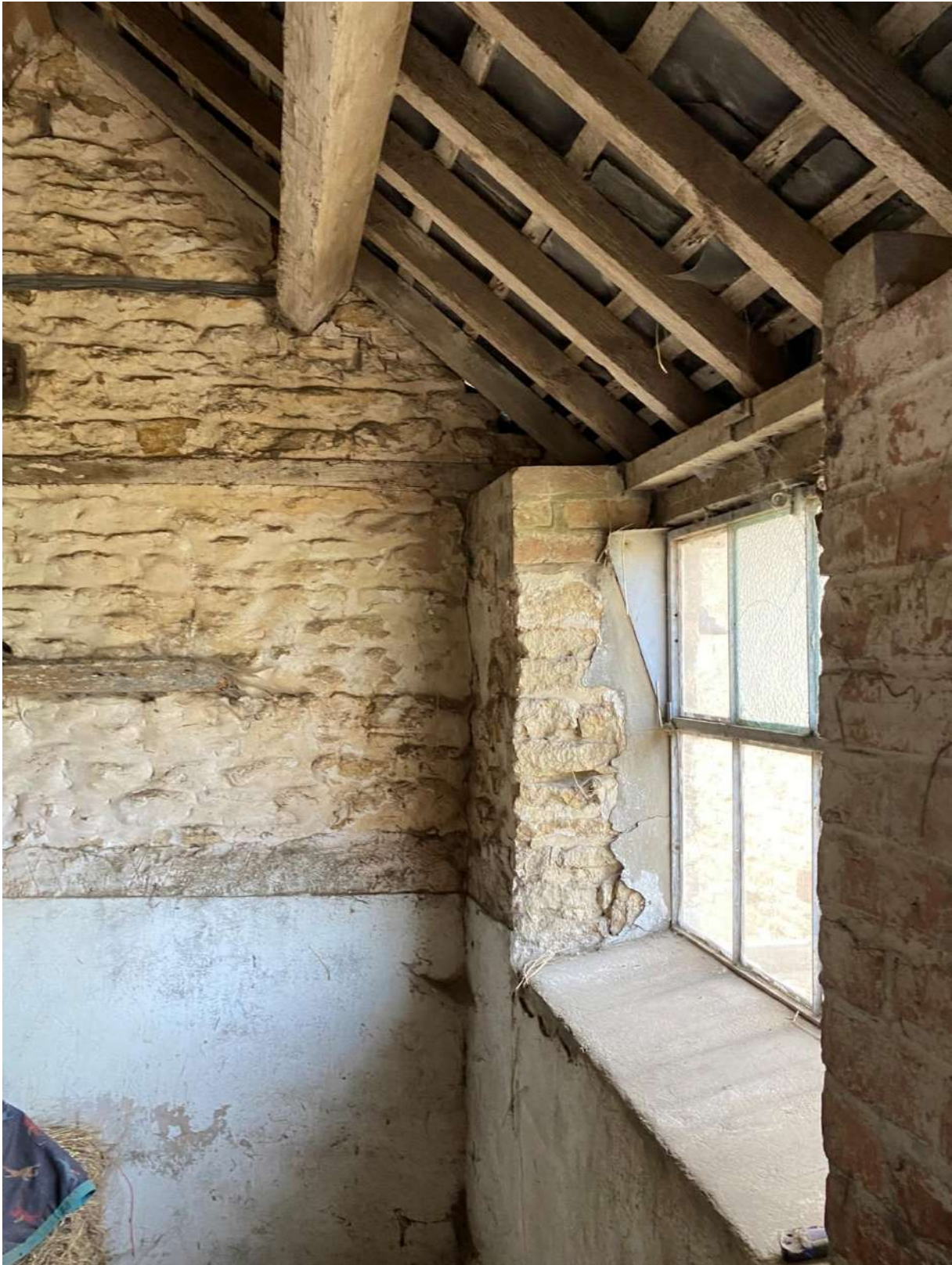
Figure 9 - Separation of Gable Wall From Wall
