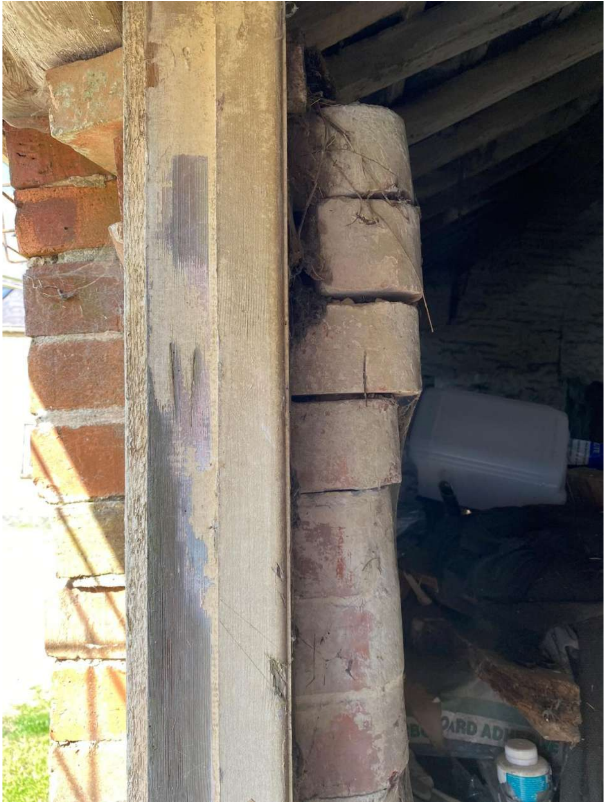
Figure 5 Damage to Masonry At Bearing of Lintel Above Entrance Door
