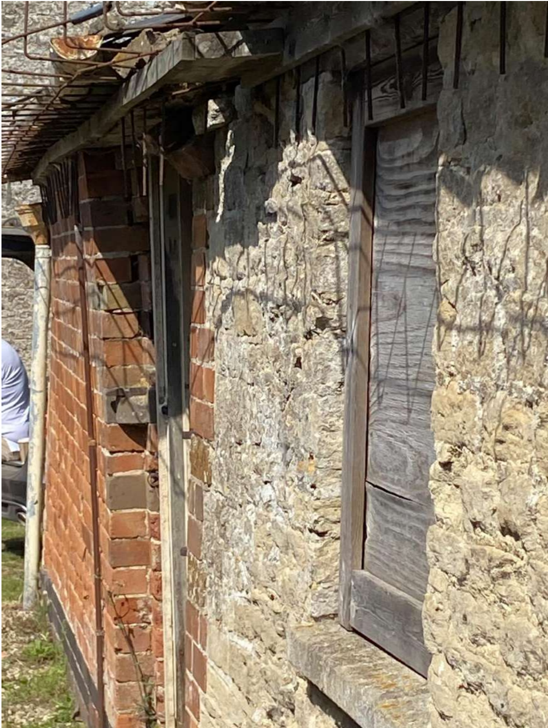
Figure 6 - Outward Movement of Brick Wall
