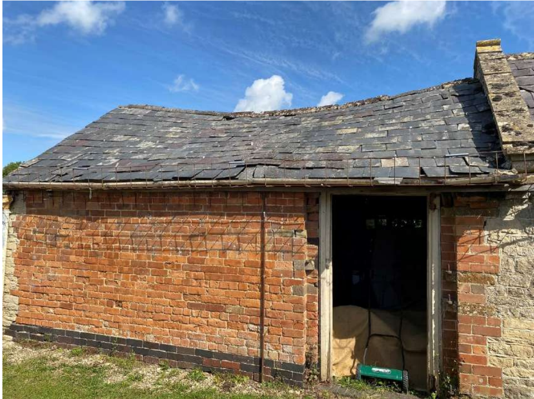
Figure 3 - Excessive Deflection of Storeroom Roof
