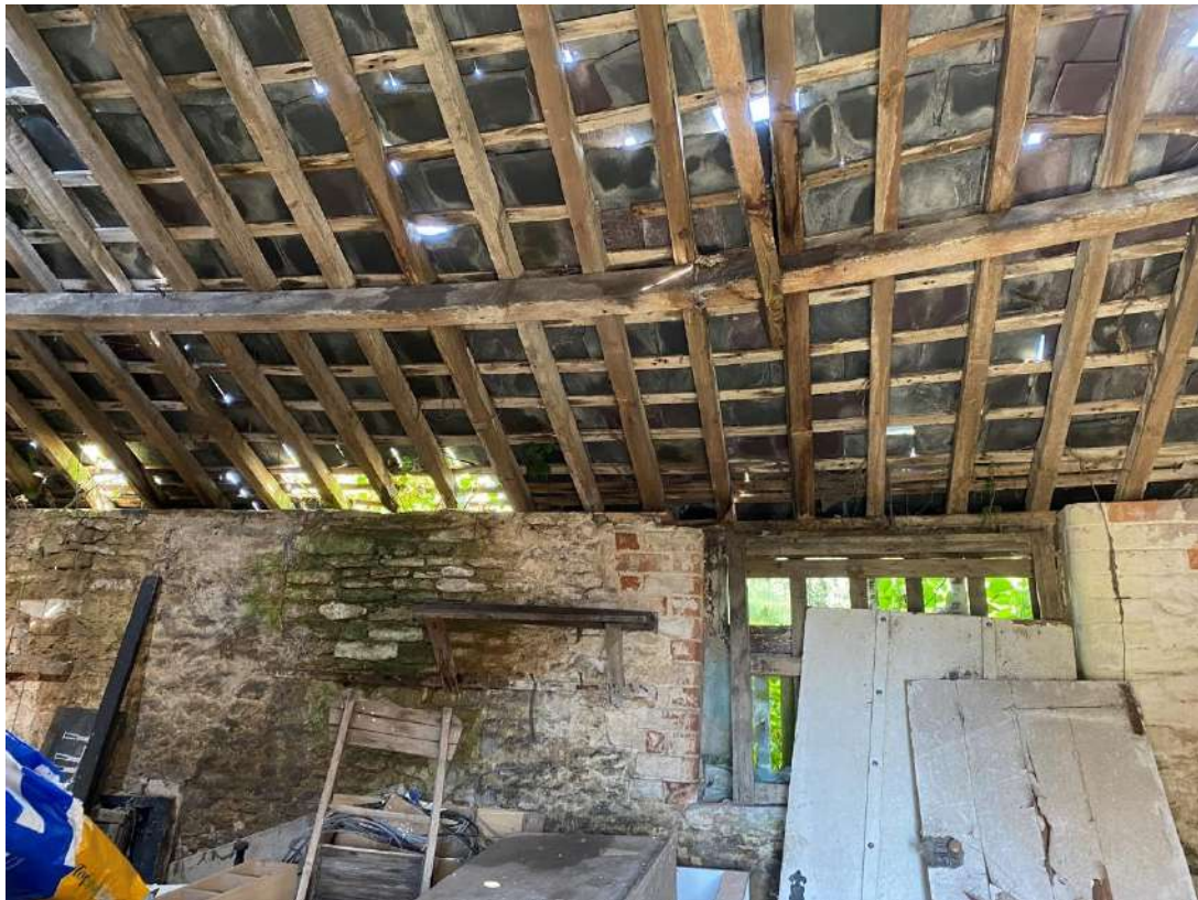
Figure 4 - Evidence of Moisture Penetration, Decay of Timber Rafters and Failure of Supporting Purlin
