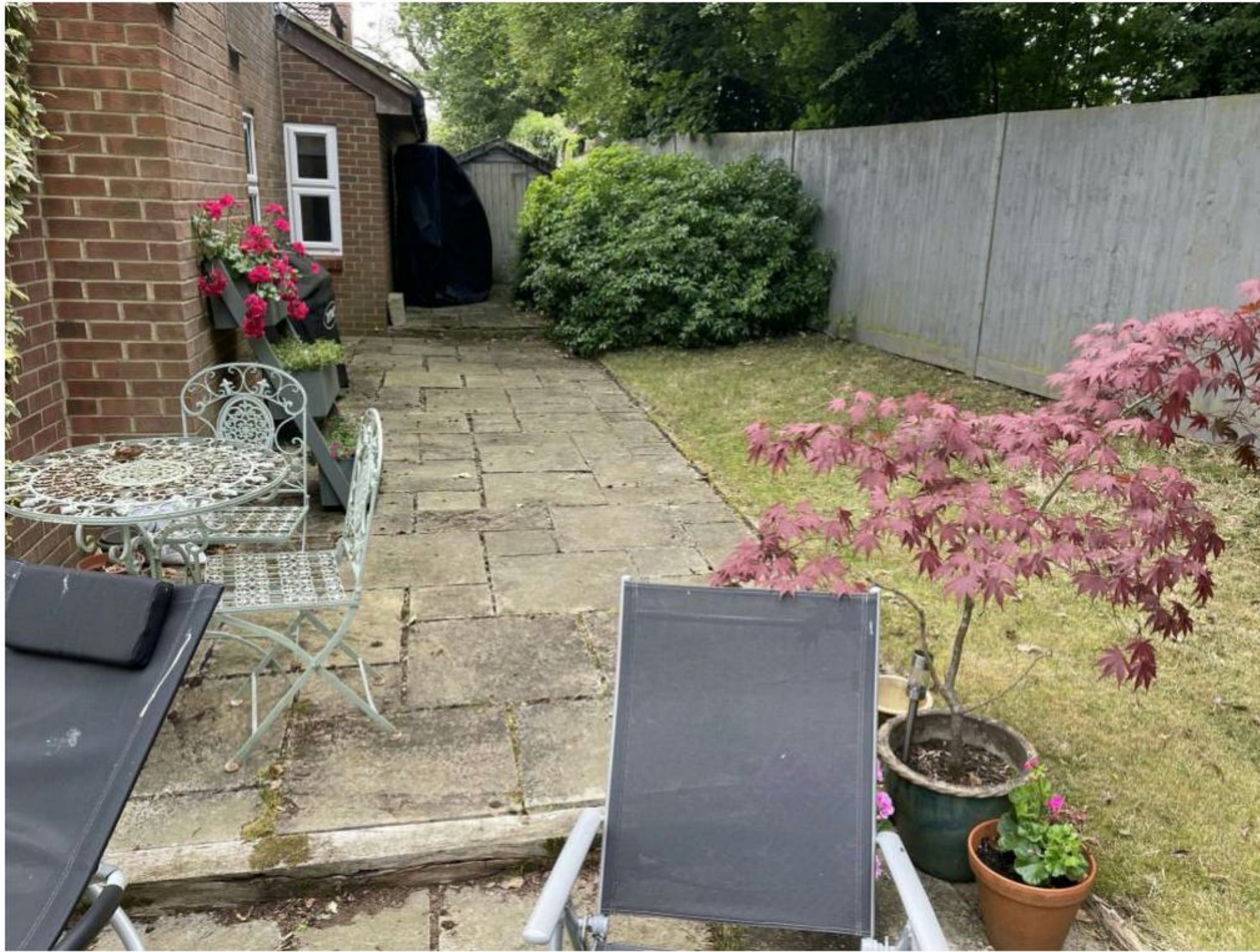
Photo shows the paving down the left hand side of the house which will need to be lifted and relaid.
