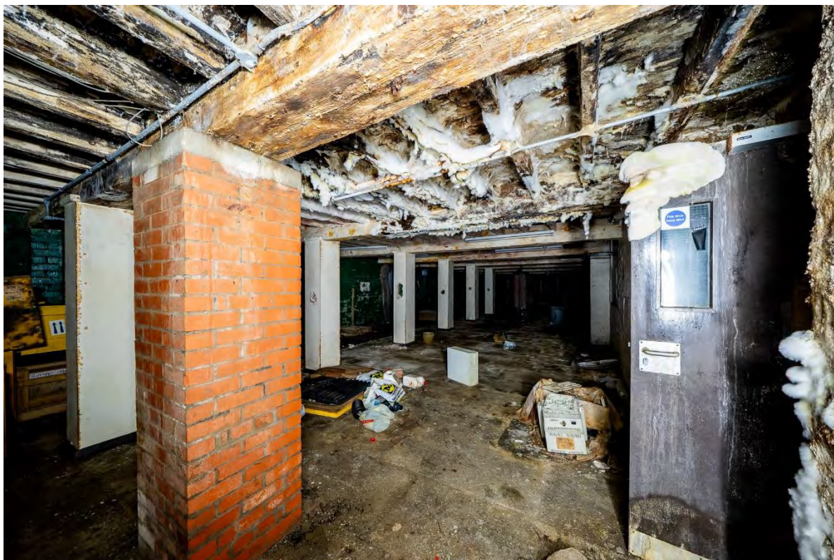
Photo 30: Overview of basement below the south range, facing southwest. Note the extensive rot and modern brick pier
