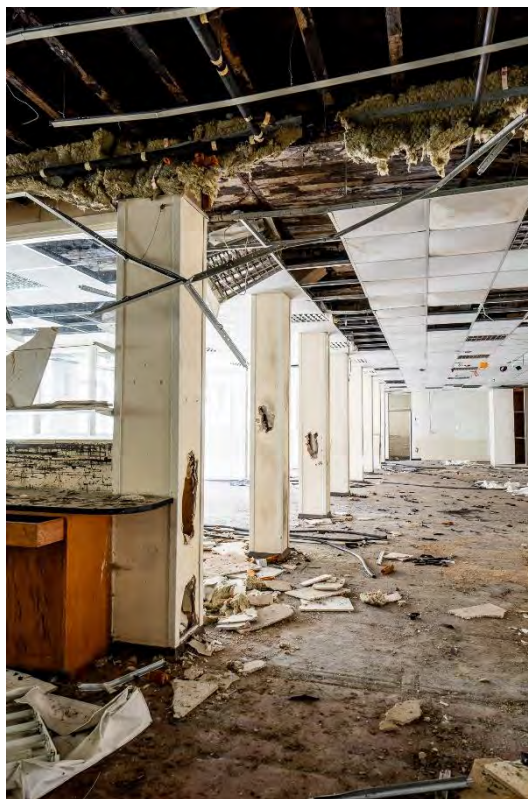
Photo 14: Row of columns to the second floor of the south range, facing west
