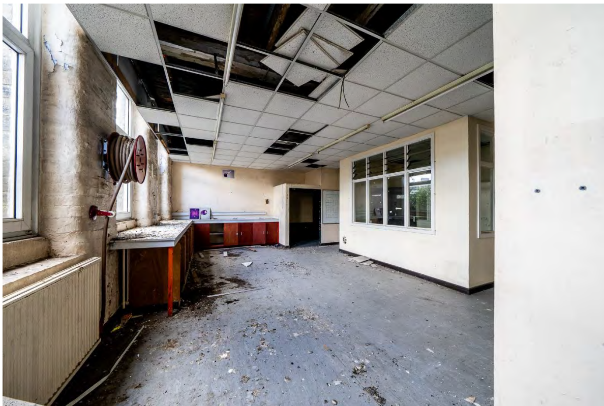
Photo 12: Third floor western room of the south range, facing east – note partitions
