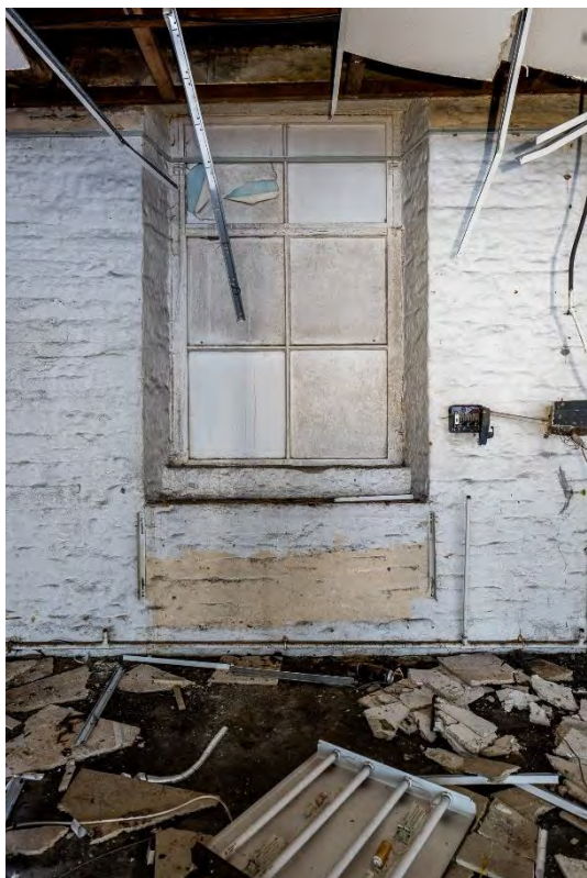
Photo 7: Retained window in former north elevation of the south range, facing north (second floor)
