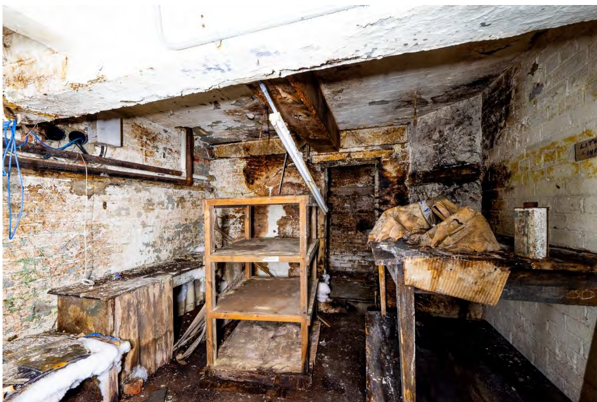
Photo 41: Northeast room of the north range basement, facing east. Note the extensive rot
