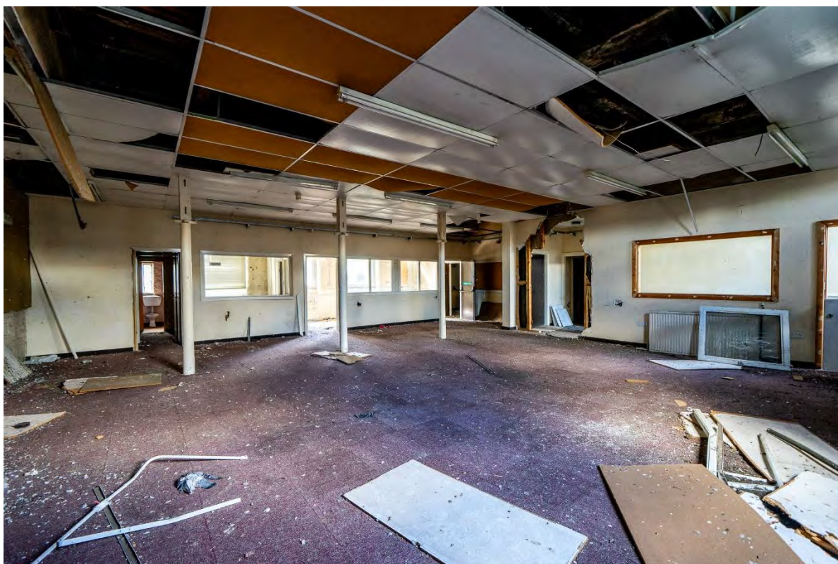
Photo 13: Third floor eastern room of the south range, facing southwest – note exposed columns
