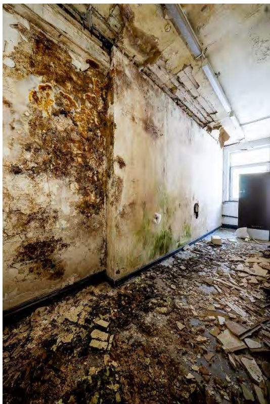
Photo 44: Extensive dry rot at eastern end of the north range (ground floor), facing northwest
