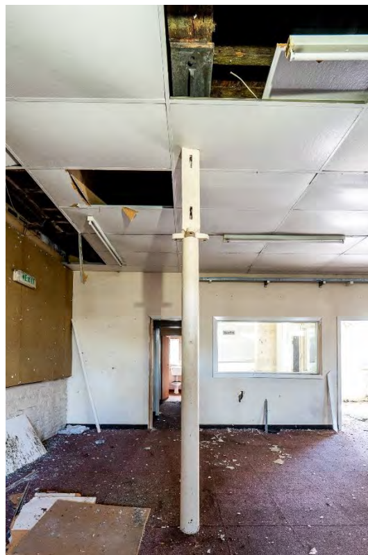
Photo 17: Exposed third-floor column
