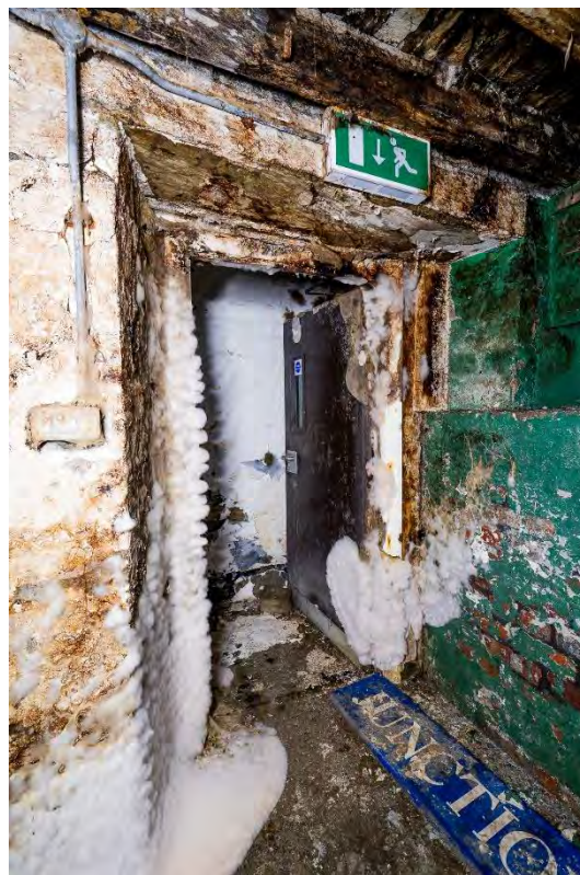
Photo 45: Dry rot at the base of the 19 th -century stair within the basement, facing north
