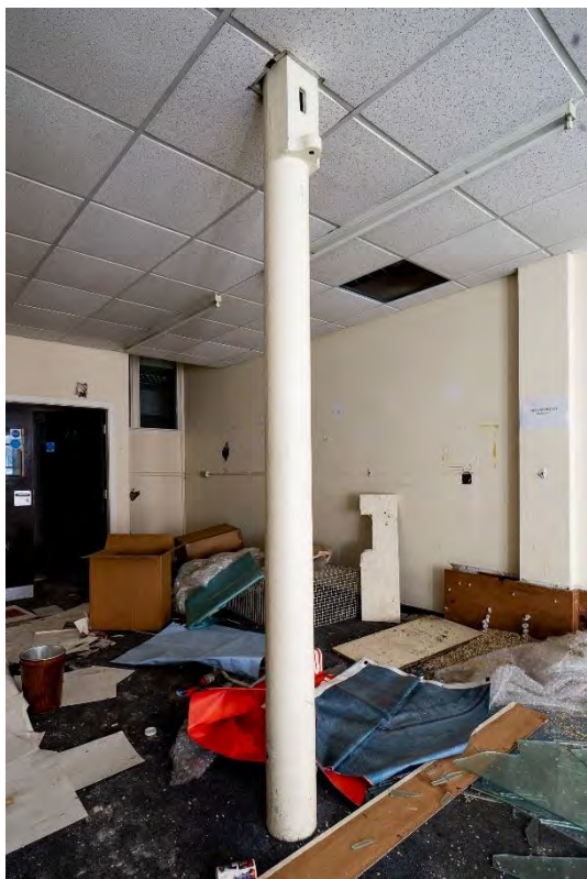
Photo 16: Partially exposed ground-floor column
