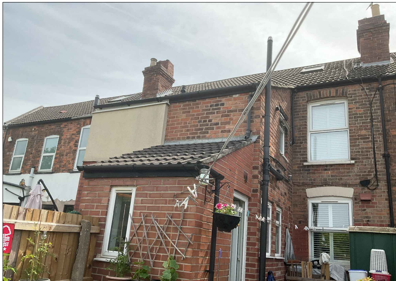
Rear elevation- The single storey projection with the back door looks to be a newer addition and is likely to have a cavity wall, so wouldn't be fitted with EWI.
