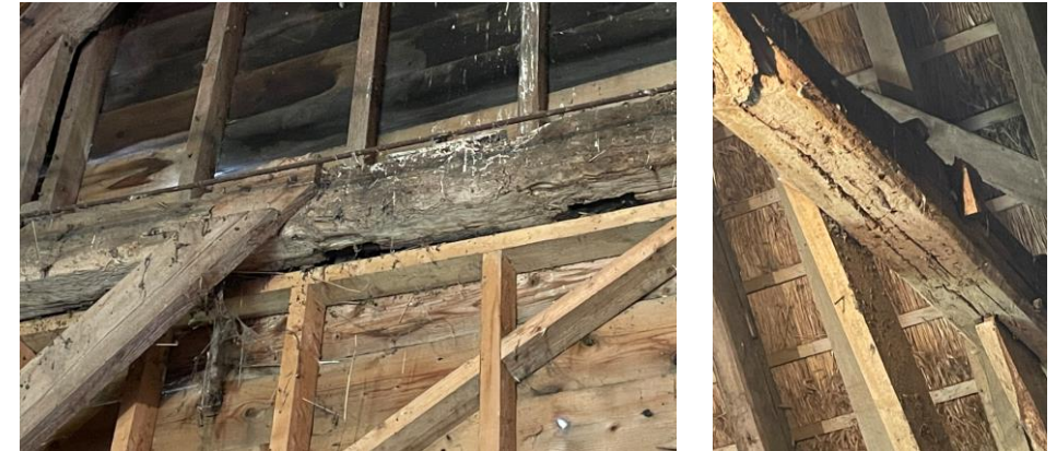
Fig.24 left - F4 insect damage, right - cracking and loss of section to F3
