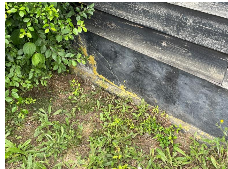
Fig.28 external plinth cracking
