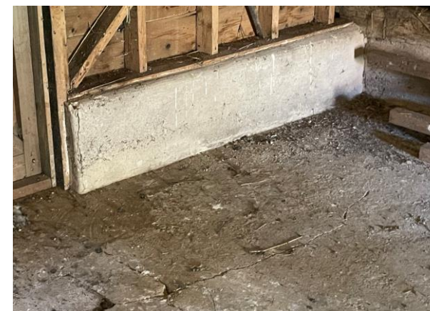
Fig.26 plinth and floor slab cracking
