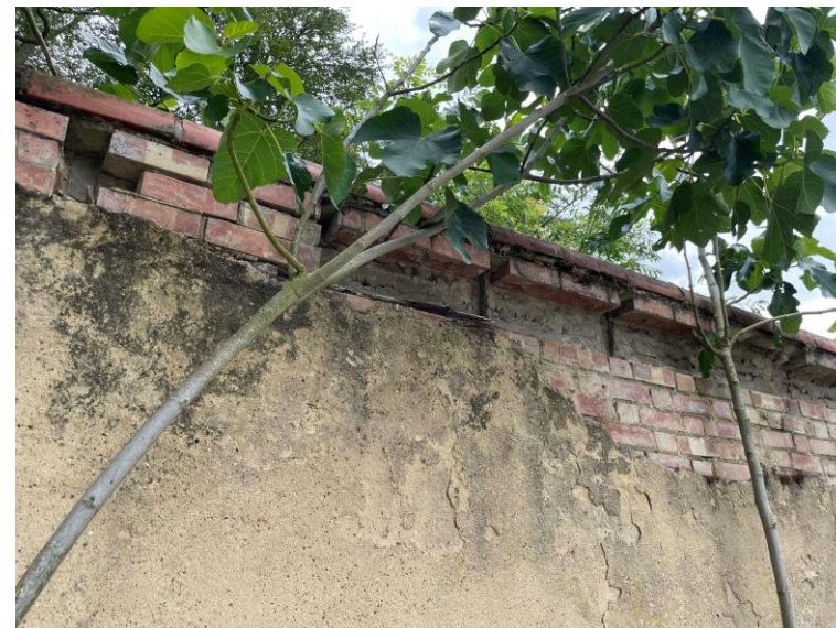
Fig.7 garden wall condition
