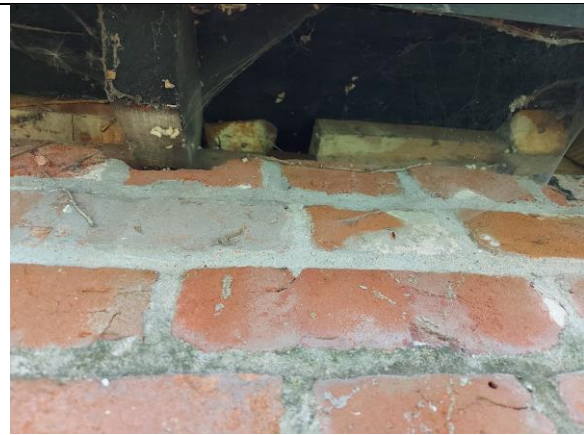
Photograph 10. Hole in north elevation B2 with possible bat dropping beneath.
