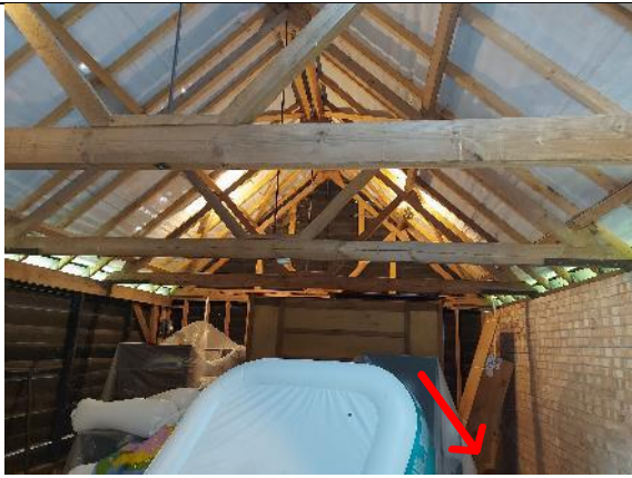
Photograph 13. B3 internal showing gaps above walls either side. Red arrow indicates area bat droppings were found.
