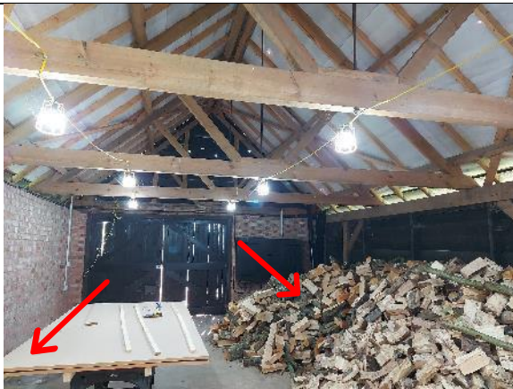
Photograph 15. B5 log store. Red arrows indicate location bat droppings were found.
