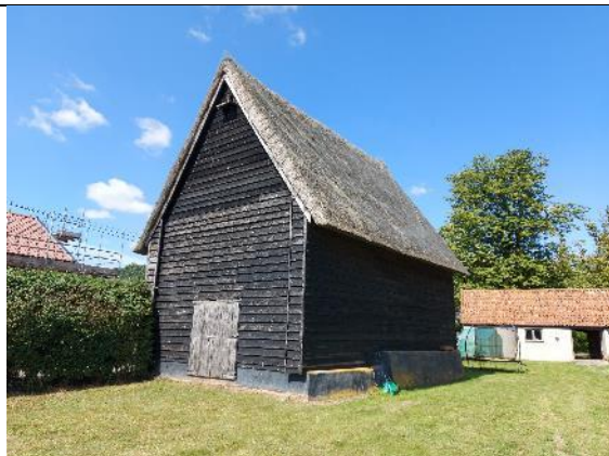
Photograph 5. B1 east gable end with defunct bird access at apex.
