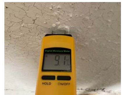
Damp Basement Storage Area.
