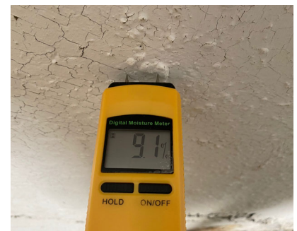
Damp Basement Storage Area.
