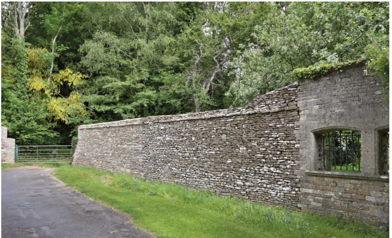
Fig. 23. Detail of the north wing wall showing the rebuilt section at its northern end adjacent to the private gated access to land outside the ownership of Ampney Park.
