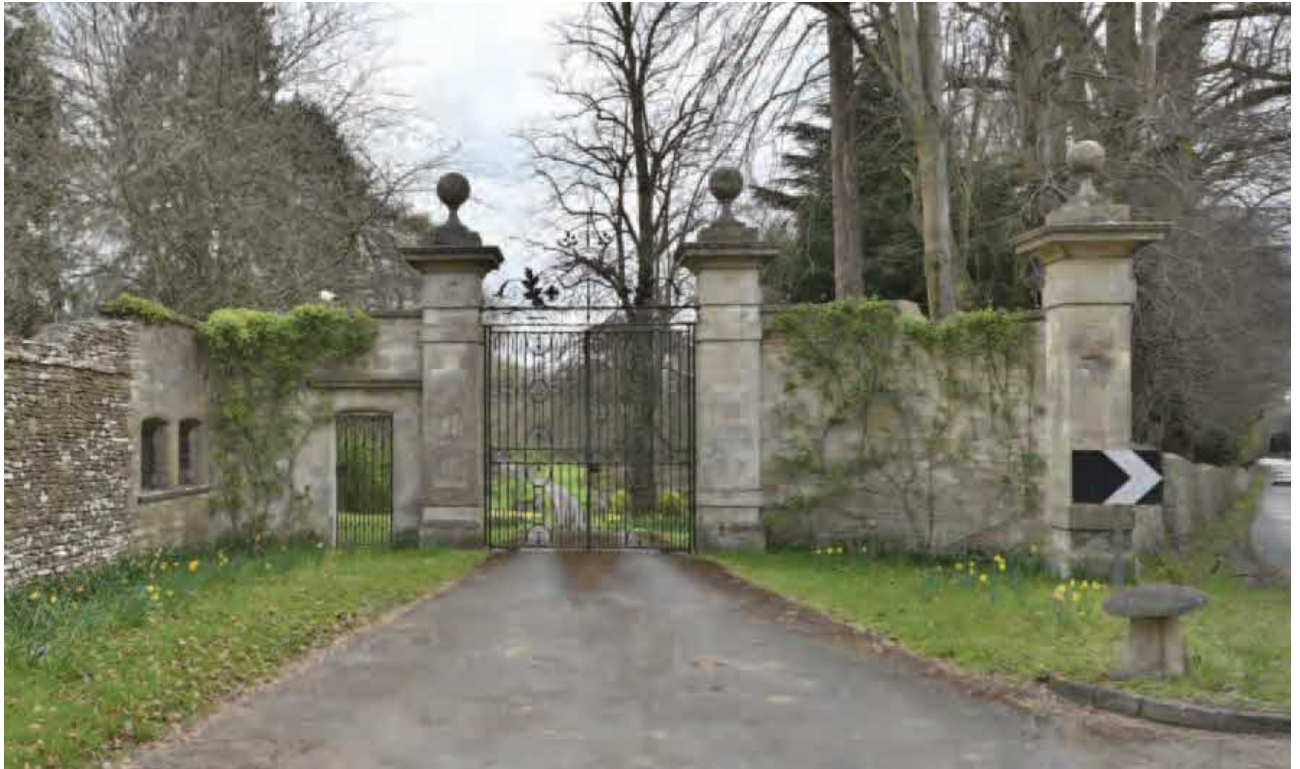
Fig. 22 The early 20th century (erected between 1902 - 1920) west entrance to the park with its asymmetrical form and stone rubble extension to the north wing wall (shown prior to repair of the collapsed section). The north wall continues westwards as a tall coursed rubble wall enclosing the open ground adjacent to the entrance, and limiting views towards woodland and pasture. A section of this wall has recently been rebuilt following vehicle impact damage. At the west end, the wall is separated from the road by a field gate opening onto a wooded track.
