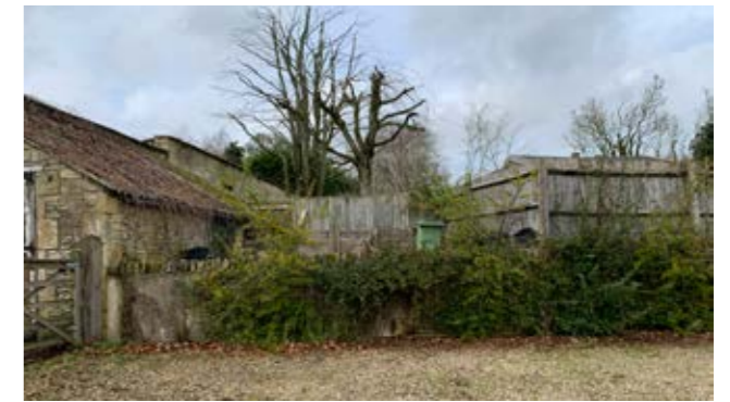
Poor existing conditions of the proposed garage area
