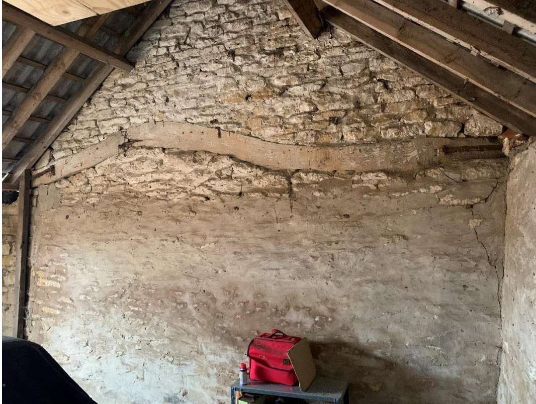
P14, above - north wall of garage showing tie beam encased in masonry.
