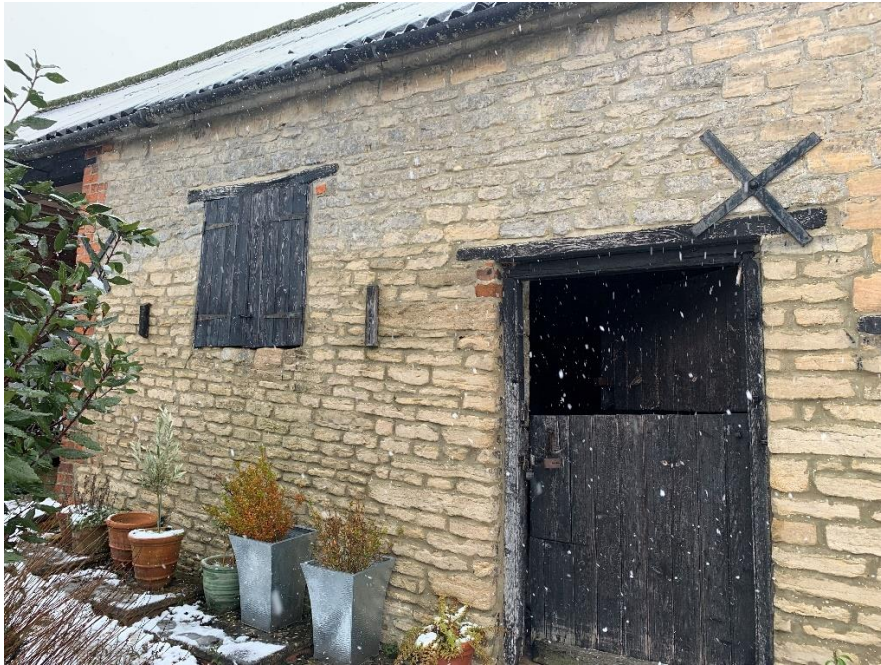
P12 left – historic shutters on cast-iron hinges and a dowel framed bead moulded plank stable door.
