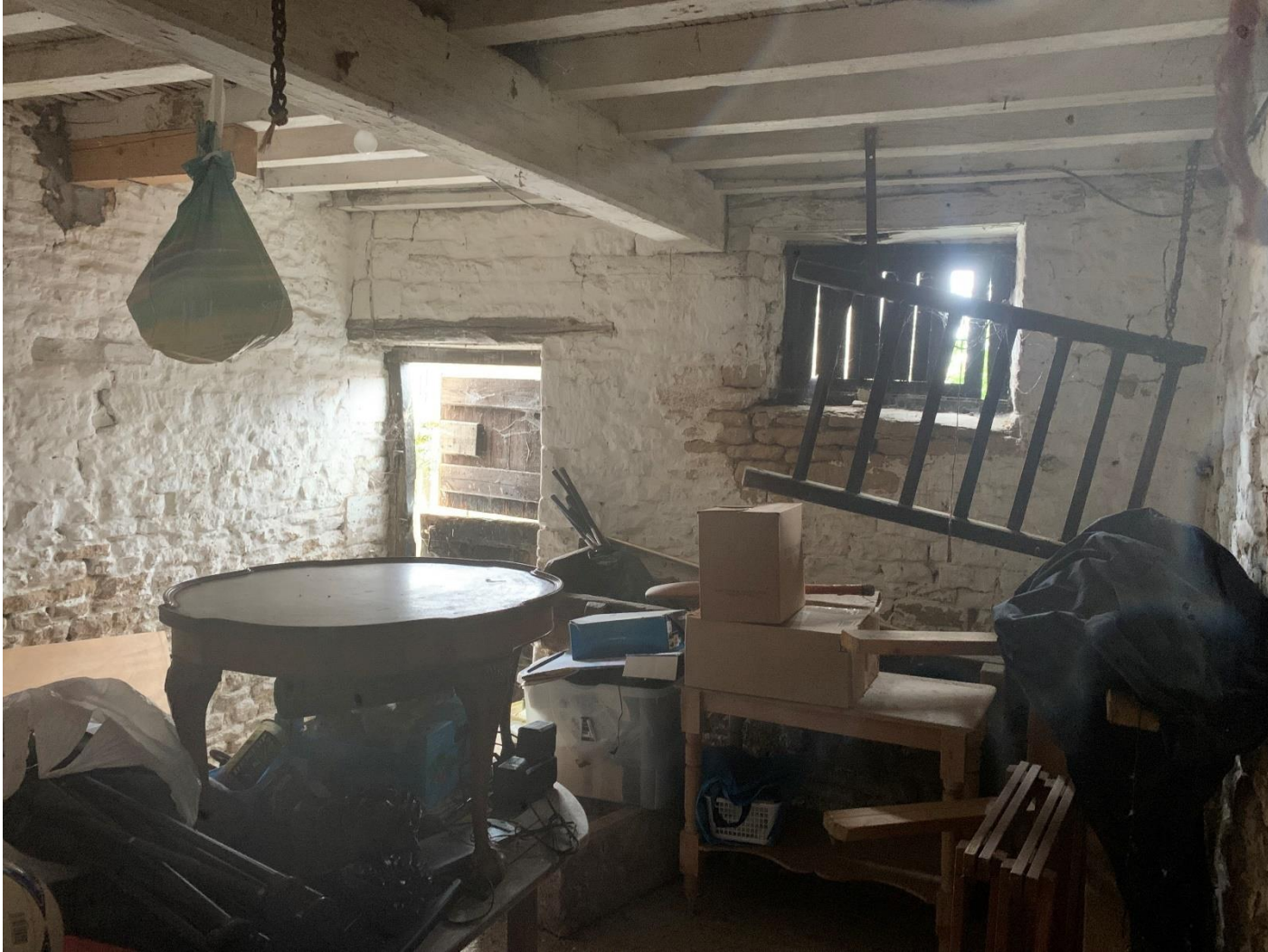
P19 – Barn 3, with beam and rafter ceiling, slatted breather vent to opening, timber lintels above the door and window opening.
