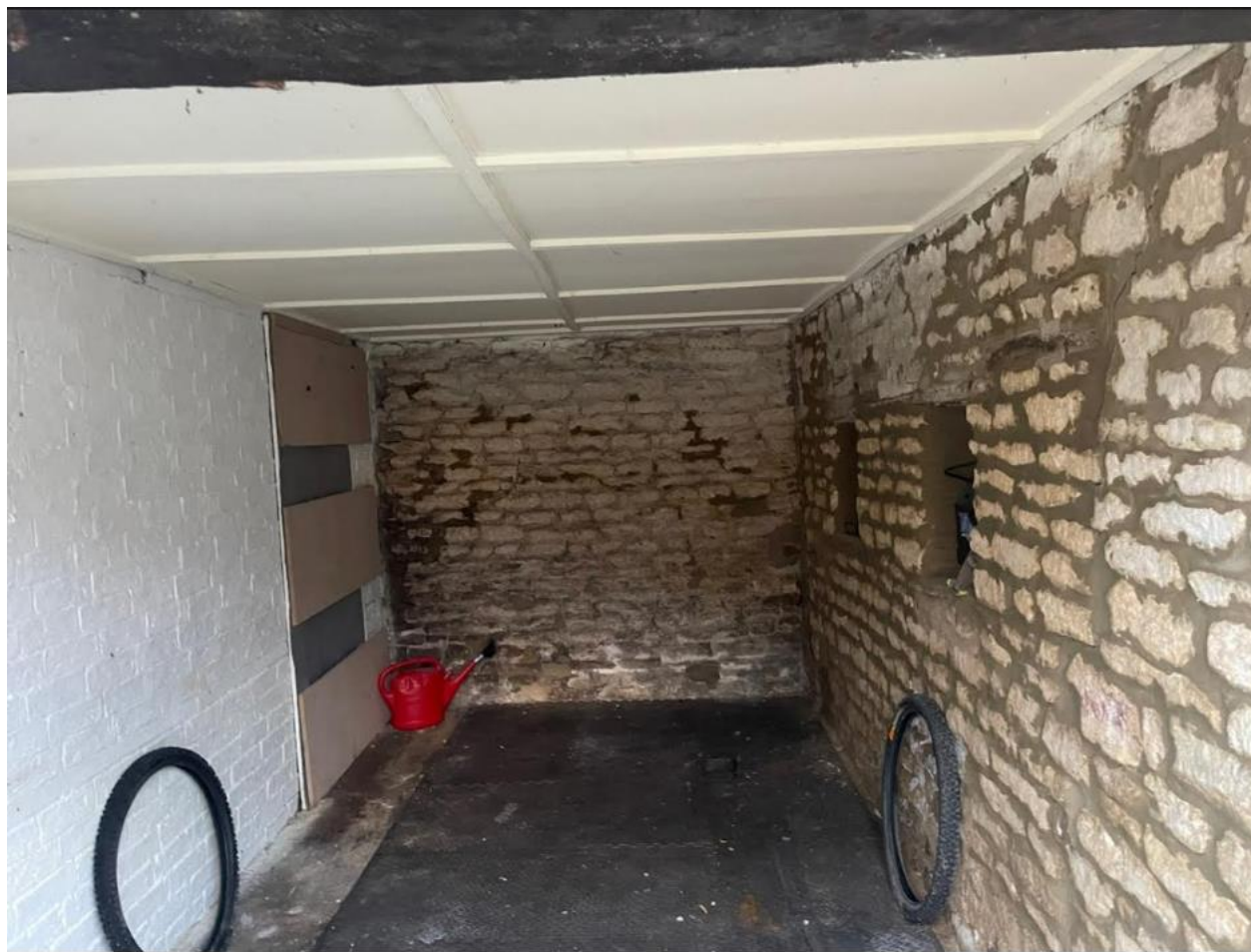
P26, Barn 2 (photo kindly supplied by the owner of the stone barn after removal of stored goods). Modern cement pointing to the walls, concrete floor, modern boarding to the ceiling and a blocked opening.
