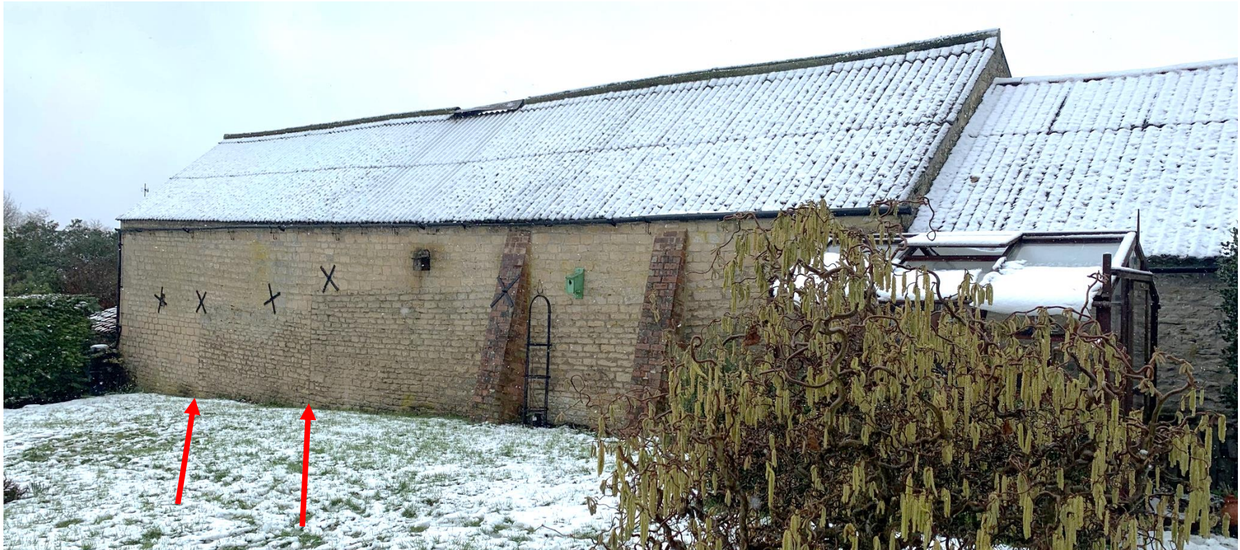
Fig 3, note the east elevation which shows part of an earlier building has been incorporated into the Stone Barn. The red arrows indicate clear joints in the building showing separate but conjoined structures. The earlier stonework is not laid level but runs at an angle following a rise in the land. Later coursing has 'levelled' the coursing.
