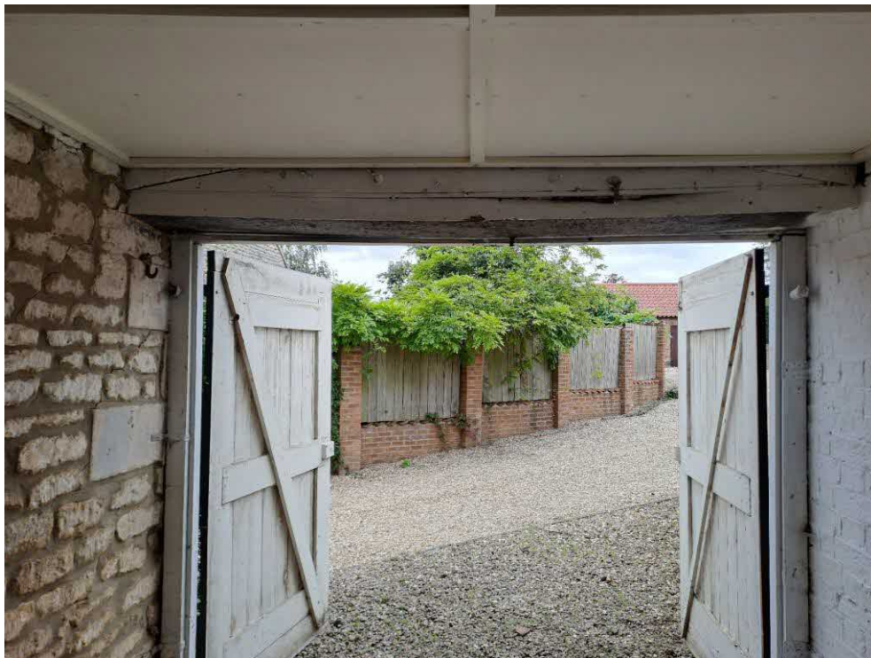
24 Barn 2. Minor deflection to timber lintel.
