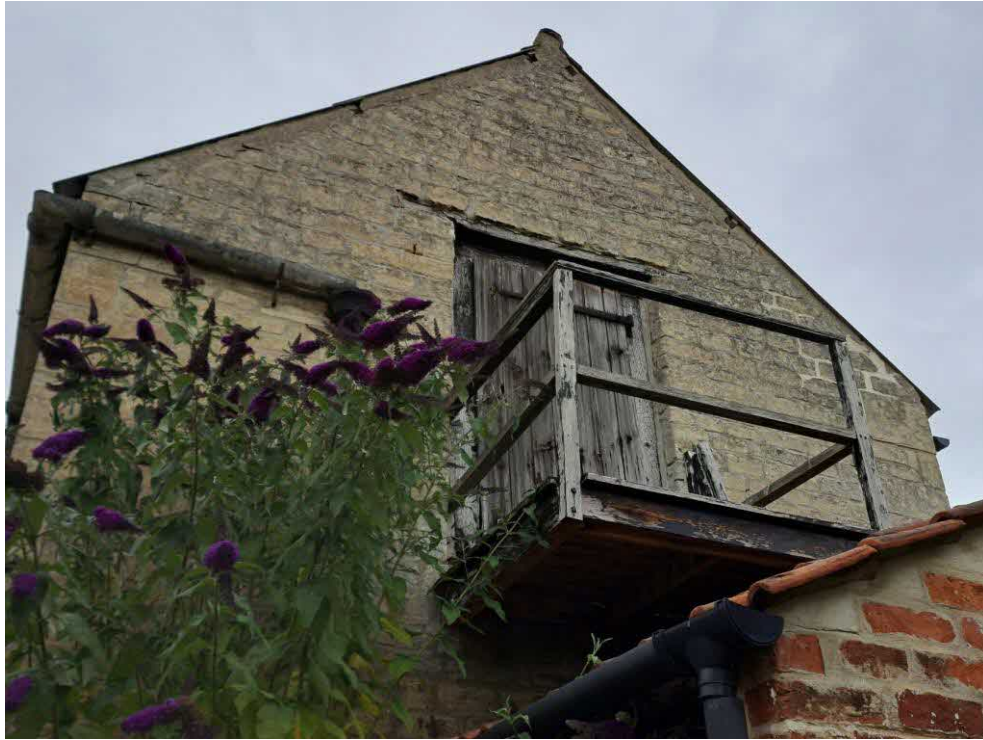
11 South elevation. Fine cracks to top of gable along eaves and west kneeler. Previous repairs around the east kneeler.
