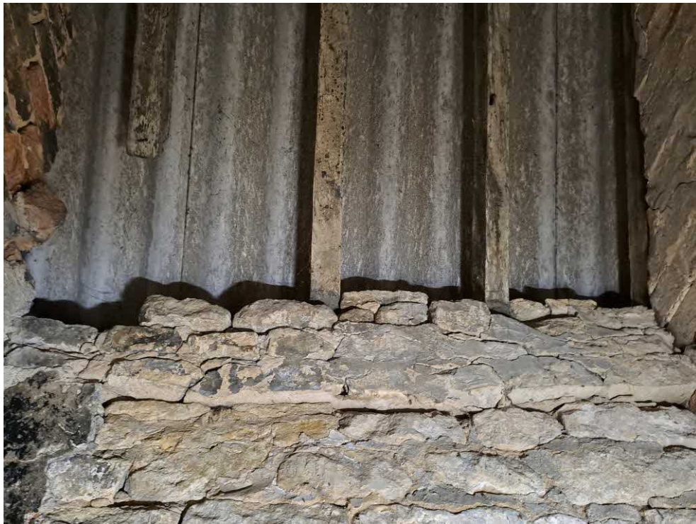
38 Stair roof. Three top courses displaced inwards. Missing rafter end to wall.
