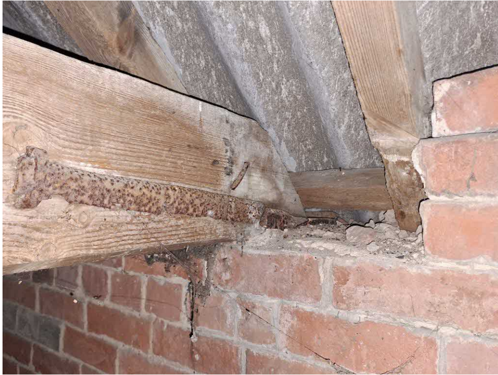
37 Store 2. Tie beam bearing on the east wall. Fractured iron tie. Reduced section to rafter foot.
