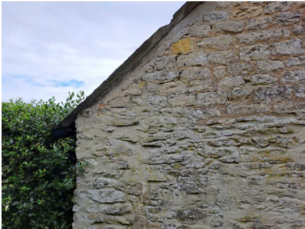
6 North elevation. Fine cracking and open joints close to eaves and connection with east and west elevations.
