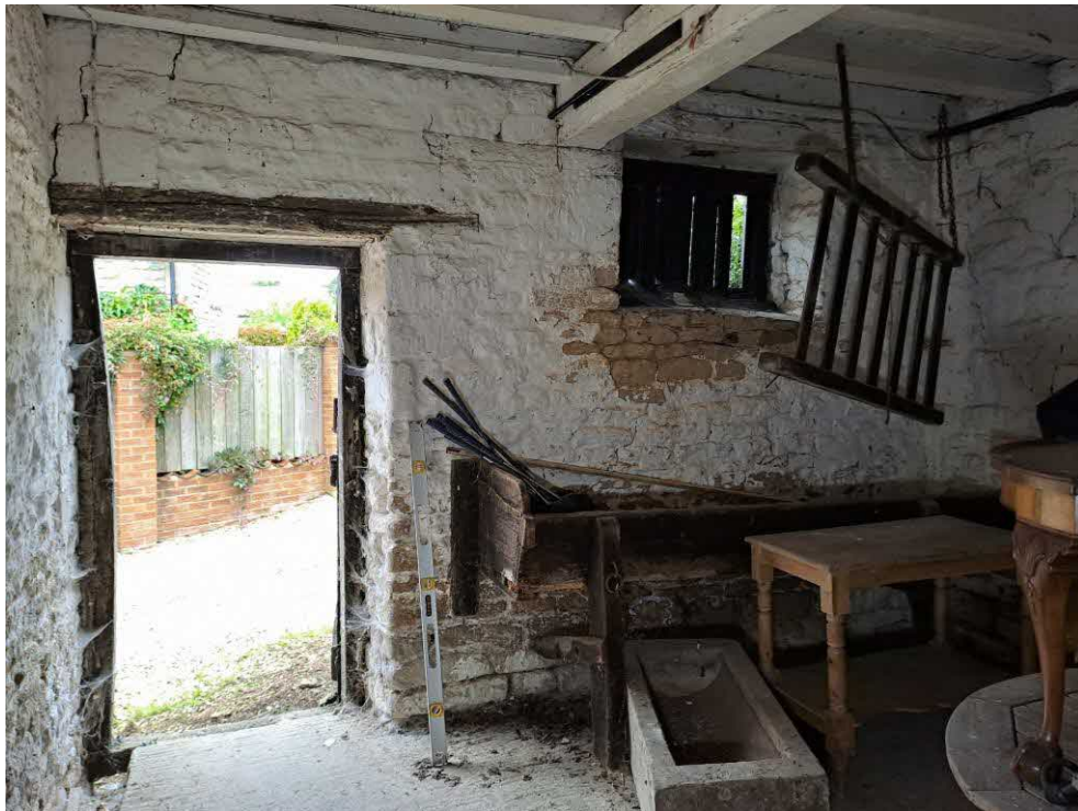
28 Barn 3. Fine diagonal cracks below and above window. Slight diagonal crack above the lintel. Deep recessed open joints and efflorescences to base of the west wall.
