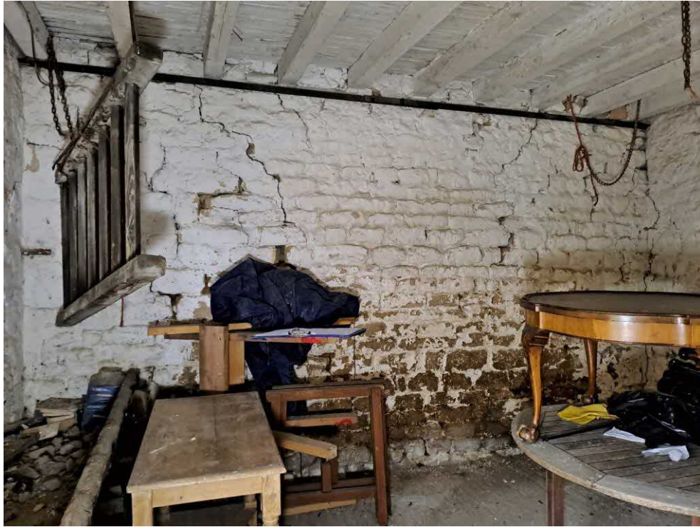
27 Barn 3. Fine to slight diagonal cracks and open joints to wall on the north side. Deep recessed open joints to the base of the west wall.
