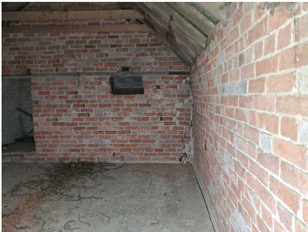
36 Store 2. Separation between the floor and east wall. Moderate deflection from the centre to the east wall. Inwards displacement of top three courses. Diagonal fine stepped cracks, very severe open joints, and fractured bricks to second-floor brick wall.
