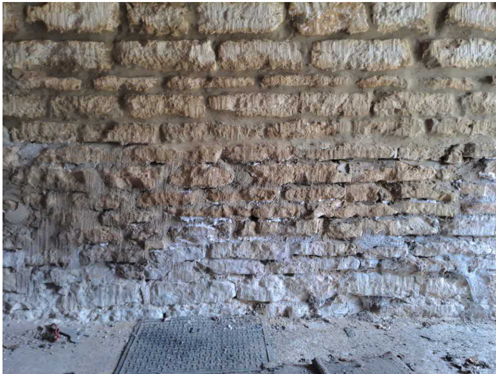
16 Garage. Efflorescence to the base of the wall.
