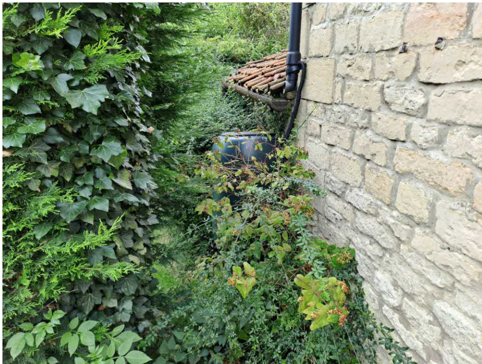
10 East elevation. Vegetation growth close to the wall. Interrupted drainage system.
