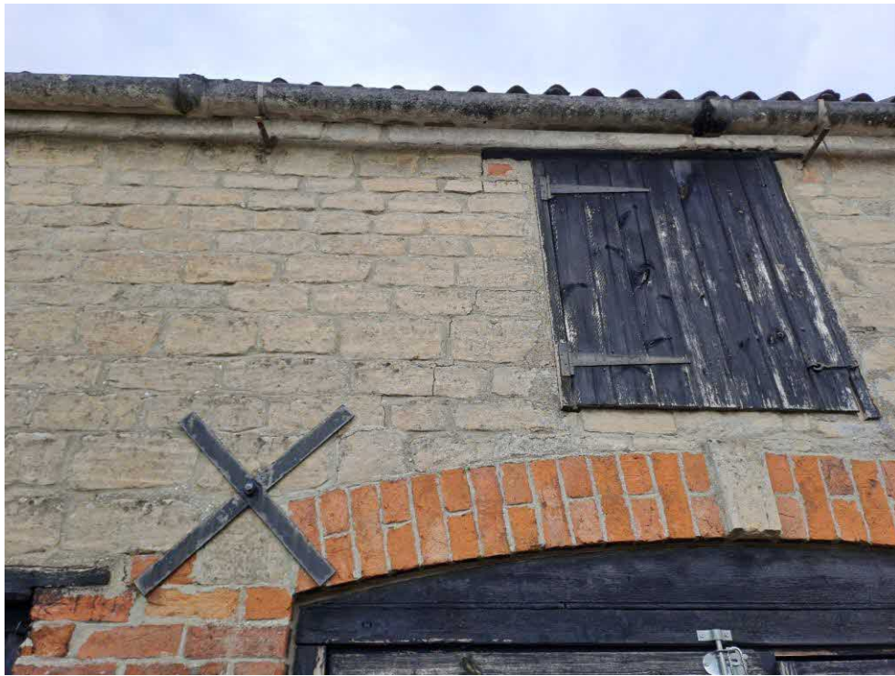
3 West elevation. Fine diagonal crack from the first-floor window in Store 2 to the cross-shaped plate.
