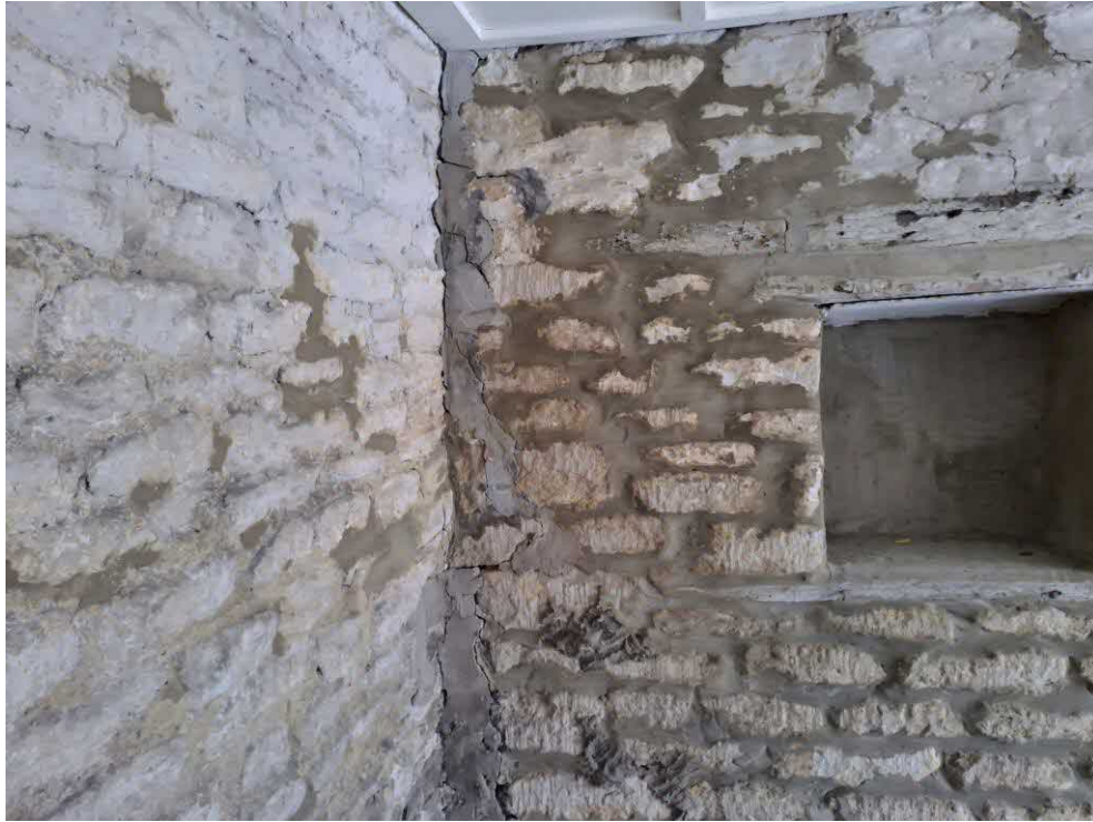
23 Barn 2. Fine to slight diagonal cracks, full height, to previously infilled joints.
