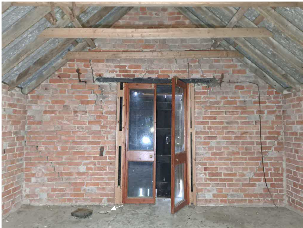
32 Store 2. Moderate to severe diagonal open joints to brick inner leaf of south gable. Fractured lime-ash floor with small hole near the door.
