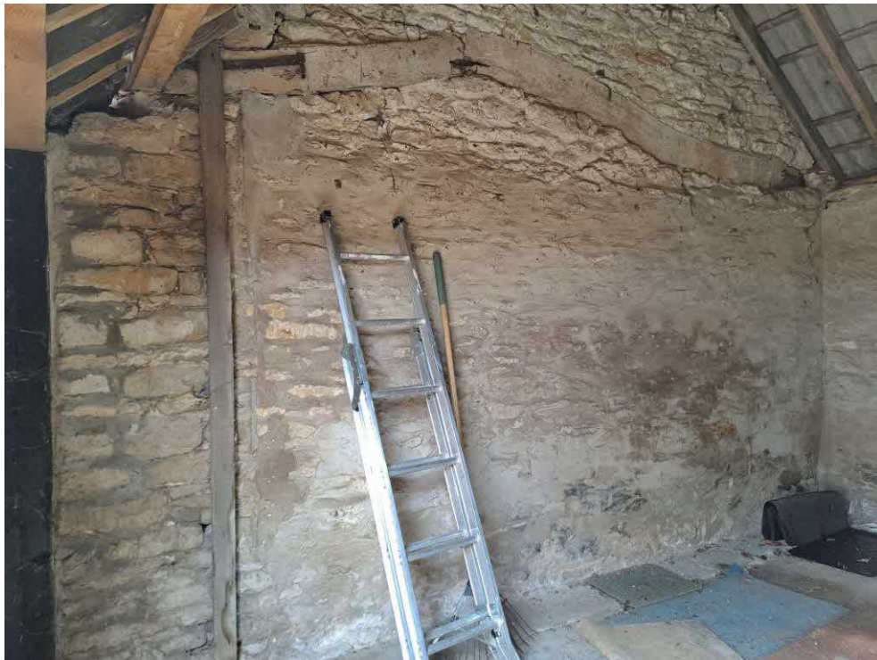
18 Garage. Historic bent tie beam with iron ties embedded in the north wall. Fine vertical crack, full height, at the northeast corner.
