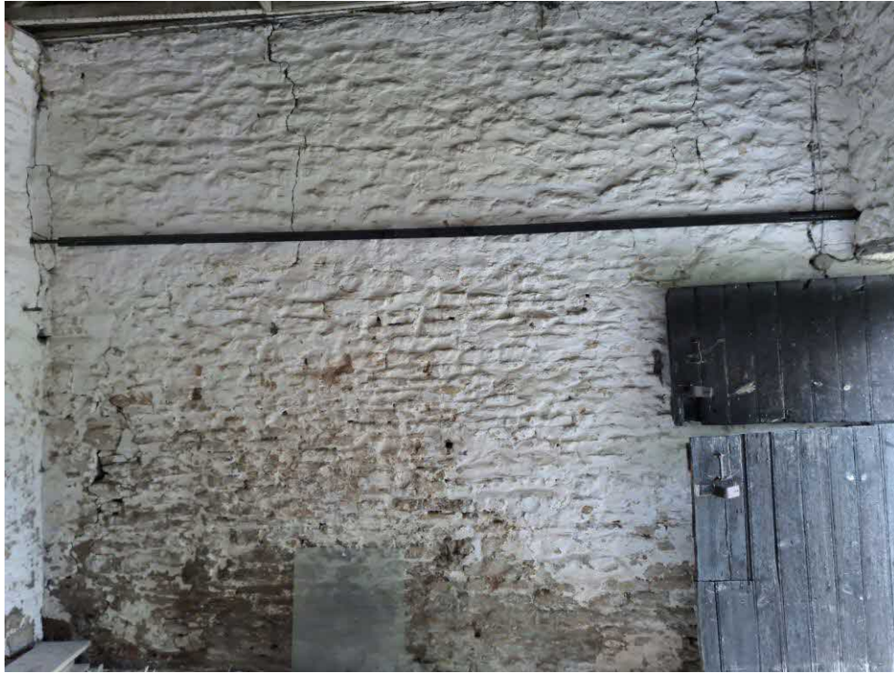
19 Barn 1. Slight vertical cracks to the top half of the wall. Steel tie anchored to the west and east walls.
