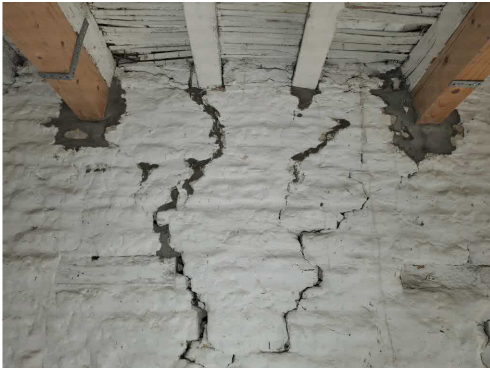
26 Barn 3. Vertical moderate open joints at the centre of the wall. New timbers added to existing joists. Infill at bearings and cracks with cement mortar. Twisting of joists.
