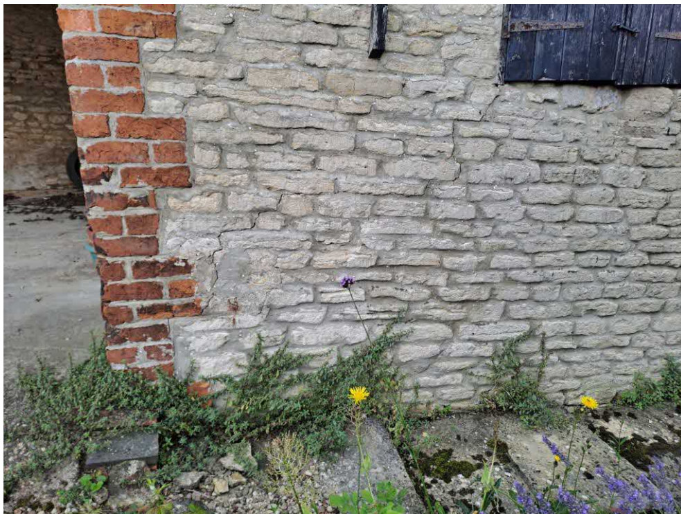
4 West elevation. Fine diagonal and bed joint crack from the corner of the window in Barn 1 to the base of the brick wall.
