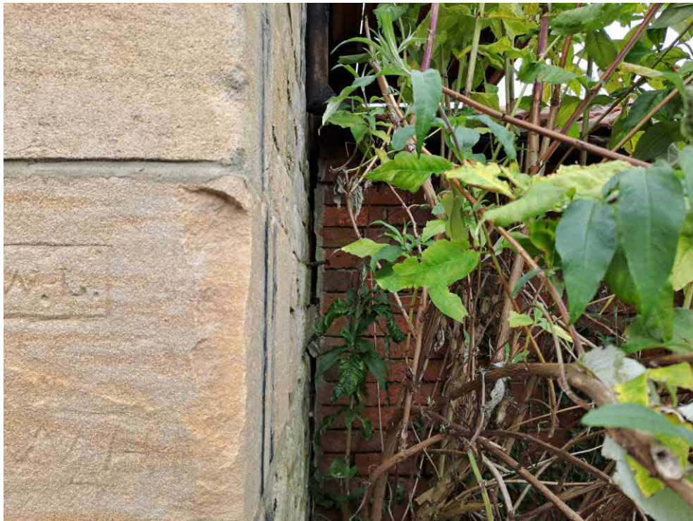
12 South elevation. Separation between the brick wall of Store 1 and the stone wall of Barn 3. Vegetation growth close to the walls.
