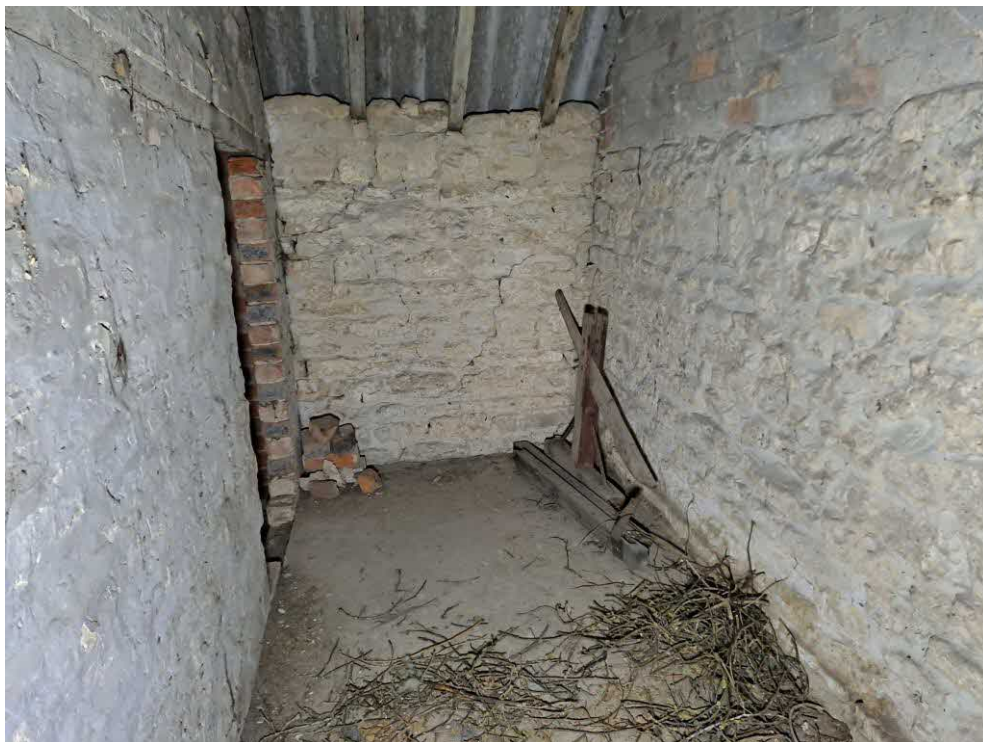
30 Stair 1 st floor. Diagonal fine cracks to the inner face of the west wall.
