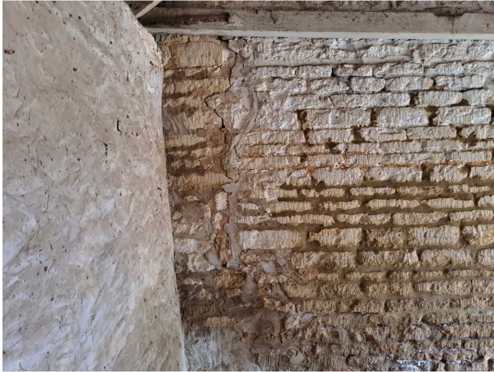
17 Garage. Open joints and cracking to connection between pre 1824 wall and 1824-1888 wall. Connection previously repaired.
