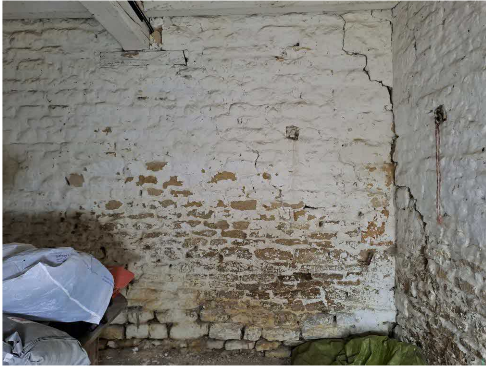
25 Barn 3. Fine to slight diagonal stepped cracks to east wall. Severe open joints to south wall and connection to east wall. Deep recessed open joints to the base of the walls.
