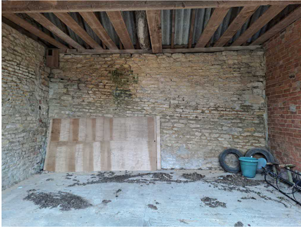
15 Car port. Wall with stonework from different construction periods (bottom pre-1824) and top from 1824-1888. Severe outward lean to wall.
