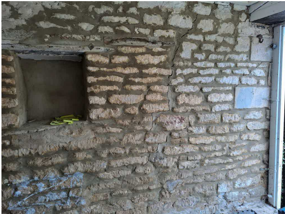
22 Barn 2. Fine to slight diagonal cracks, full height. Joints previously infilled.
