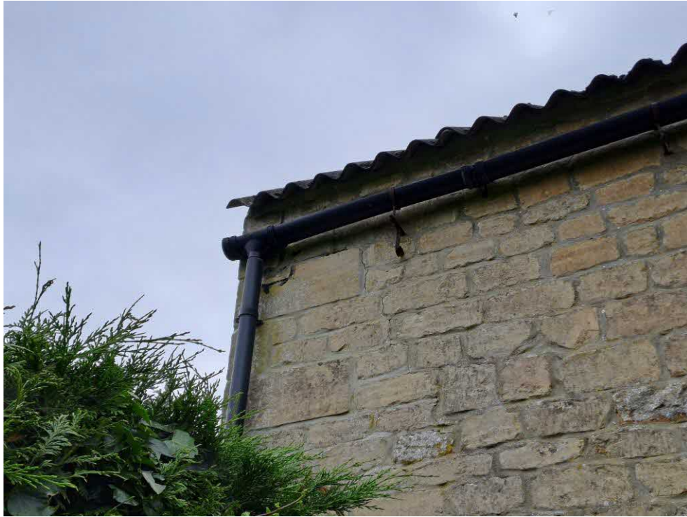
9 East elevation. Fine cracks to the wall starting from the kneeler.
