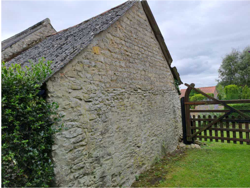
5 North elevation. Distinct stonework from possible different periods of construction. Vegetation growth to the top of the northeast corner.
