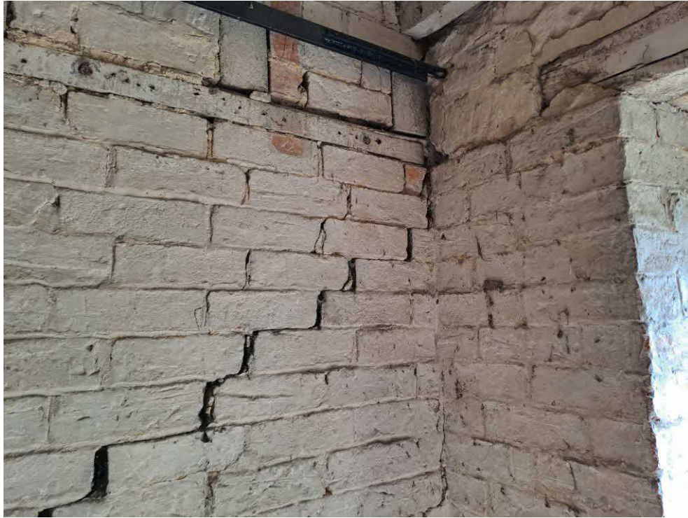
21 Stair. Diagonal fine stepped cracks and moderate open joints (full height) to brick wall. Detail of the tie end: threaded bar bolted to flat plate.
