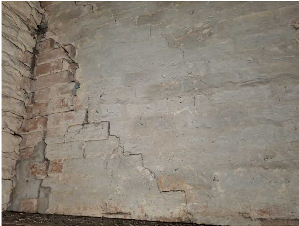
29 Stair 1 st floor. Diagonal fine stepped cracks, very severe open joints, and fractured bricks to second-floor brick wall. Complete separation of east wall.
