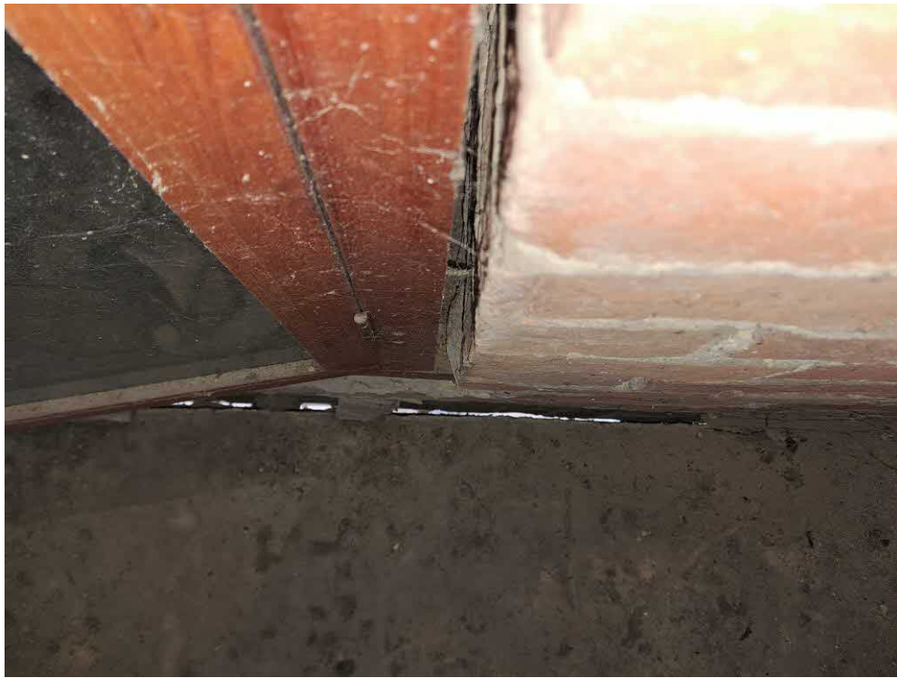
35 Store 2. Separation between the floor and west wall. Separation between window timber frame and brick inner leaf.
