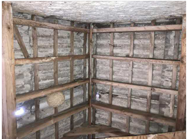
Underside of roof (note wasp nest)
