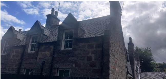
Photo 2: Eastern elevation with BRP at areas of loose and lifted slates. Wallheads are well-sealed with no BRP.
