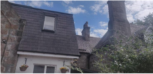
Photo 1: Northwestern elevation where new extension is proposed to be added. Slate roof is mostly well-sealed with low bat roost potential (BRP). The original roof behind it has a higher quantity of loose and lifted slated and moderate BRP.
