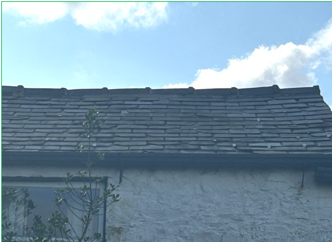
Showing crevices and gaps under the slates on the east elevation of the cottage
