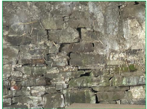
Crevices in the interior wall of outbuilding B
