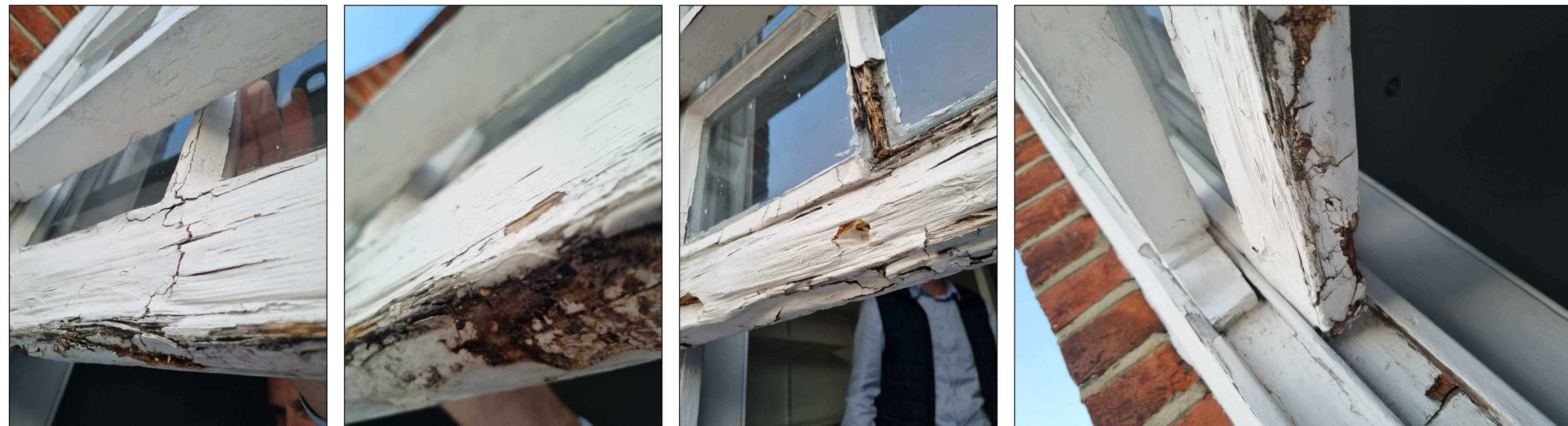
IMAGES SHOWING ROTTEN WINDOW
