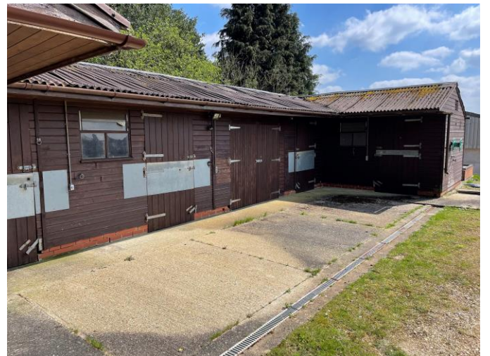
4. Front concrete hardstanding. Note the joints in the slab and drainage channel
