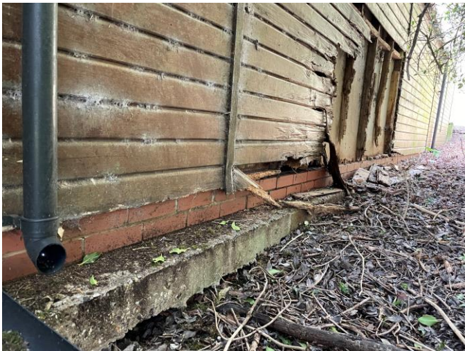
7. Rotten studwork and cladding on East side. Note the undermining of the slab
