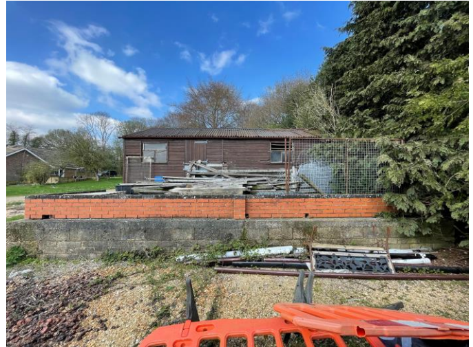
6. South Elevation. Note the retaining wall, change in levels, and poor condition of the windows and cladding
