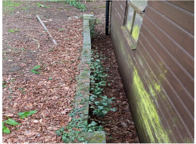
10. Block retaining wall distorted and bowed
