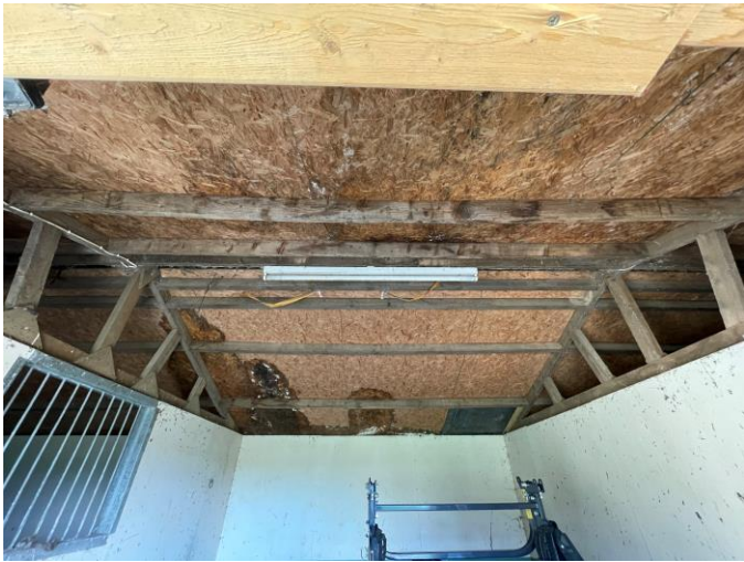
17. Lightweight purlins and damaged roof boarding.
