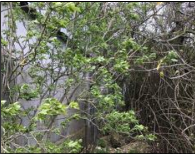
Image 17: Dense vegetation obstructs the east elevation of B2.
