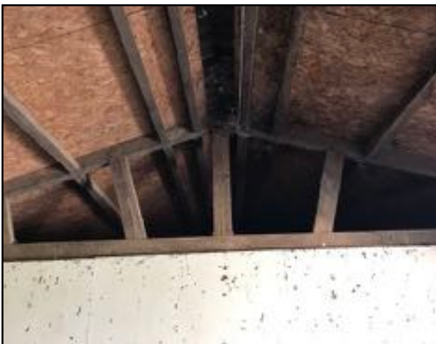
Image 11: The chipboard lining of the roof does not fully cover the ridge beam in B1.
