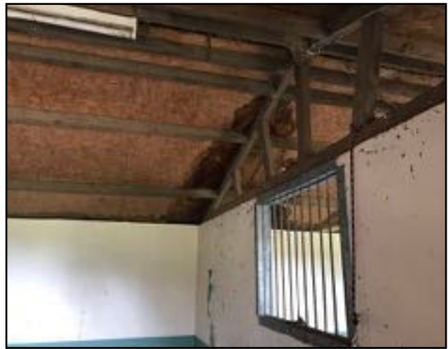
Image 8: An internal view of damp inside B1, indicating a leak in the roof above.
