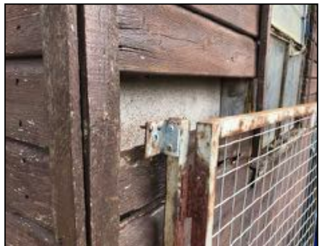
Image 6: A closer look of a damaged section of wall on the south elevation of B1.
