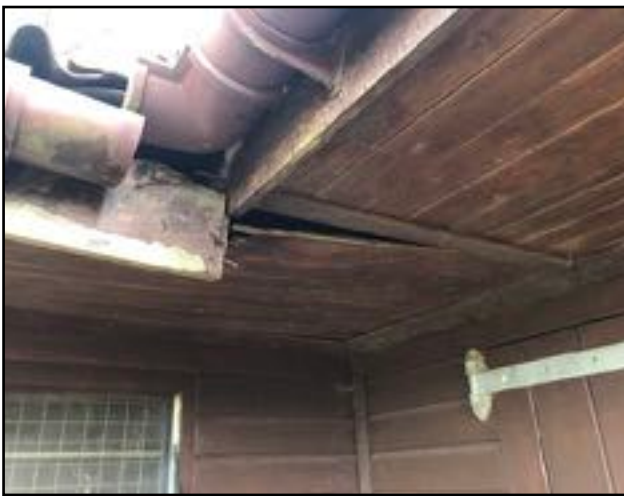
Image 9: An area of damaged soffit box on the west elevation of B1.
