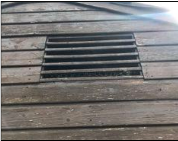
Image 7: Timber vents on the west-facing gable ends are blocked with chicken wire.
