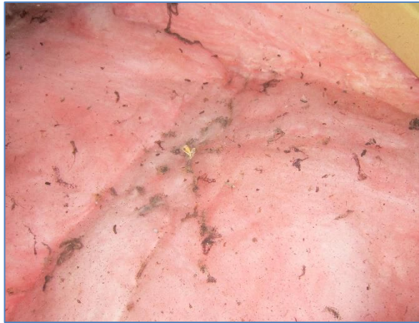
Scattered droppings within voids.
