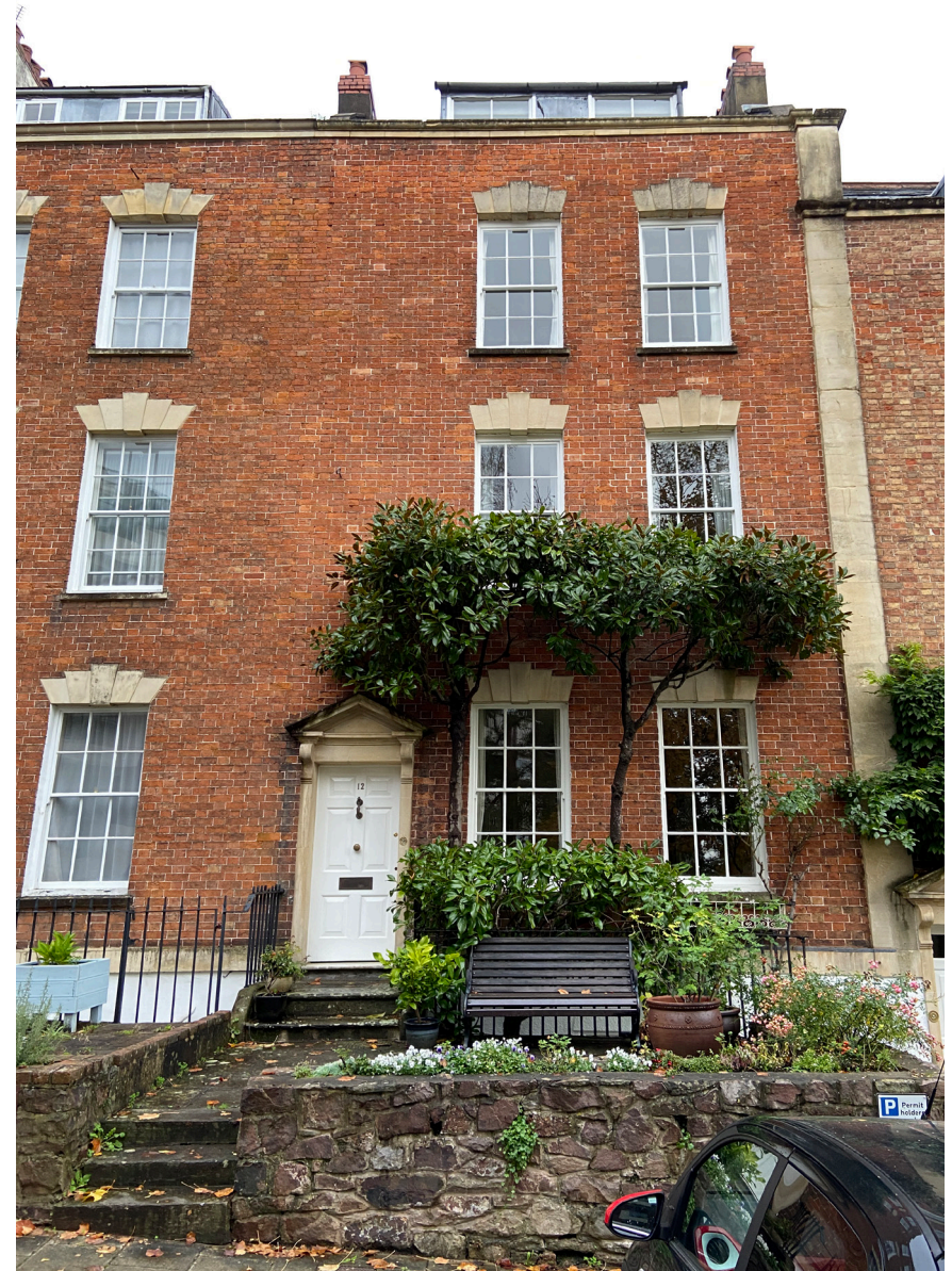
View of the front of 12 Hope Square showing the windows subject for replacement
