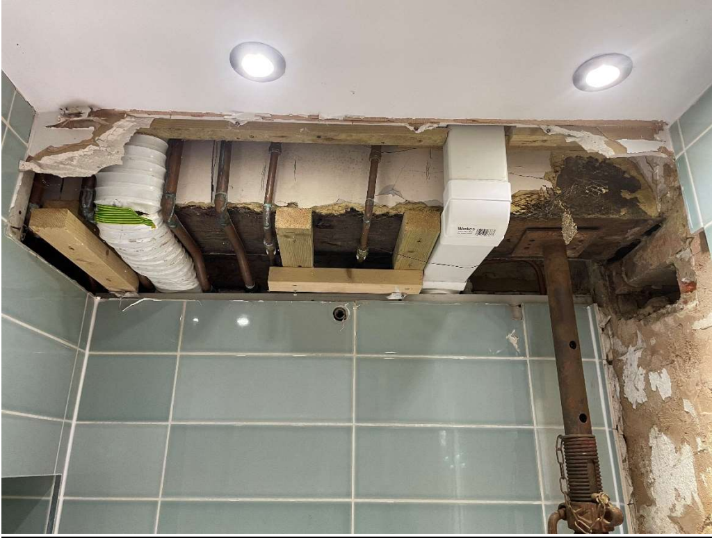
Timber Lintel to be replaced with concrete lintol
