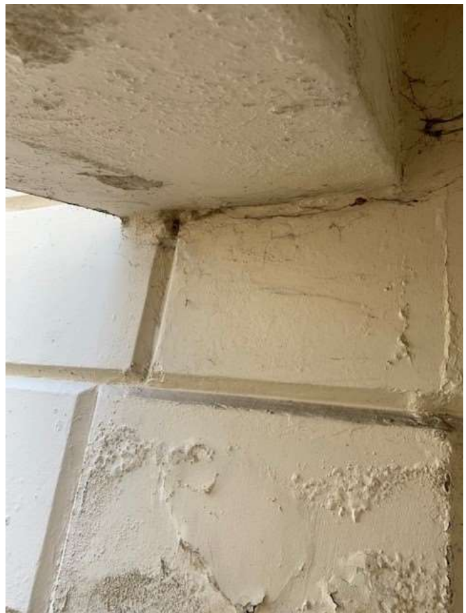
Figure e. Blistering of paint finish on stucco beneath steps
