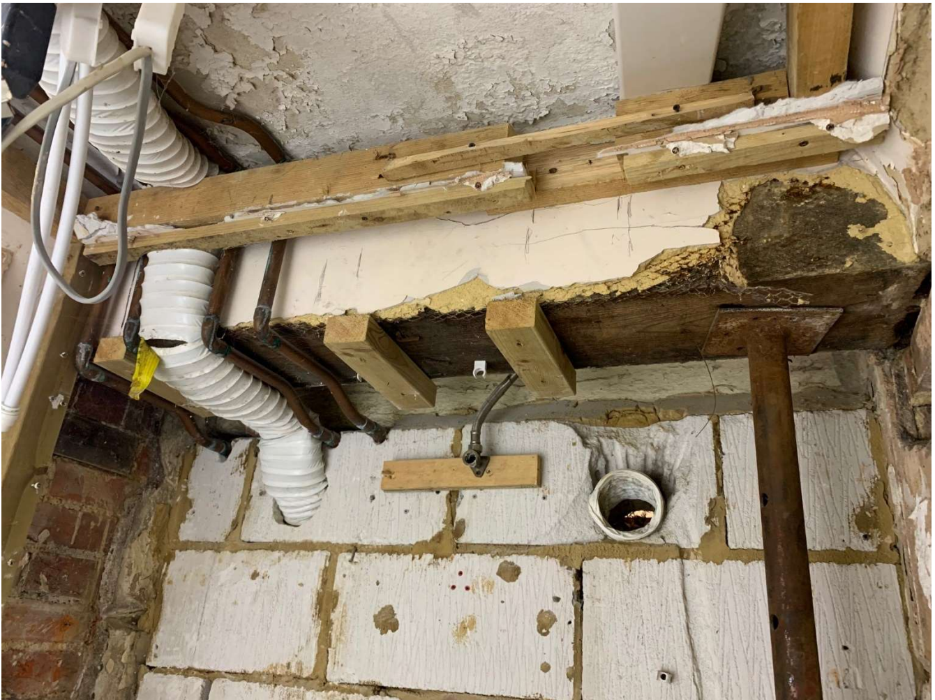
Figure a. High level timber beam in basement with blockwork infill beyond.
