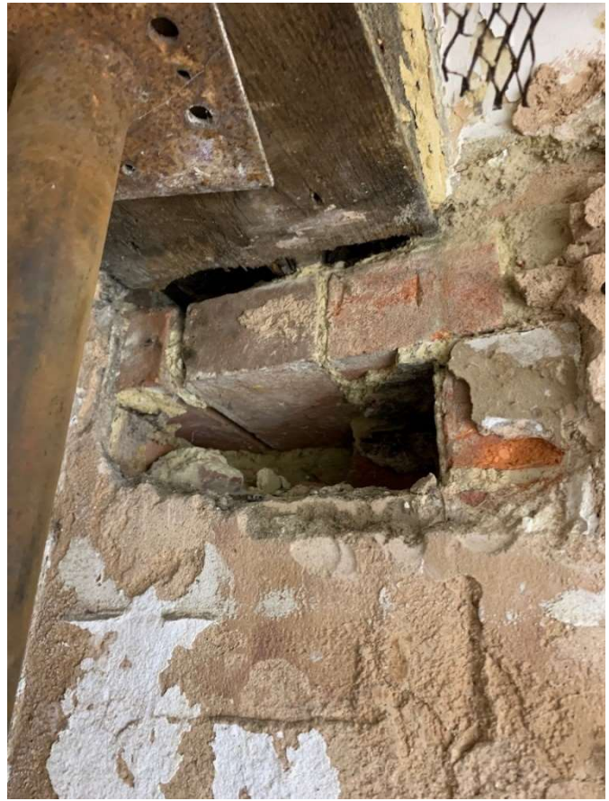
Figure c. Wall supporting RH end of beam with timber bonding brick missing.
