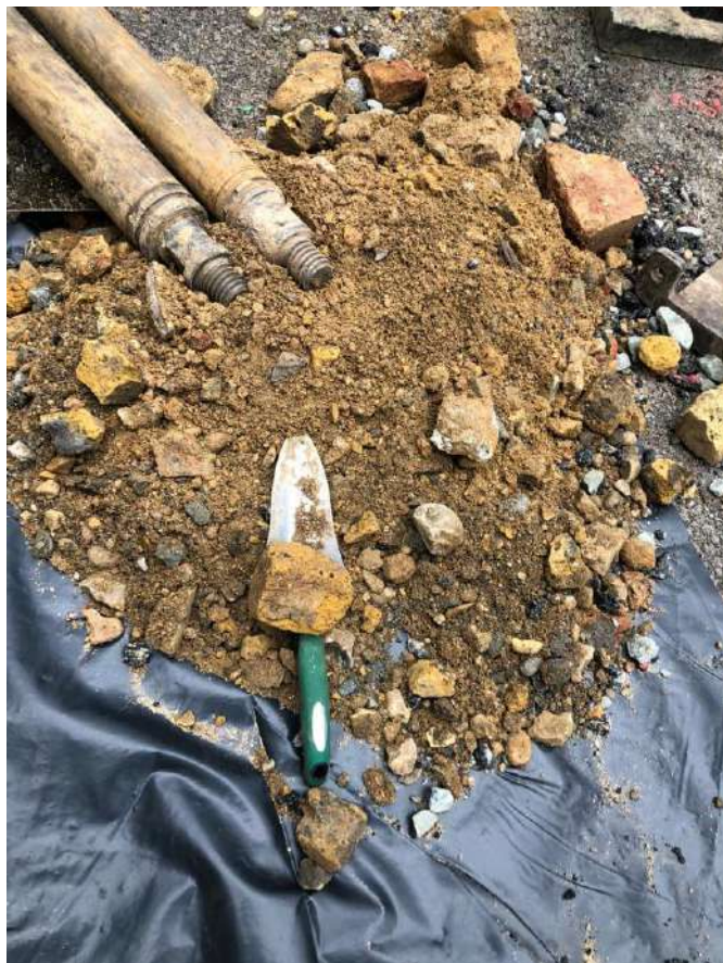
Photos 8 – Showing the soil arisings from the hand dug safety starter pit
