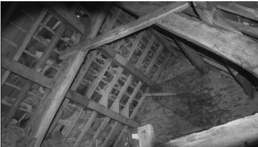
Figure 3b: Screenshot from infra-red camera at darkest point of survey (dawn survey 08/06/2023): interior of barn.
