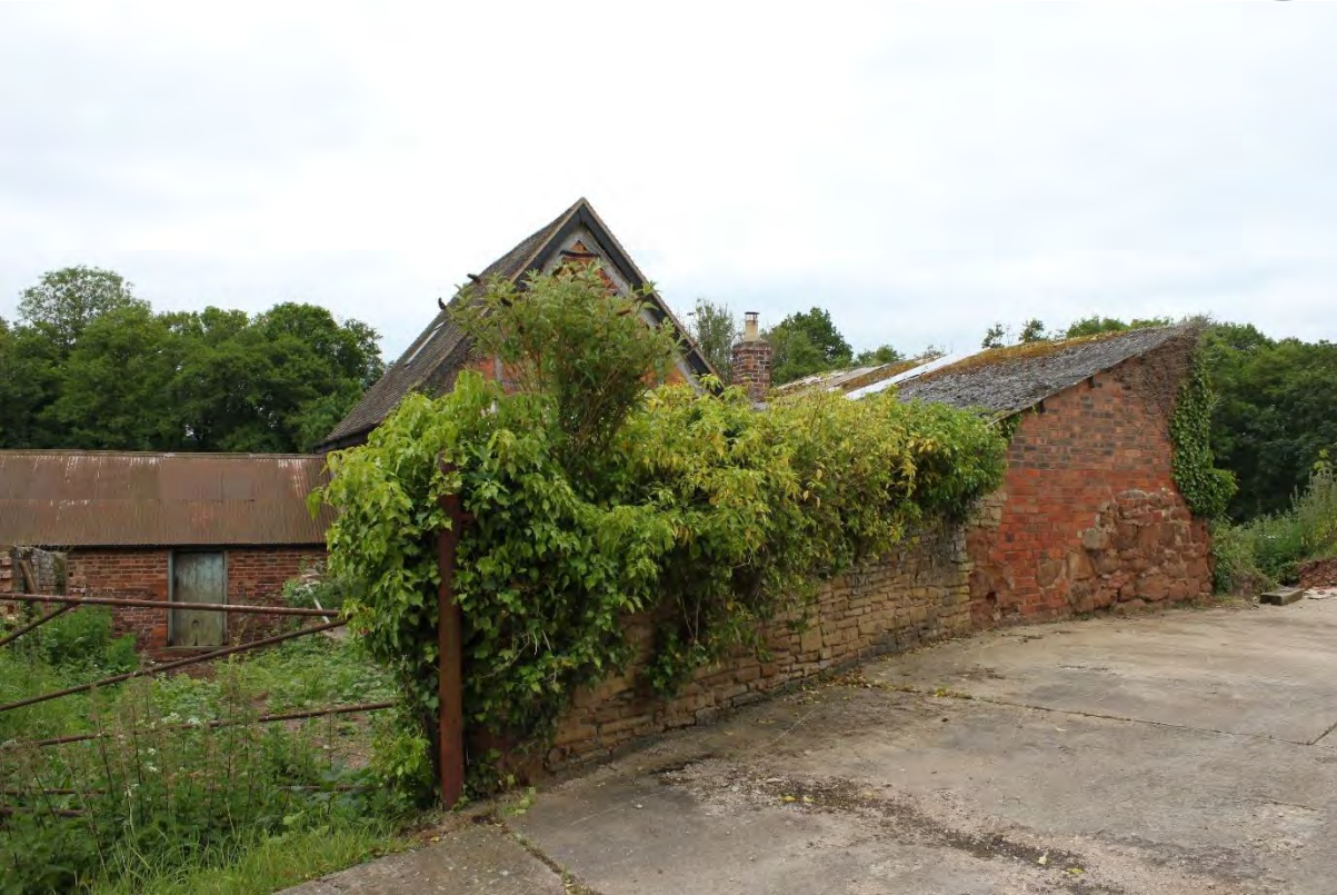
Figure 27: Plate 14 View to the structure understood to include the former Blowing House, looking southwest
