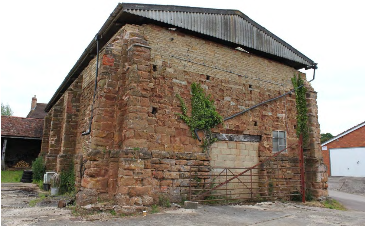
Figure 16: Plate 3 The building, view to the south and west elevations, looking northeast
