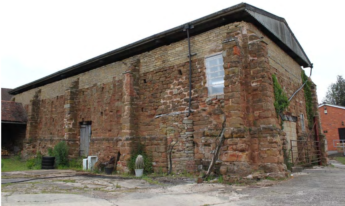
Figure 17: Plate 4 The building, view to the south and west elevations, looking northeast (2)
