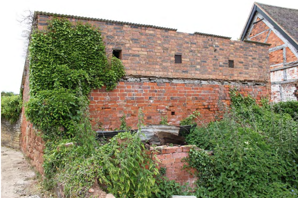
Figure 30: Plate 17 View to the structure understood to include the former Blowing House, looking east
