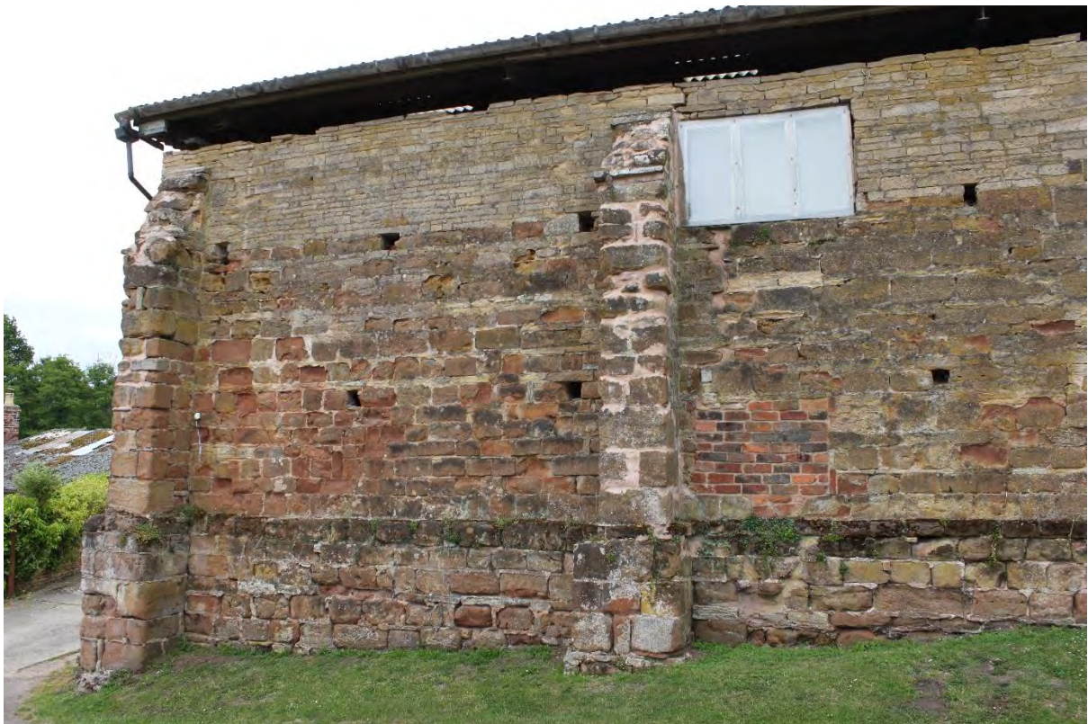
Figure 38: Plate 25 The building, view to the south section of the east elevation, looking southwest
