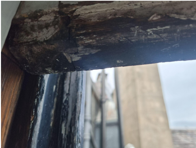
Rotting and failing tenon joint.
