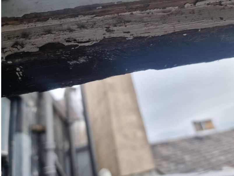
Rotting and water damaged bottom rail.
