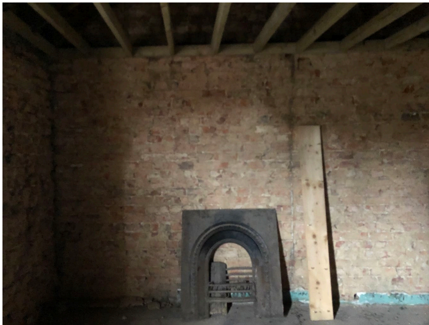
Photo 7: Fire grate in storage
