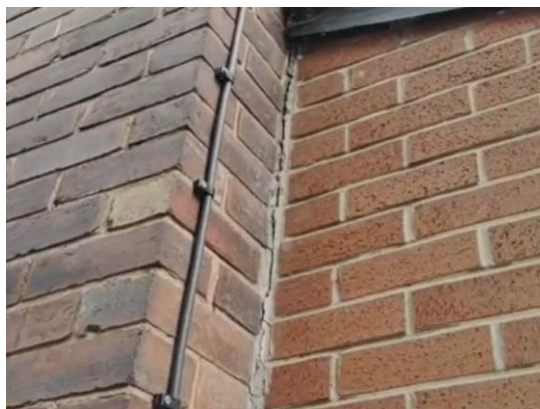
Picture 1: Crack between house and garage
