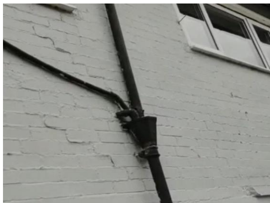
Picture 3: Cracking to rear elevation
