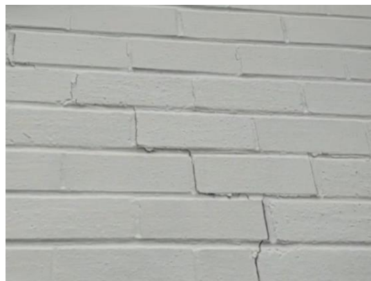
Picture 4: Cracking to rear of garage
