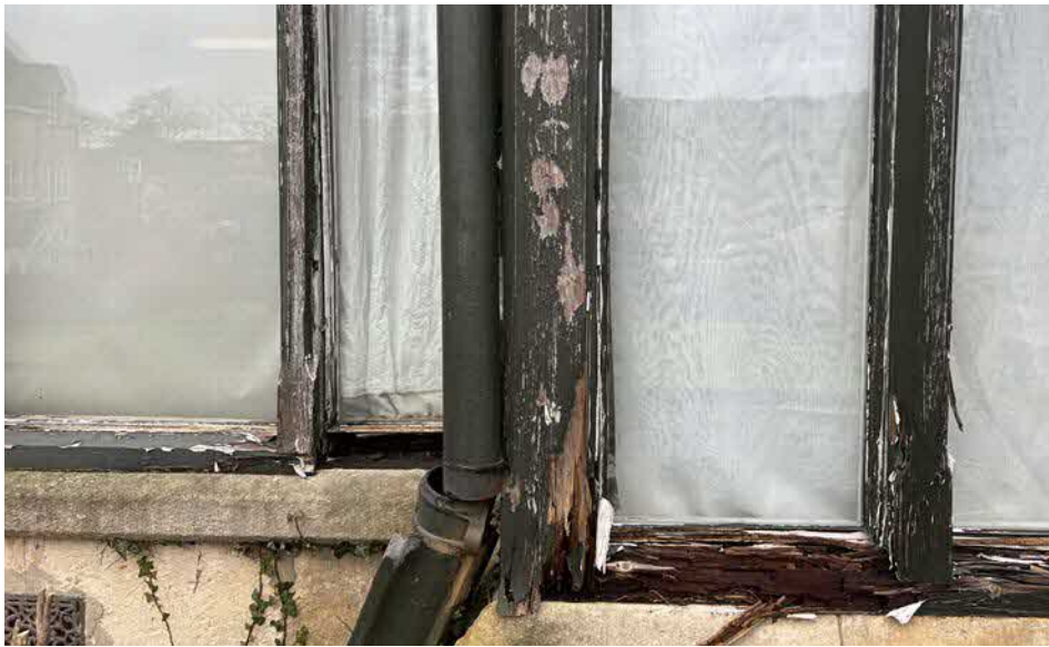
Fig 15. Deteriorating timber structure
