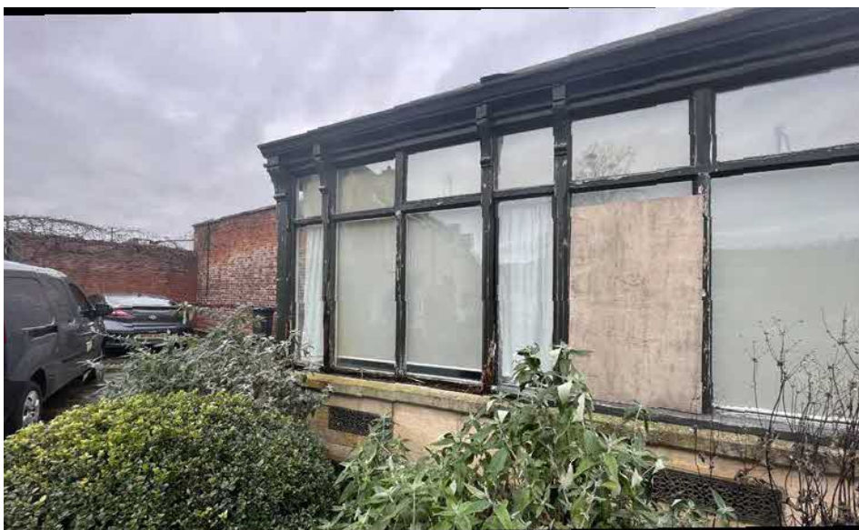
Fig 16. Existing conservatory south elevation with broken glazing
