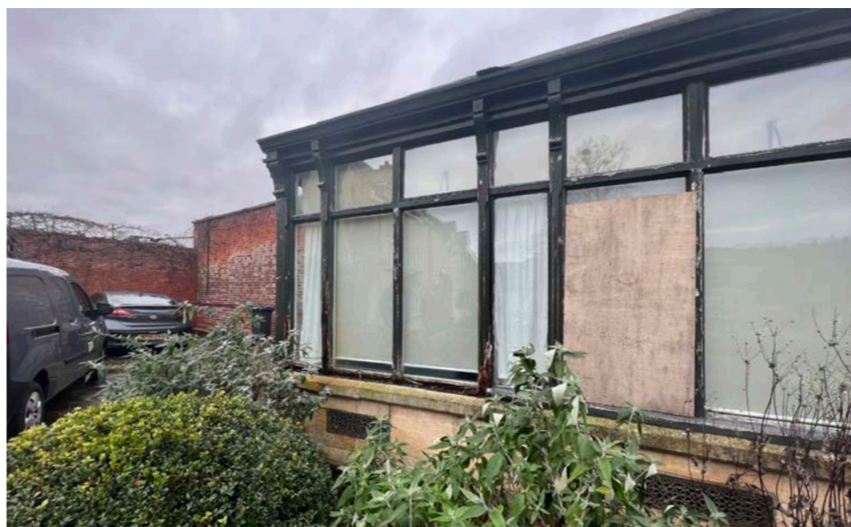
Fig 16. Existing conservatory south elevation with broken glazing
