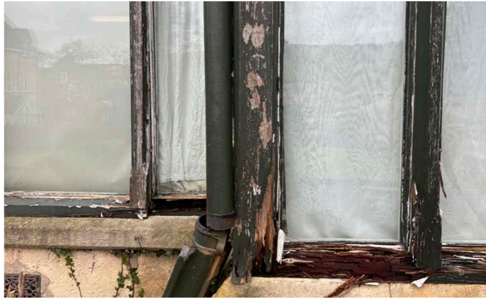
Fig 15. Deteriorating timber structure
