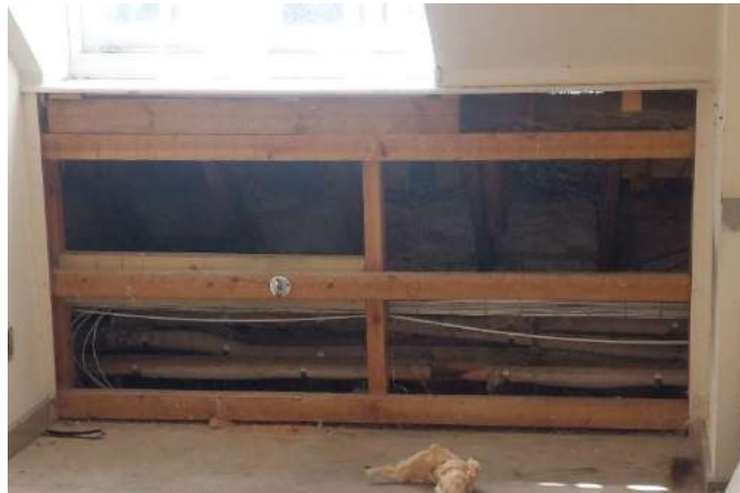
Fig. 17 Roof void visible through missing panelling
