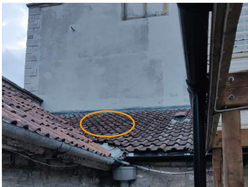
Figure 16 The location of the common pipistrelle day roost access point located below a lifted tile on the western pitch of the roof of the Rear Extension
