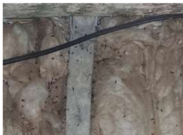
Fig. 60 Bat droppings found in The Barn roof
