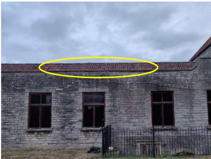
Figure 15 The location of the soprano pipistrelle day roost access point located on the eastern pitch of the Link Building (precise location unknown)
