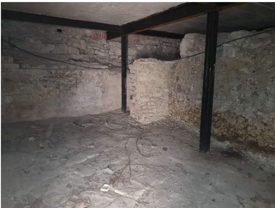
Fig.14 Back Cellar (southern end) indicating wall behind which LHS bat was found (see detail below)
