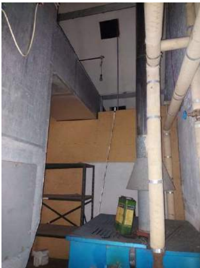
Fig. 40 Boiler room above Barn
