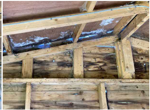
Gap along roof edge (south gable)
