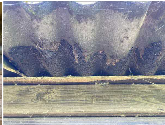
Unsealed roof edge
