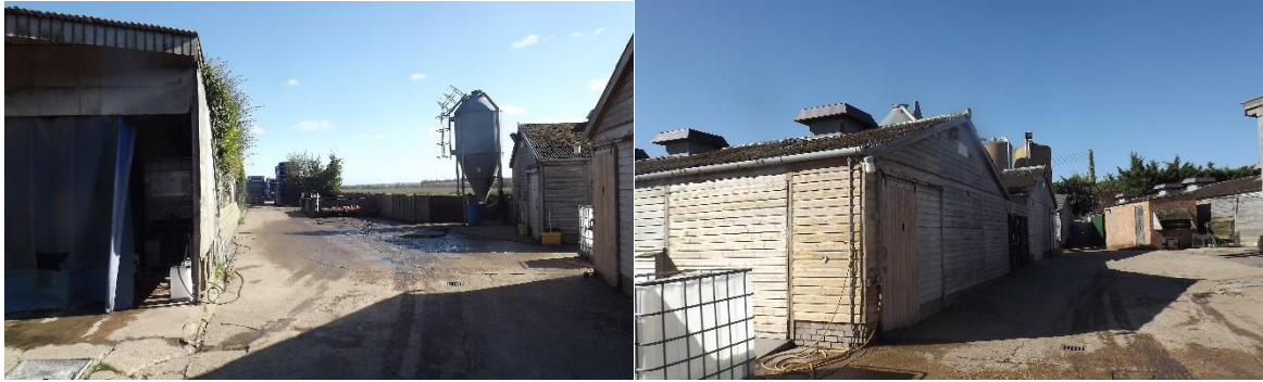
Figure 7 – Feed hopper and concrete aprons (left) and gable ends of sheds B4-B6 (right)
