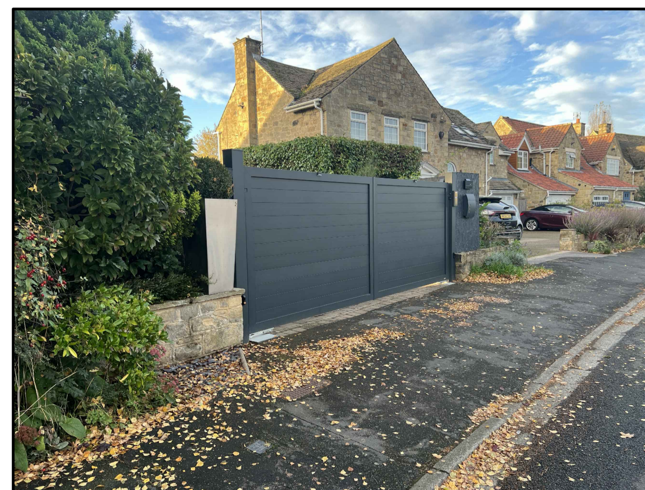
ELEVATION ON INSTALLED GATE
