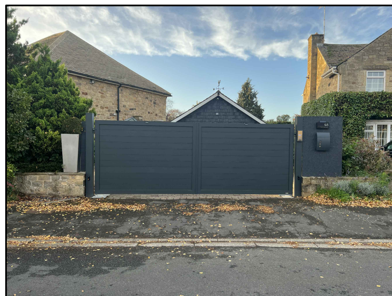
ELEVATION ON INSTALLED GATE
