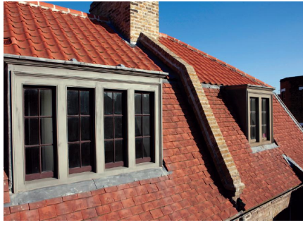
TURNER STREET IN THE SPITALFIELDS CONSERVATION AREA SHOWING TRADITIONAL LEAD DORMERS WITH TRADITIONAL CORNICES
