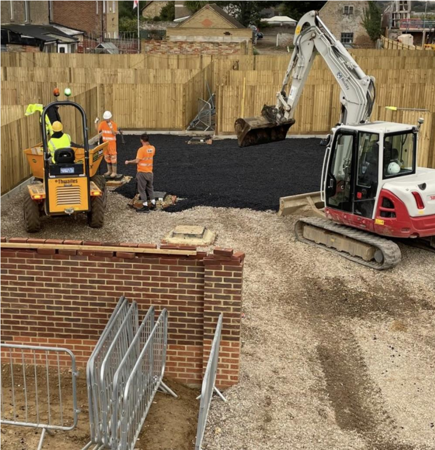
Figure 2 – Installation of the base layer in the courtyard to the rear of Plots 24 & 25.
