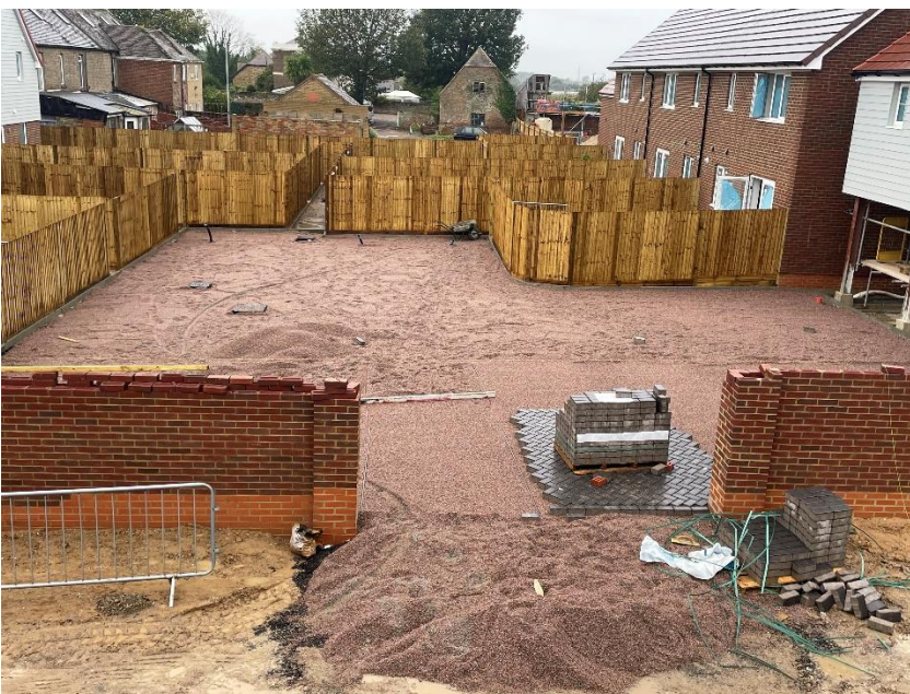
Figure 3 – Installation of the bedding layer and permeable blockwork in the courtyard to the rear of Plots 24 & 25.
