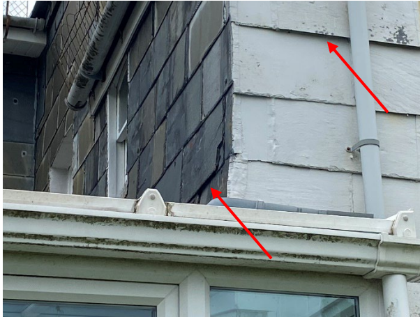
Figure 15. Gaps between slate tiles on the southern elevation of the dwelling.
