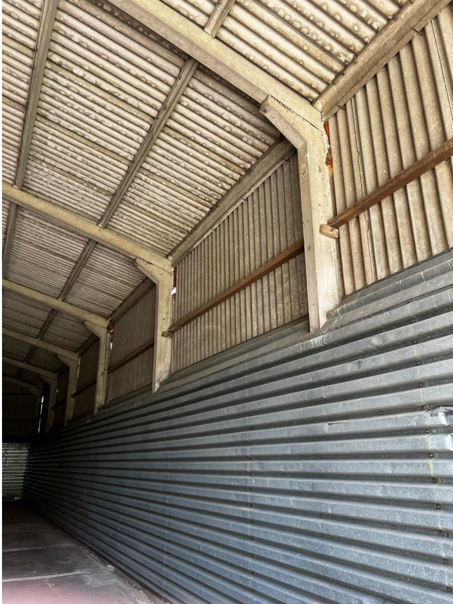
5.15 Portal bolted haunched connection to east elevation, timber cladding rails, steel corrugated sheeting retaining wall at low level
