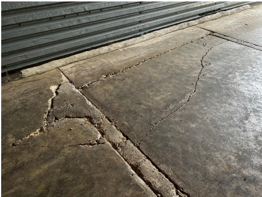
5.19 Cracking to ground bearing slab
