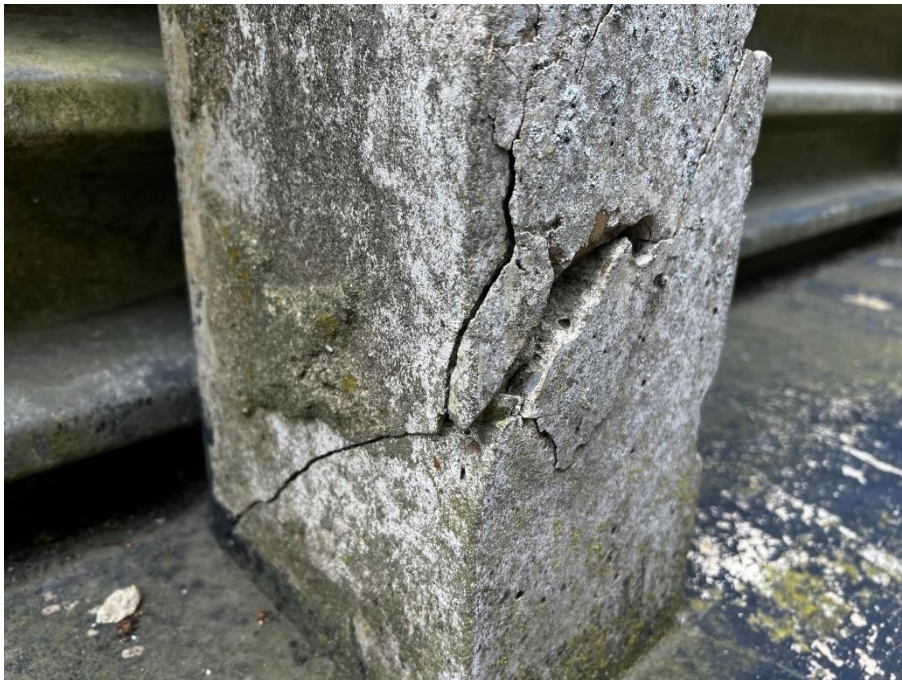
5.21 Cracking to gable column on north elevation at low level
