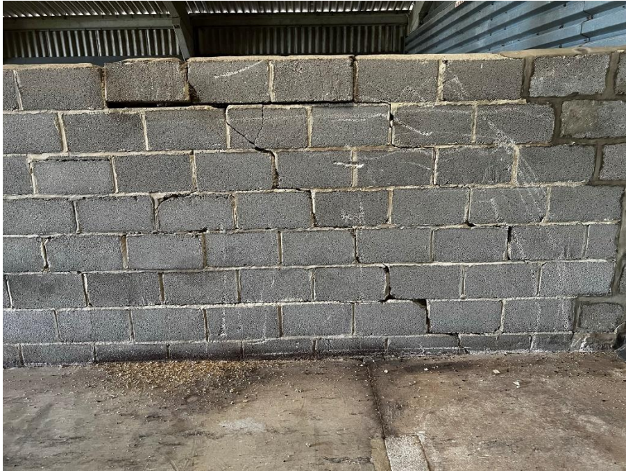
5.20 Movement and cracking to internal blockwork dividing wall
