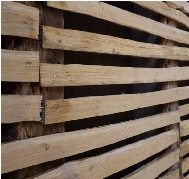
New timber laths if existing ones cannot be retained, spaced to allow key for plaster scratch coat
