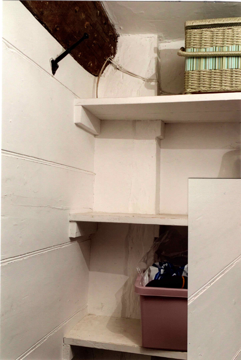
View of the existing ground floor store corner looking towards the ceiling, where the SVP will be located, if situated internally.
