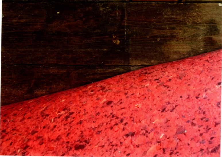
Close -up view of the floor boards in the bedroom where the basin waste went through the floor.
