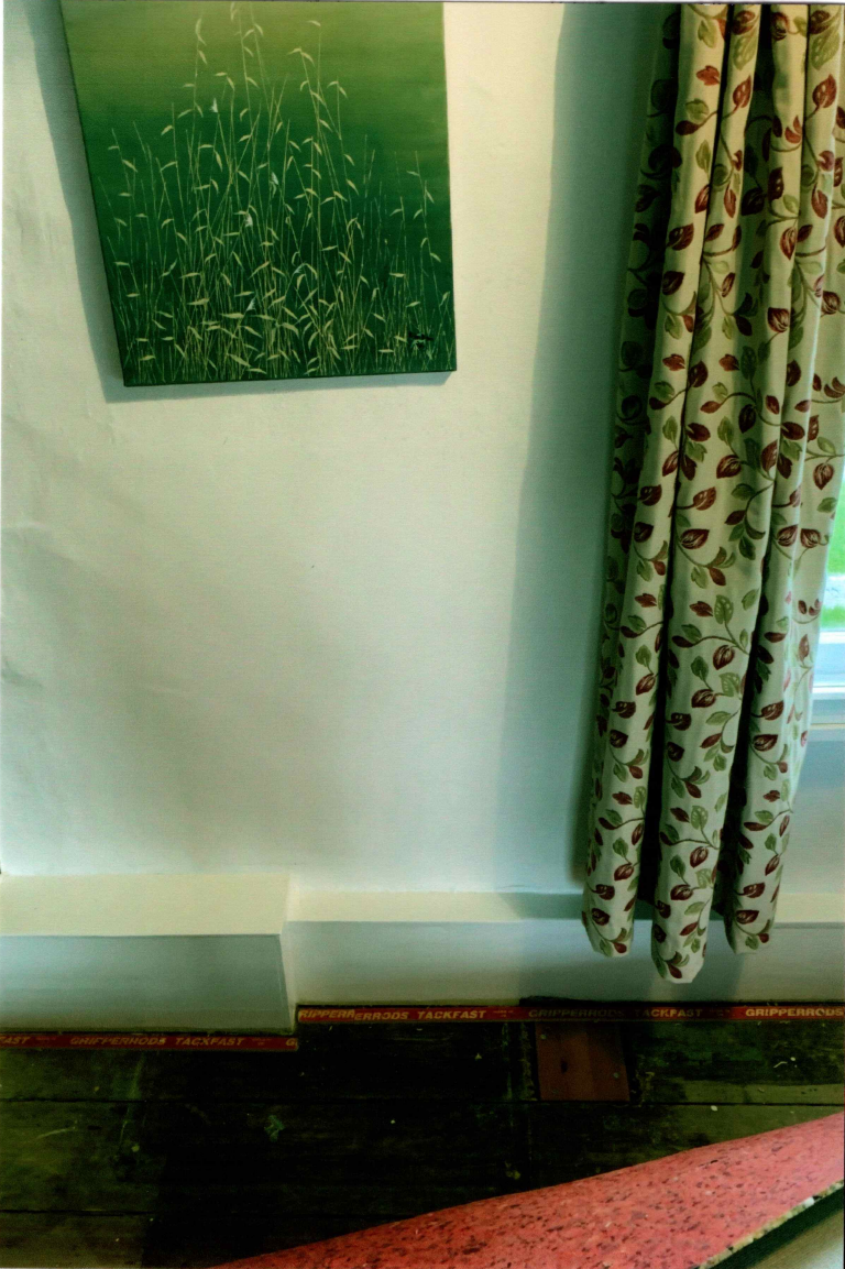
View of the bedroom external wall where a basin was located previously. The repair to the floor boards shows where the waste pipe went through the floor.
