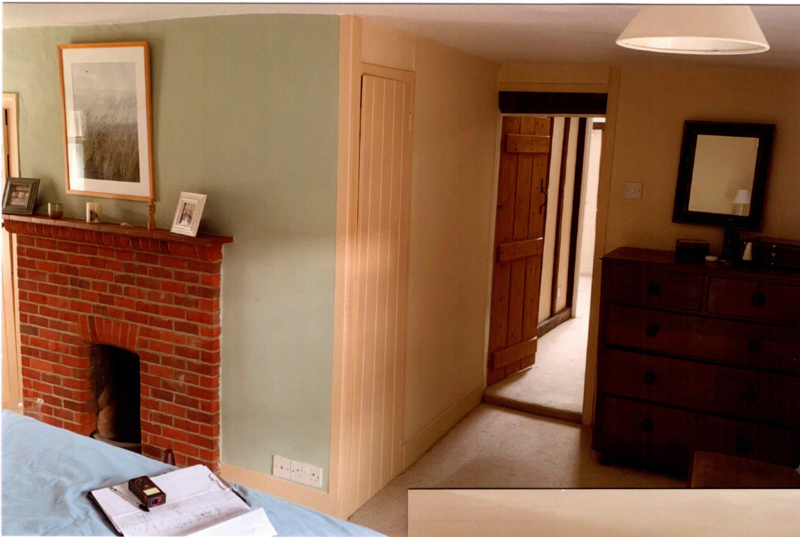
View of the cupboard to be removed to expose the chimney at first floor level in bedroom 2.
